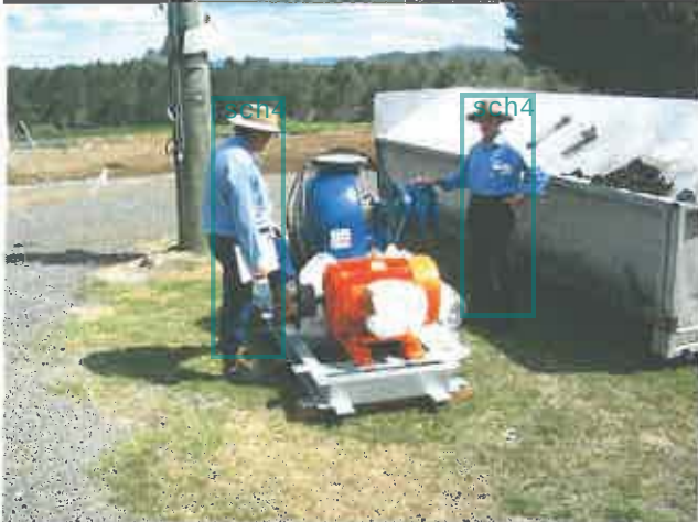
Photo. 1: New VITOX pump unit and 75HP electric motor awaiting installation at the Aerobic Pond as part of the upgrade of the oxygen delivery system to the pond. Enclosed "Scutch" transport skip in background.
