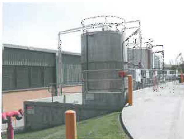
Fig 1: Bulk corrosive materials storage.
