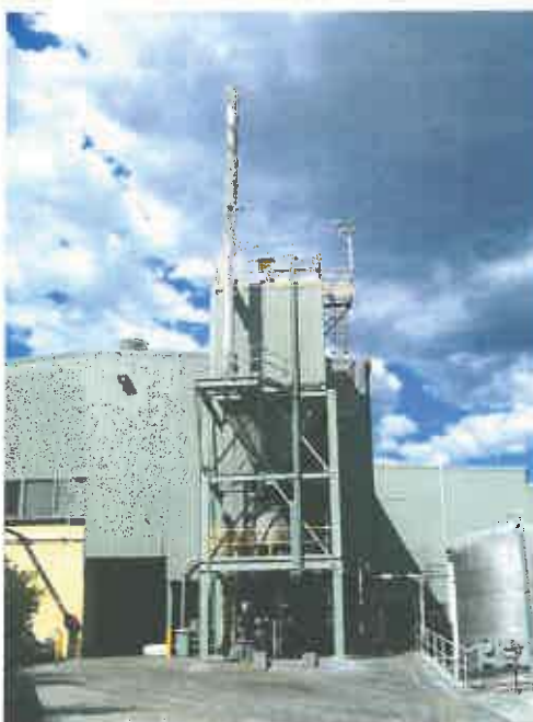
Photo. 37: Finafire coal-fired Boiler with the new Bag House unit located on the tower, to the rear and right of the Stack.
