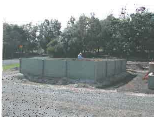
Fig 11: Wastewater treatment plant biofilter.
