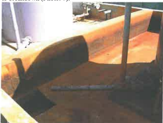
Photo. 7: View of the internal bund wall showing the early breakdown of the epoxy coating. While the repair/upgrade job has been scheduled for resealing work, to date, no leakage to the external soil environment has been apparent.
