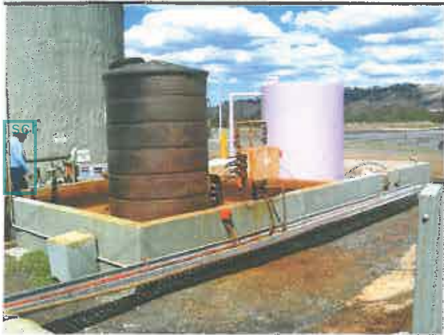
Photo. 6: Chemical storage tank bund being inspected during the audit. While the external bund condition appeared sound, the internal epoxy wall cover had begun to breakdown (Photo. 7).
