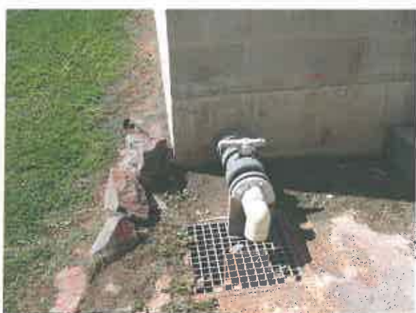
Fig 3: Bund drainage / shutoff valve. Permits the release of uncontaminated stormwater.
