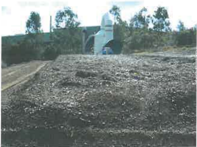
Photo. 35: Bed of the large Biofilter unit treating gelatine plant processing air, which was rehabilitated early in 2004. Optimum internal humidity conditions are maintained using top laid "soaker" hoses. Further maintenance work is to be undertaken on the fan housing and surrounding drainage works, during the upcoming 2004/2005 shutdown.
