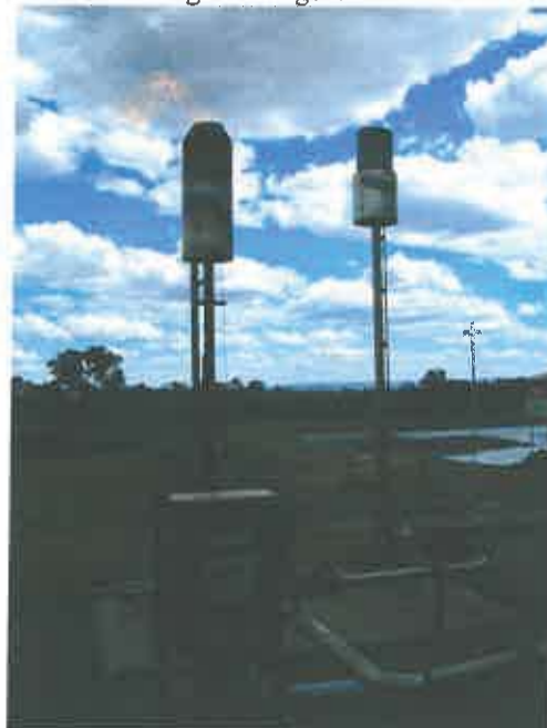
Photo. 15: Methane gas flare plant burning off materials produced by the Hybractor Primary Digester unit. This material has been considered as a potential energy resource for an on-site co-generation project, which application remains "on hold" at this time.
