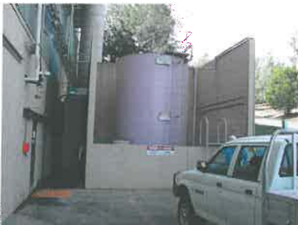
Fig 8: Bulk sulphuric acid storage and bunded area.
