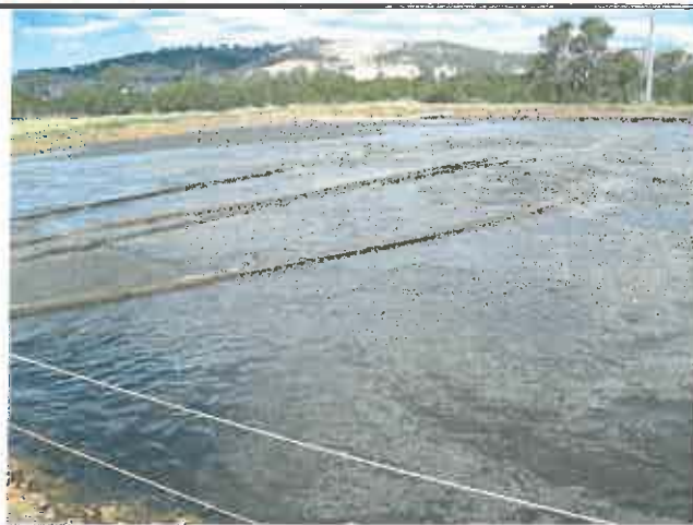
Photo. 9: Aerobic effluent treatment pond showing air entrainment supply hose lines from the air Blower Unit aerating the pond contents. During the formal site audit and inspection, the Aerobic Pond was noted to be an "ideal" chocolate brown colour (C Smeal).
