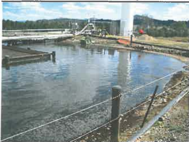
Photo. 11: View of the "old" VITOX oxygen delivery plant (top, centre), on the bank of the Aerobic Pond, due for replacement with the "new" unit shown in Photograph 1.
