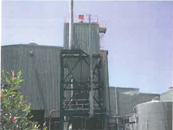
Photo 2 – New baghouse installed on the Finafire coal-fired Boiler.
