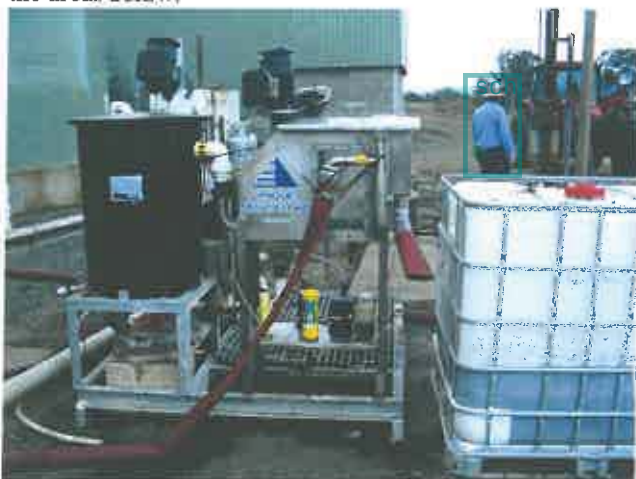
Photo. 13: Experimental fat removal unit using induced air entrainment principles to physically remove tallow from the effluent stream.
