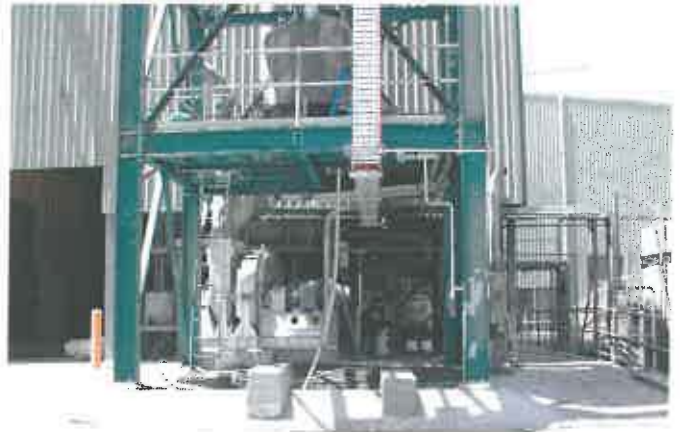
Photo 4 – Connection chamber for the Finafire coal-fired Boiler to the new baghouse installation.
