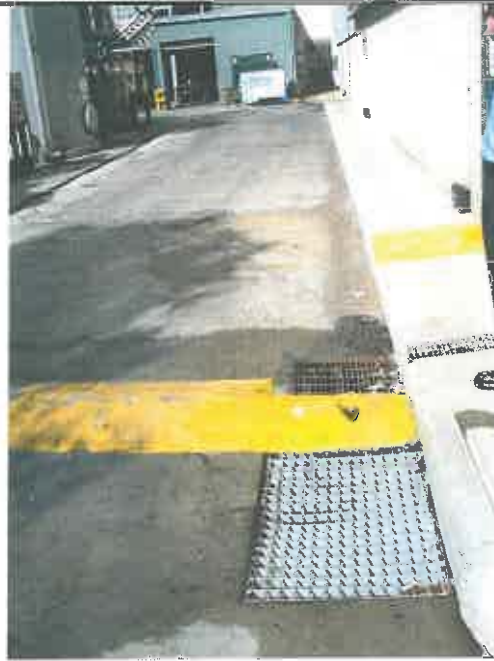
Photo. 40: The yellow roll-over bund separates the "dirty" area gully trap (upper) servicing access to the "scutch" load-out tank and draining to the effluent treatment system from the "clean" access roadway area stormwater gully trap (lower) draining to the plant surrounds "catch dam" (Photo. 29). A sump pump services the "dirty" area gully trap.
