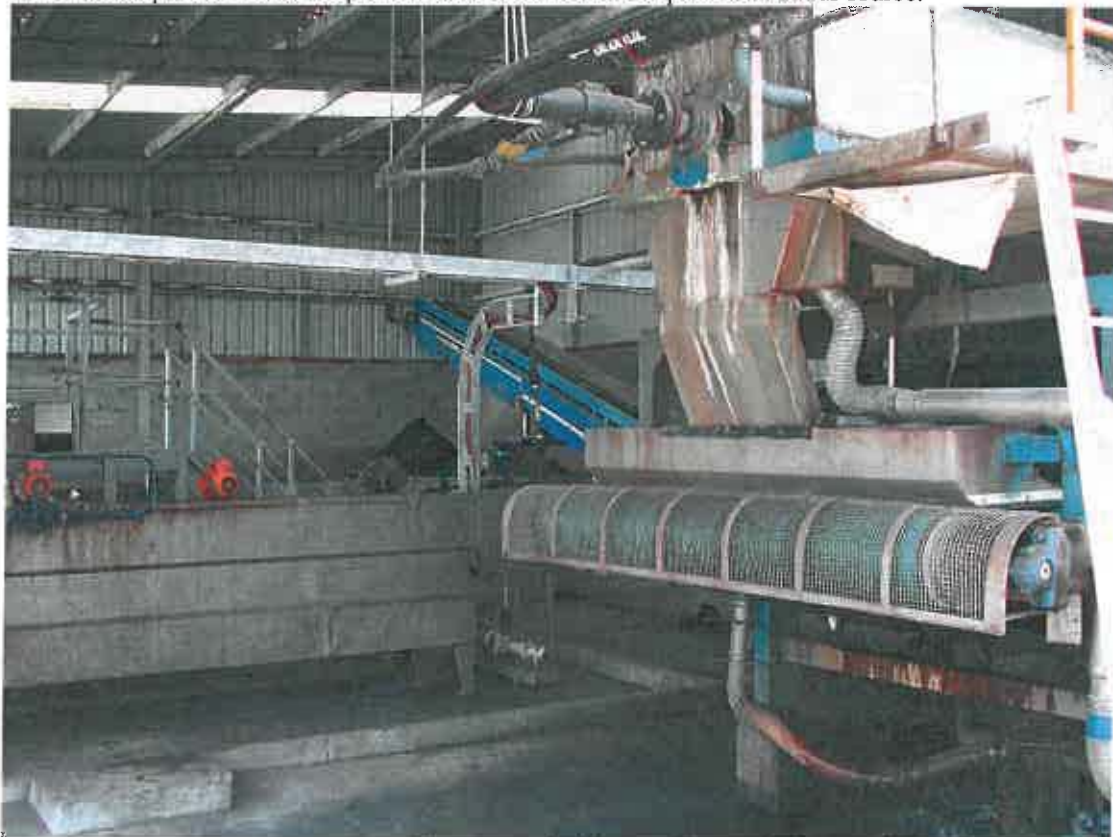
Figure 4: Belt press facility. There was a significant odour emitted sporadically from this activity.
