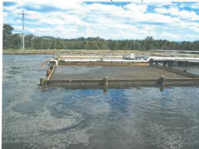
Photo. 10: Another view of the Aerobic effluent treatment pond showing the VITOX oxygen injection/sparge line. The Company has secured three (3) floating Dissolved Oxygen (DO) Meters at the end of the line tray towards the centre of the pond (centre, left) to provide continuous readout/backup of pond DO results. Three (3) units are employed using the theory that should one (1) unit fail a "backed-up" unit remains, allowing monitoring coverage at all times, of the critical oxygen levels being achieved in the pond. The Aerobic Pond was stated to be in a "healthy" condition, according to daily monitoring data generated by the Company. Continuous, accurate DO results ensure critical pond aerobic conditions are maintained, while minimising wastage/costs associated with operation of the VITOX system.
