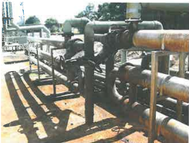
Photo. 12: Recently upgraded heat exchanger units showing the absence of any leaked effluent material onto the areas below.
