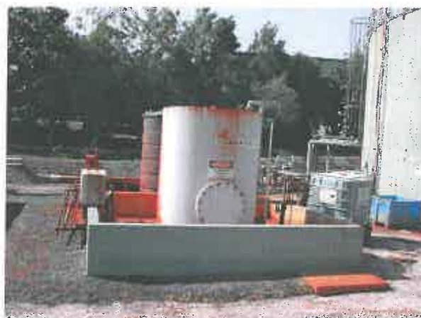
Fig 10: Bunded sodium hydroxide storage for the wastewater treatment plant.
