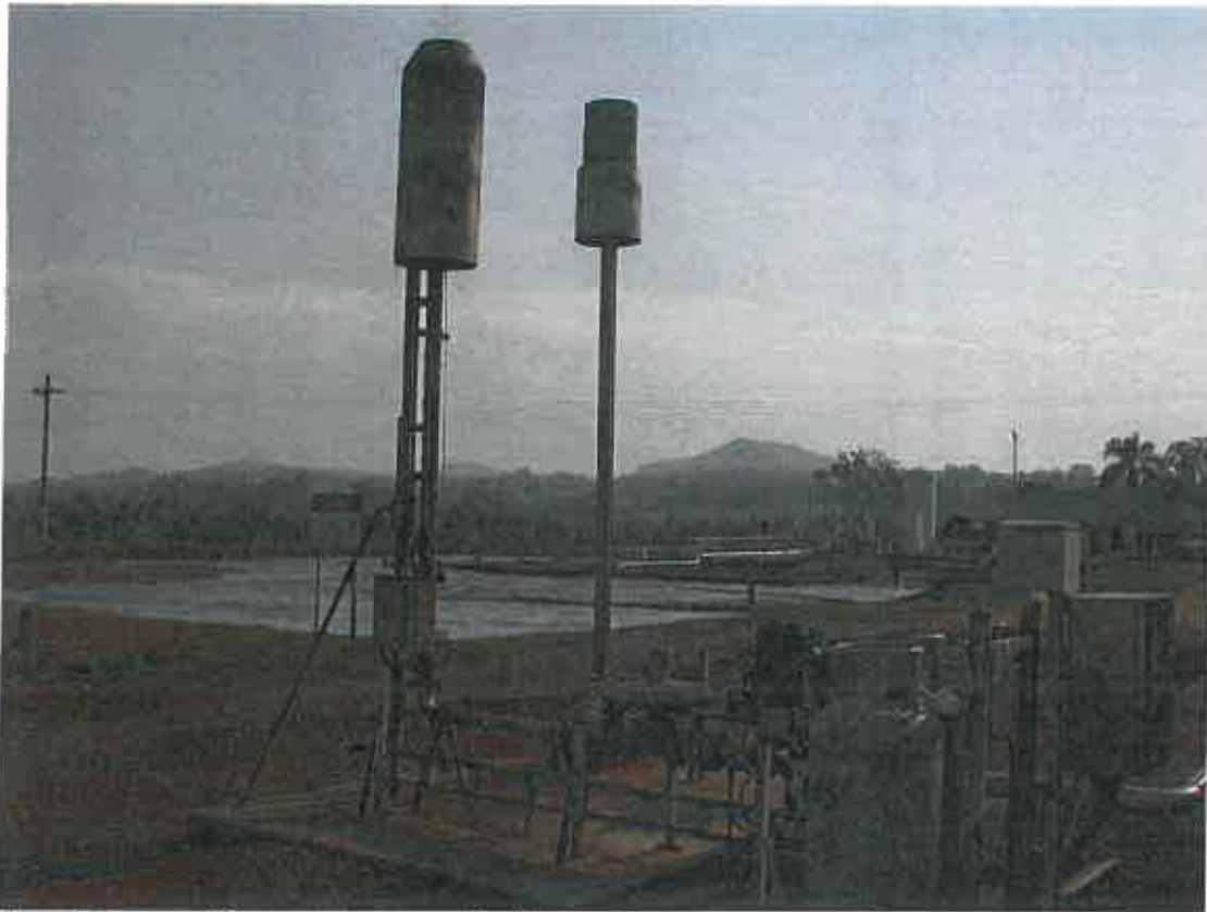
Figure 7: Wastewater treatment facility.
