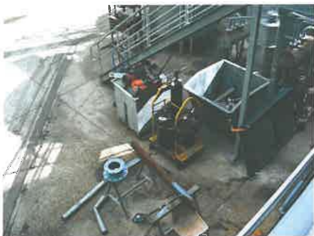
Photo. 39: Boiler surrounds general work area. Boiler water treatment chemicals are held on banded pallets on the floor deck of the tower, from which this photograph was taken (Photo. 37).
