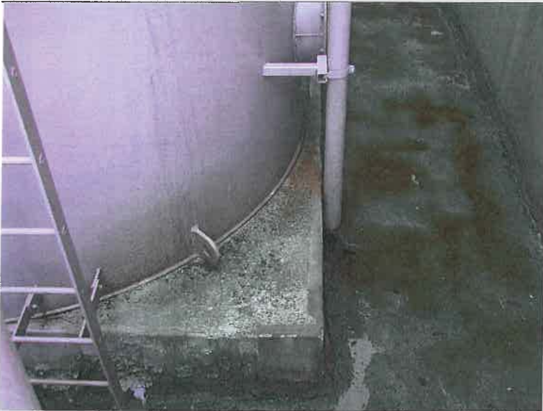
Figure 5: Leaking acid has caused some erosion of the concrete bunding material resulting in the destruction of the steel reinforcing material within the concrete. Davis Gelatine is currently investigating this issue.
