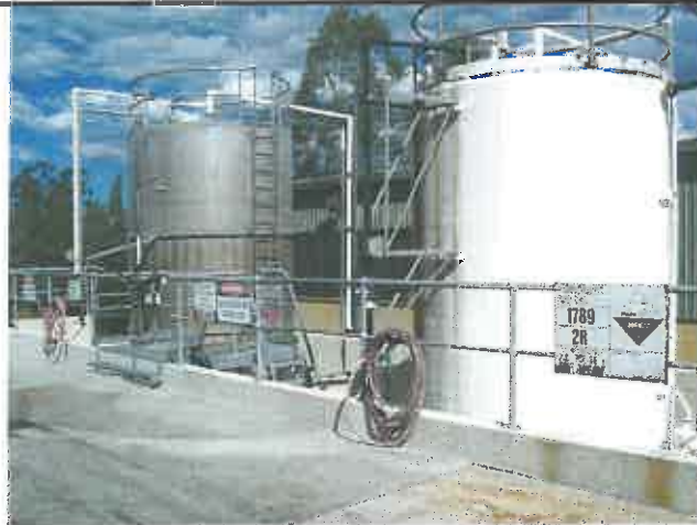
Photo. 36: Effectively bunded bulk chemical and ammonia storage tanks at the rear of the gelatine extraction/processing plant.
