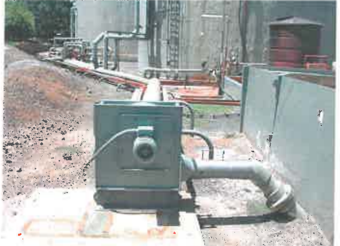
Photo 5 – New, sealed, foul air extraction fan from the Hybractor effluent treatment system to the small Biofilter (odour / control elimination).
