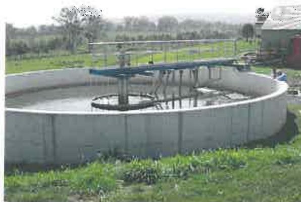
Fig 16: Wastewater Clarifier tank.
