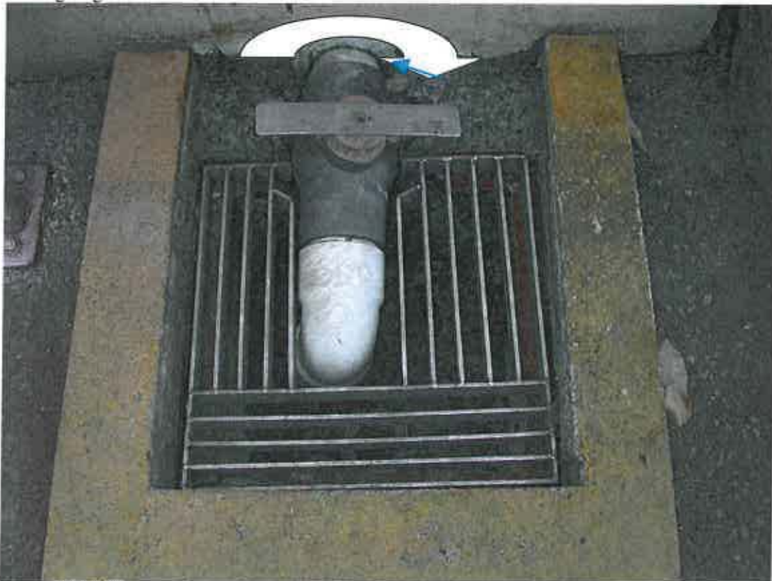
Figure 6: Drain for Sulphuric acid bund. The seal (marked) has deteriorated and it is possible to move the drain around in the direction shown.
