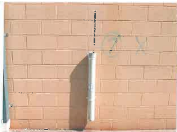
Fig 7: A number of these kits are located around the site near stormwater drains. They contain a foam mat that is placed over the drain to prevent contaminated water entering the stormwater drain.
