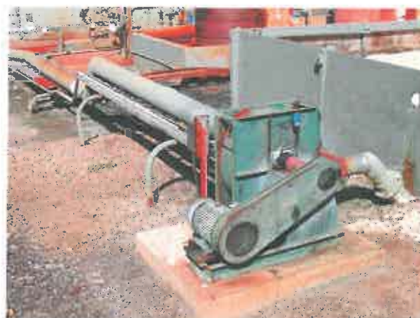
Fig 12: Biofilter foul air pump.
