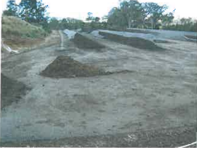
Photo. 17: View of covered composting windrows set out on the asphalt-sealed compost mixing pad/area.
