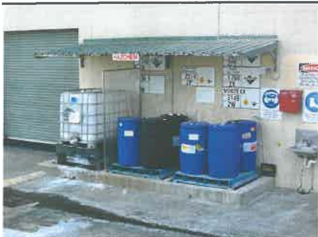
Photo. 34: Roofed and bunded chemical drum storage area on the northern external wall of the gelatine extraction/processing plant. The gully trap in the left, bottom corner of the photograph drains to the effluent treatment system.
