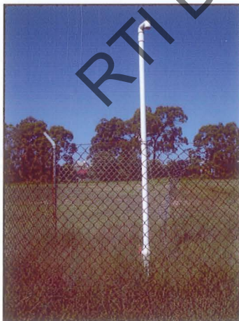
Photo 5: General View of existing gas vent 17/04/09
