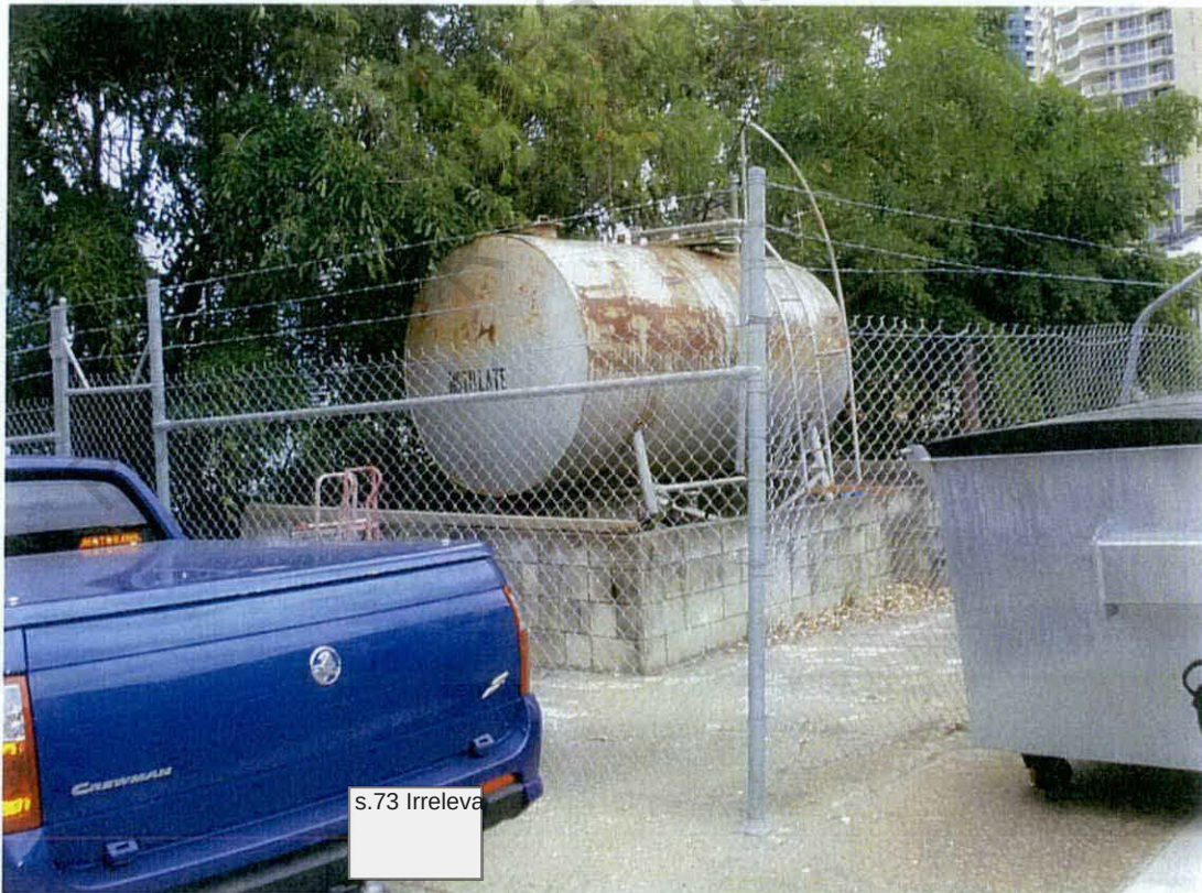
View of disused diesel AST (Lot 3).
