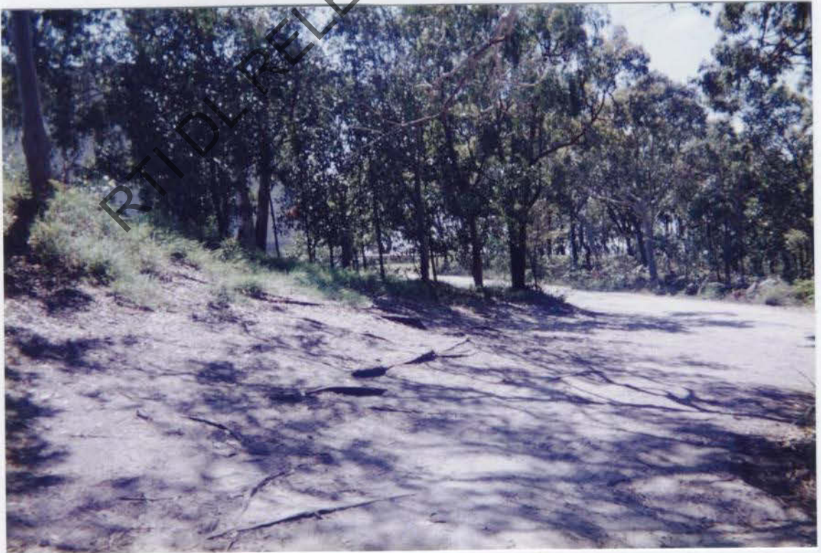
Carlo Sand Blow: The car park is unsealed and lack of relevant drainage is resulting in erosion. Planning for redevelopment of the car park has commenced to provide defined car parking a bitumen surface, fencing and relevant drainage to minimise erosion.
