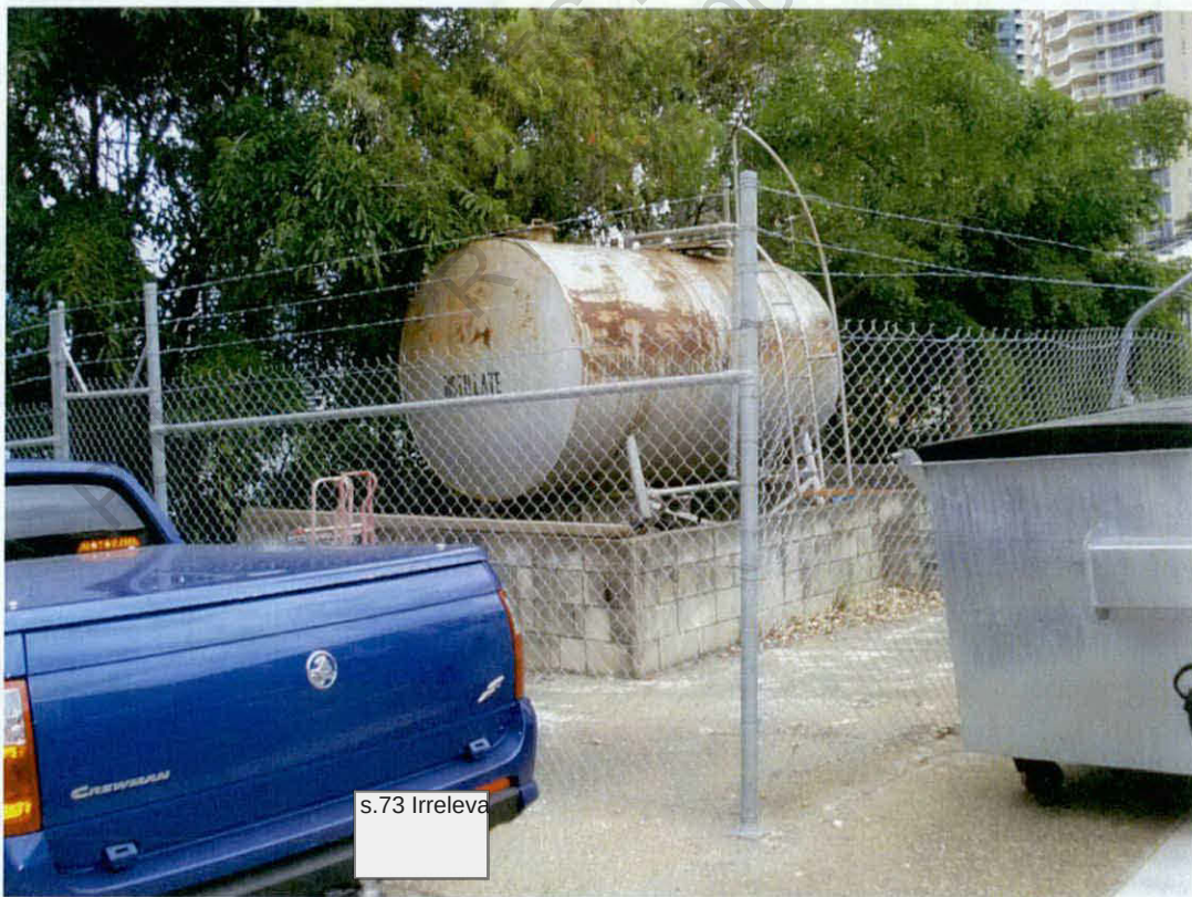
View of disused diesel AST (Lot 3).
