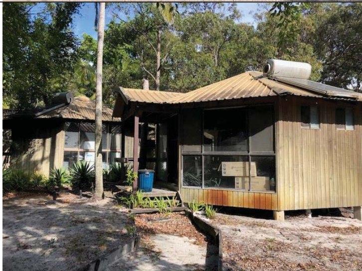
Image 5: Image showing a hut in poor condition, being used for storage purposes.
