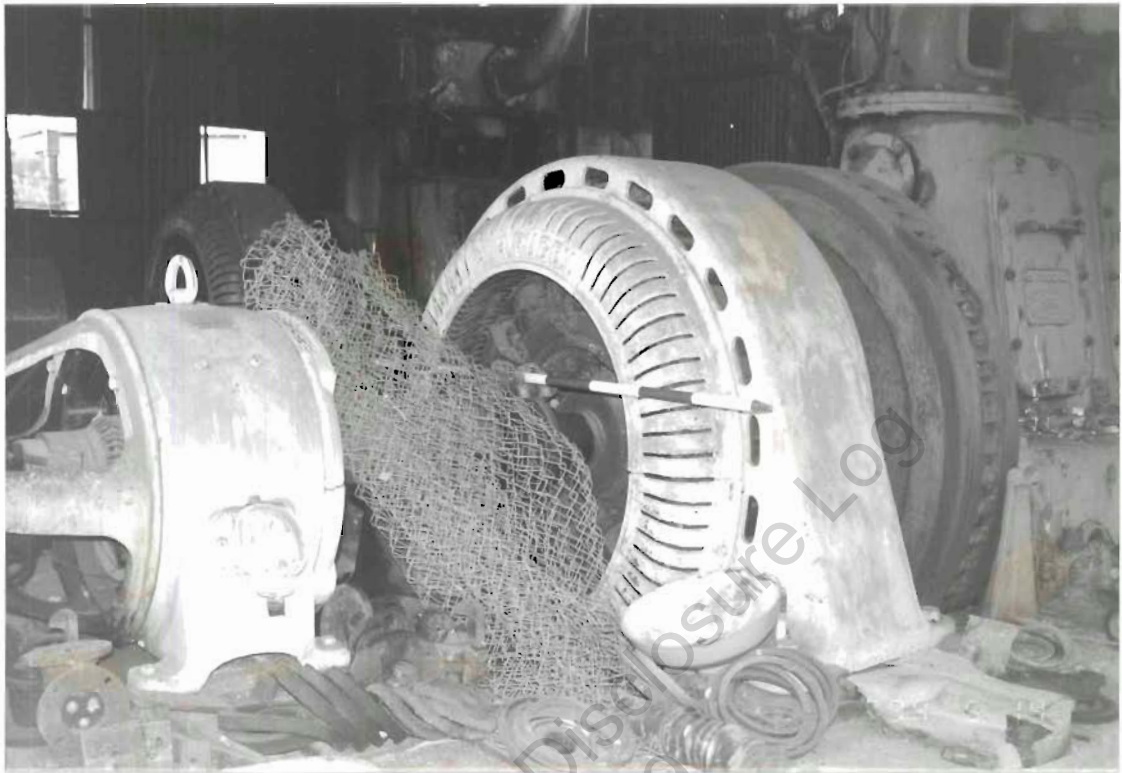
Power house showing a BTH Rugby generator coupled to a Belliss & Morcom engine (on right). Looking W.
