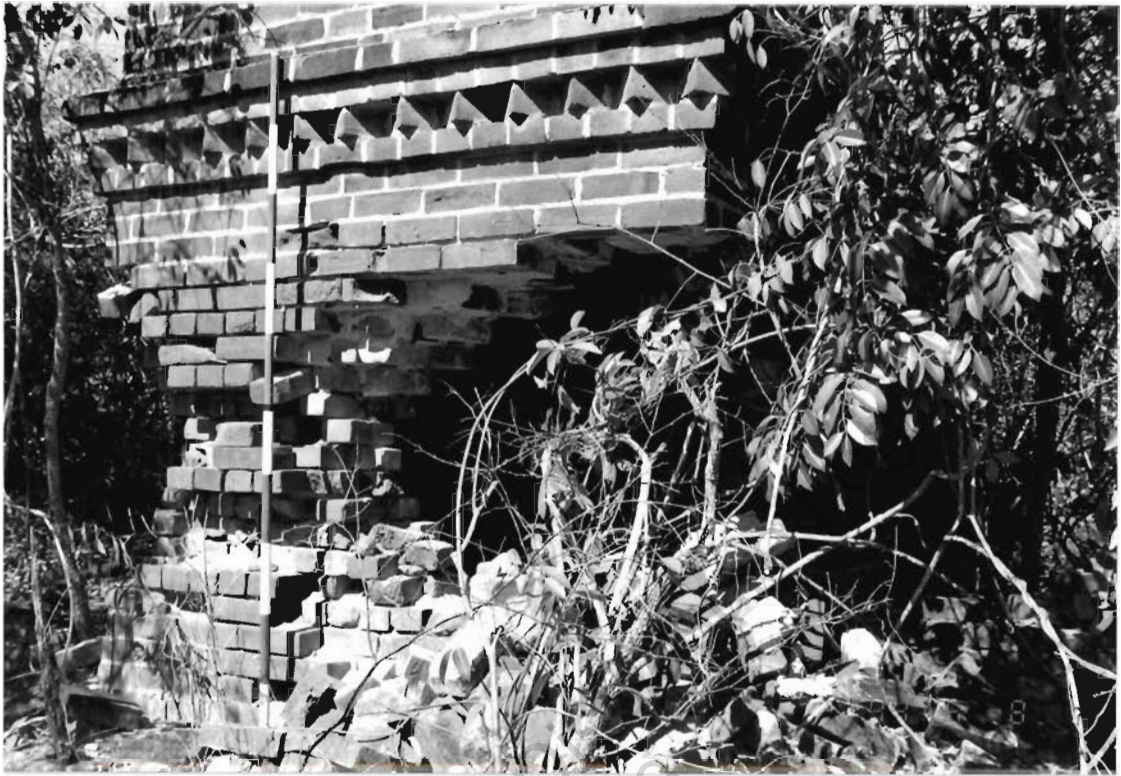
Damaged base of brick chimney, looking SE.
