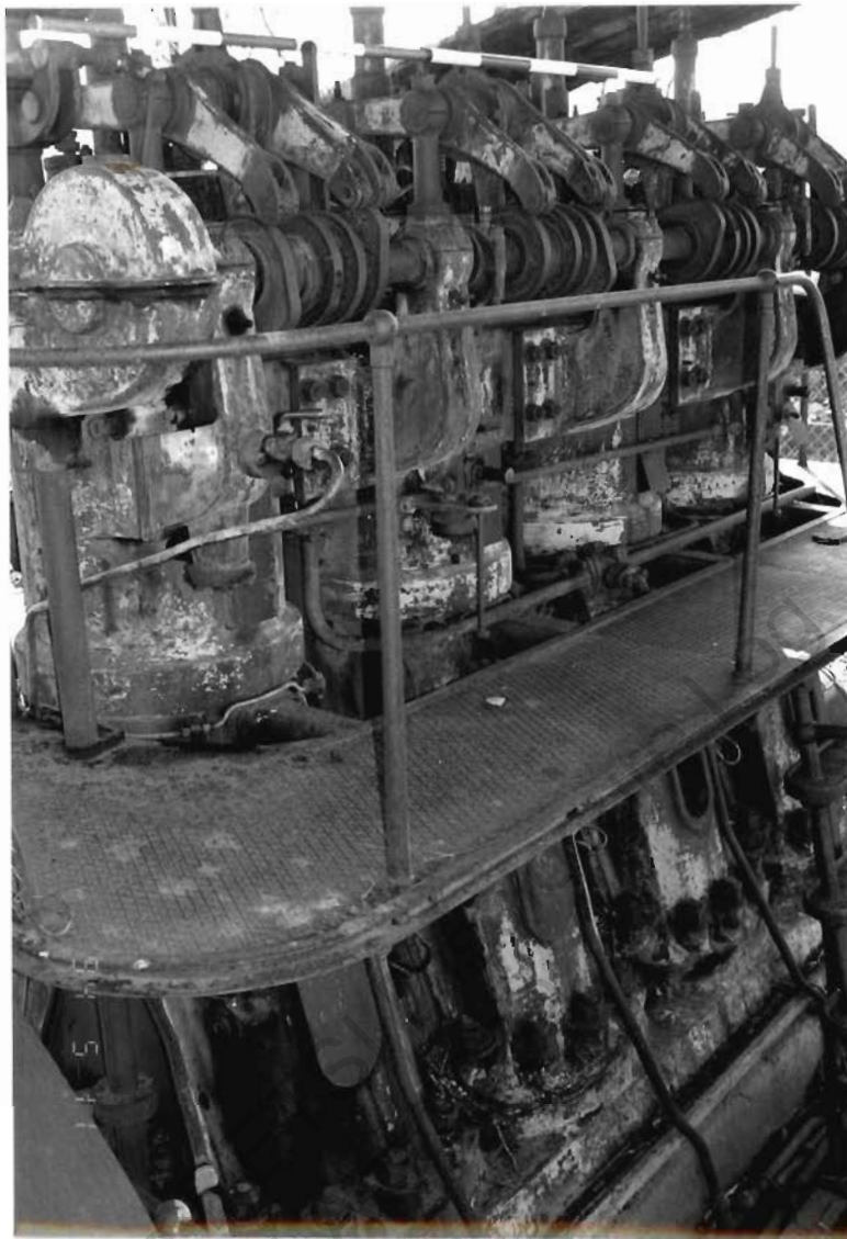
Diesel engine top section, looking NE.
