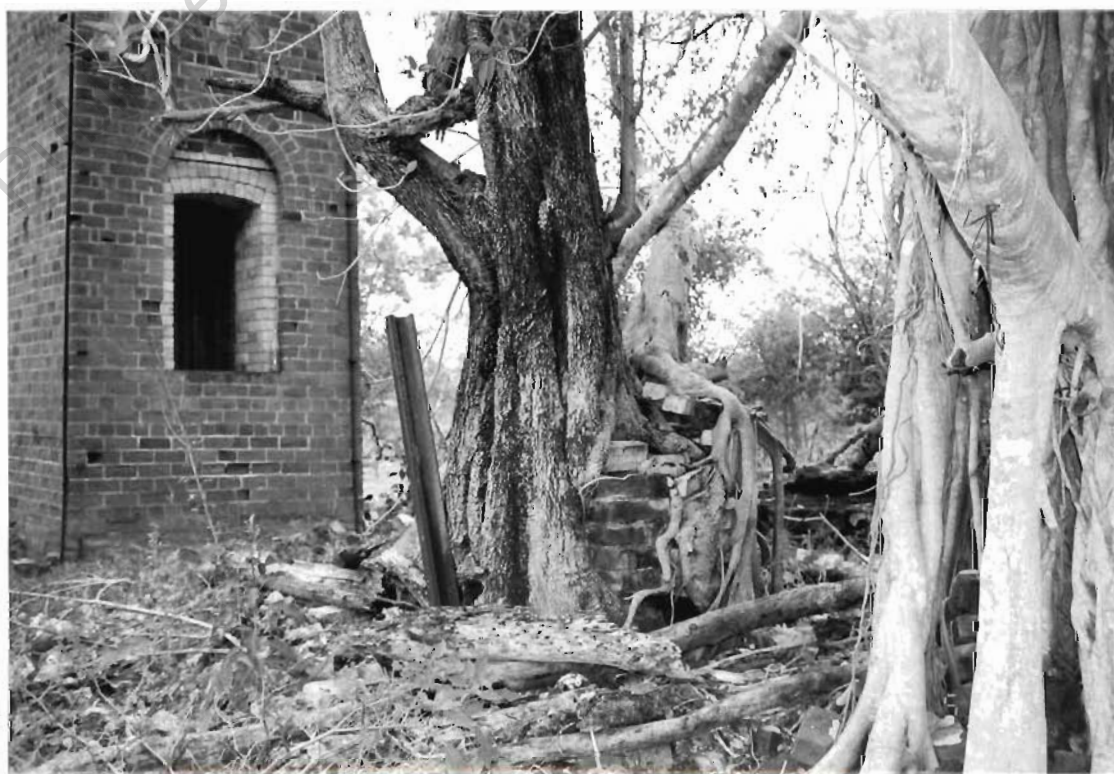
Fig tree growing through the reverberatory furnace flue (centre), with the chimney on the right. Looking W.
