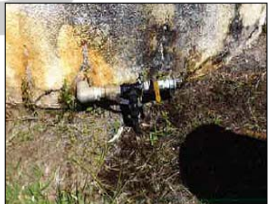
Figure 7. Concrete water tank tap, sample was collected.
