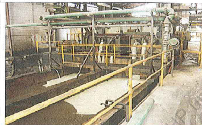
Photo: 1020654 – Collection area for runoff from the production area – oil and trade waste end up here from QE3.
