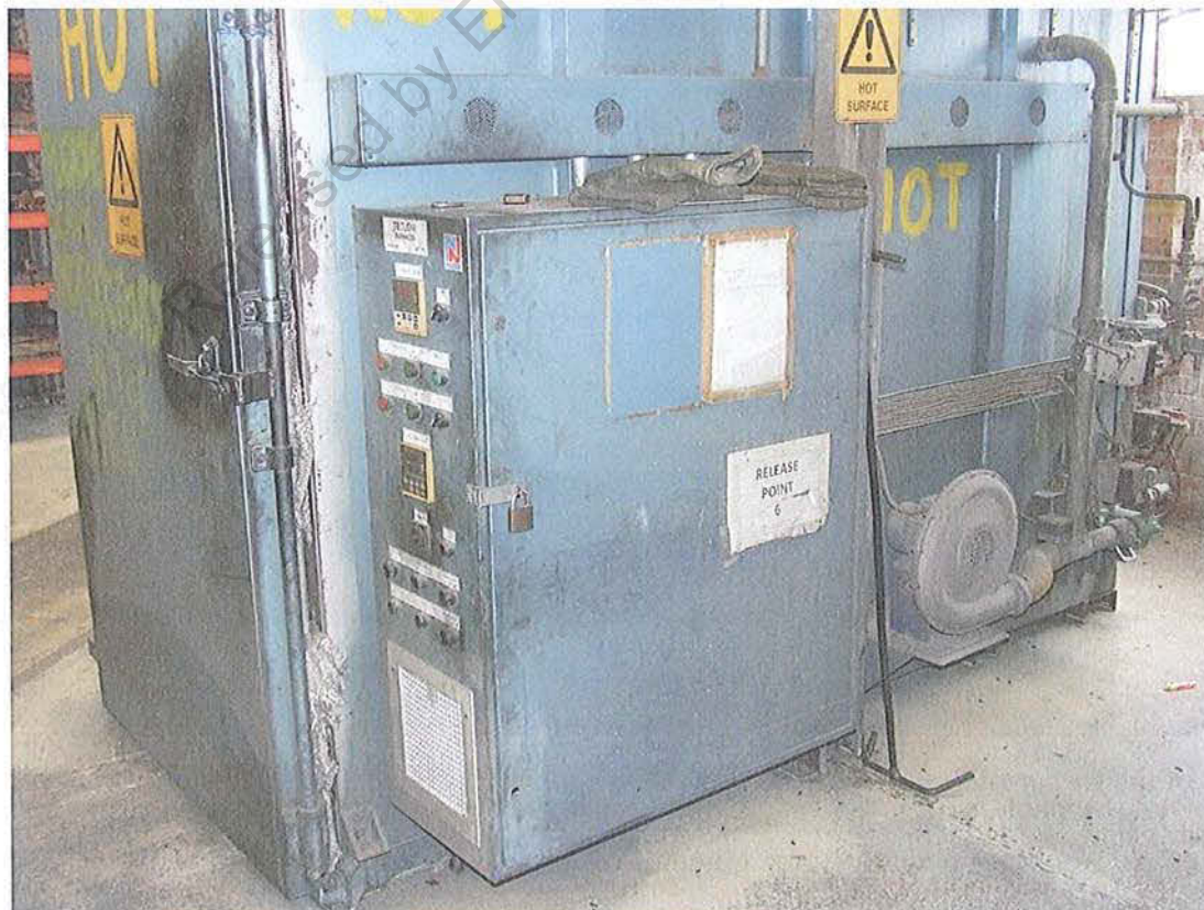
View of the gas-fired delivery cleaning oven.
