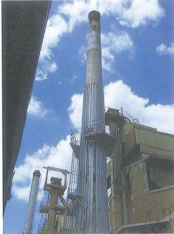
View of Release Point 1 – the QG1 furnace stack.
