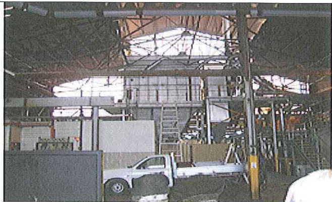
Photo: IMG2803 - Baghouse
