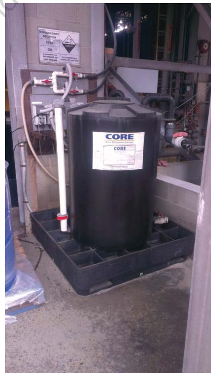
Photo 12 – Bunded sodium hypochlorite water treatment system.
