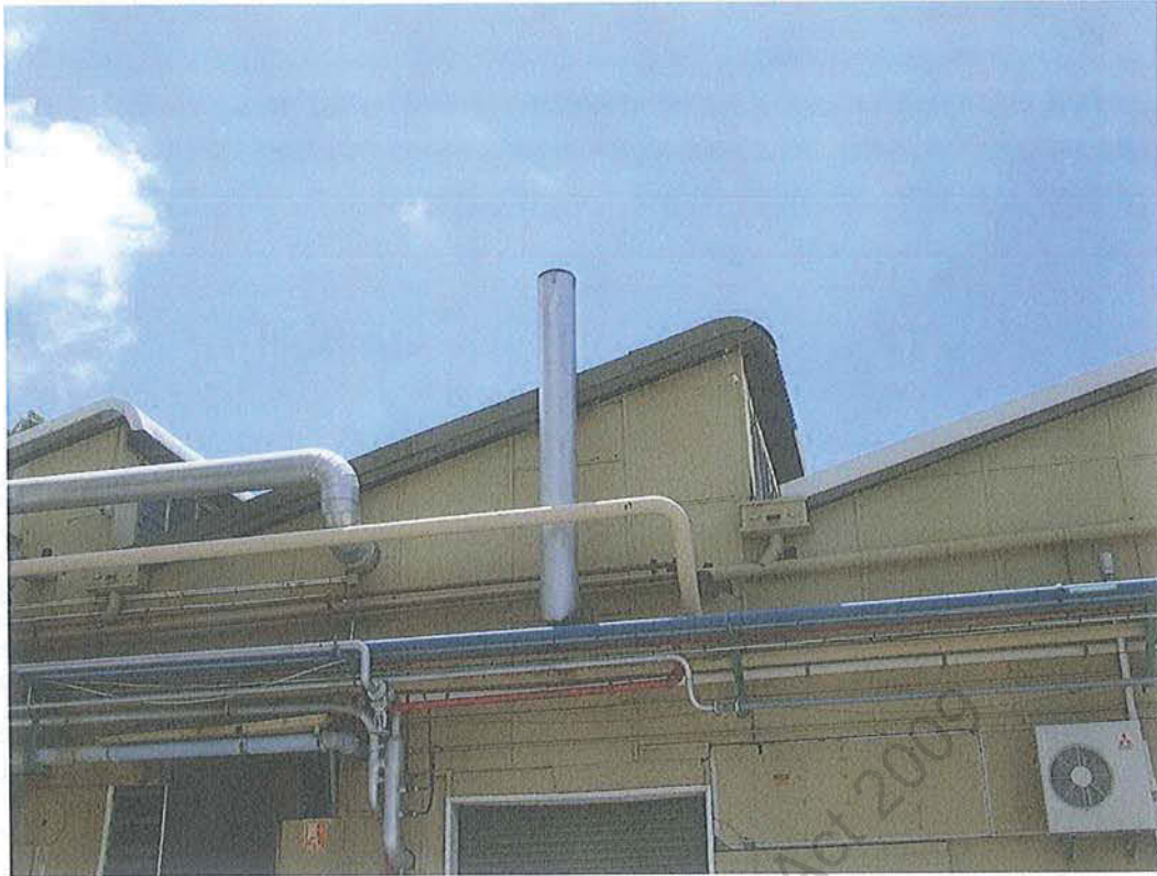
View of the generator exhaust stack. No labelling or sampling access is required.
