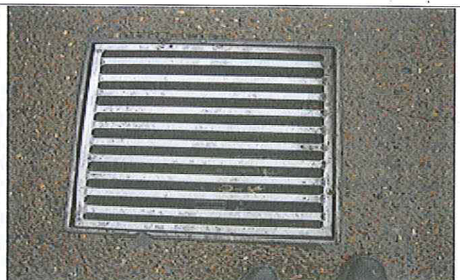
Photo: 1010678 –Stormwater fabric filter.
