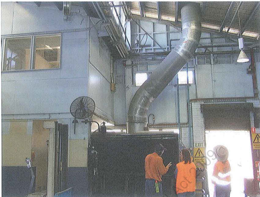
View of Release Point 4 – Mould shop solid film lubricant spray booth. The booth is fitted with a fabric filter as required by condition B13.
