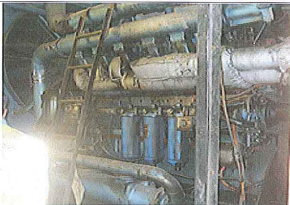
Photo: 1020676 – This is the diesel engine that runs the generator.
