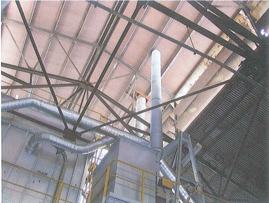
View of Release Point 5 – stannic chloride fabric filter dust collector (baghouse). RP5 was not compliant with the labelling requirements of conditions B11 and B12. Direct access to the sampling ports looked to be via the roof. This situation should be checked for compliance with the requirements of Australian Standard AS 4323.1-1995 Stationary source emissions- Selection of sampling positions .
