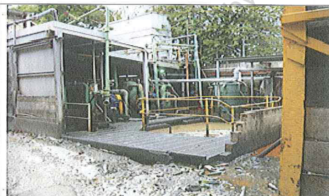
Photo: 1020664 – Back of main production building – the production building is fully bunded including the area shown in the picture – The water here is cooled in the cooling pond and recycled through QG1.
