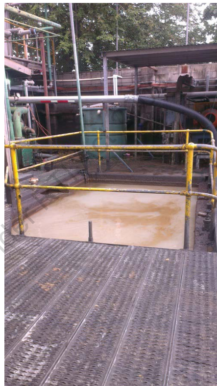
Photo 16 – Water treatment system, water returned to production.
