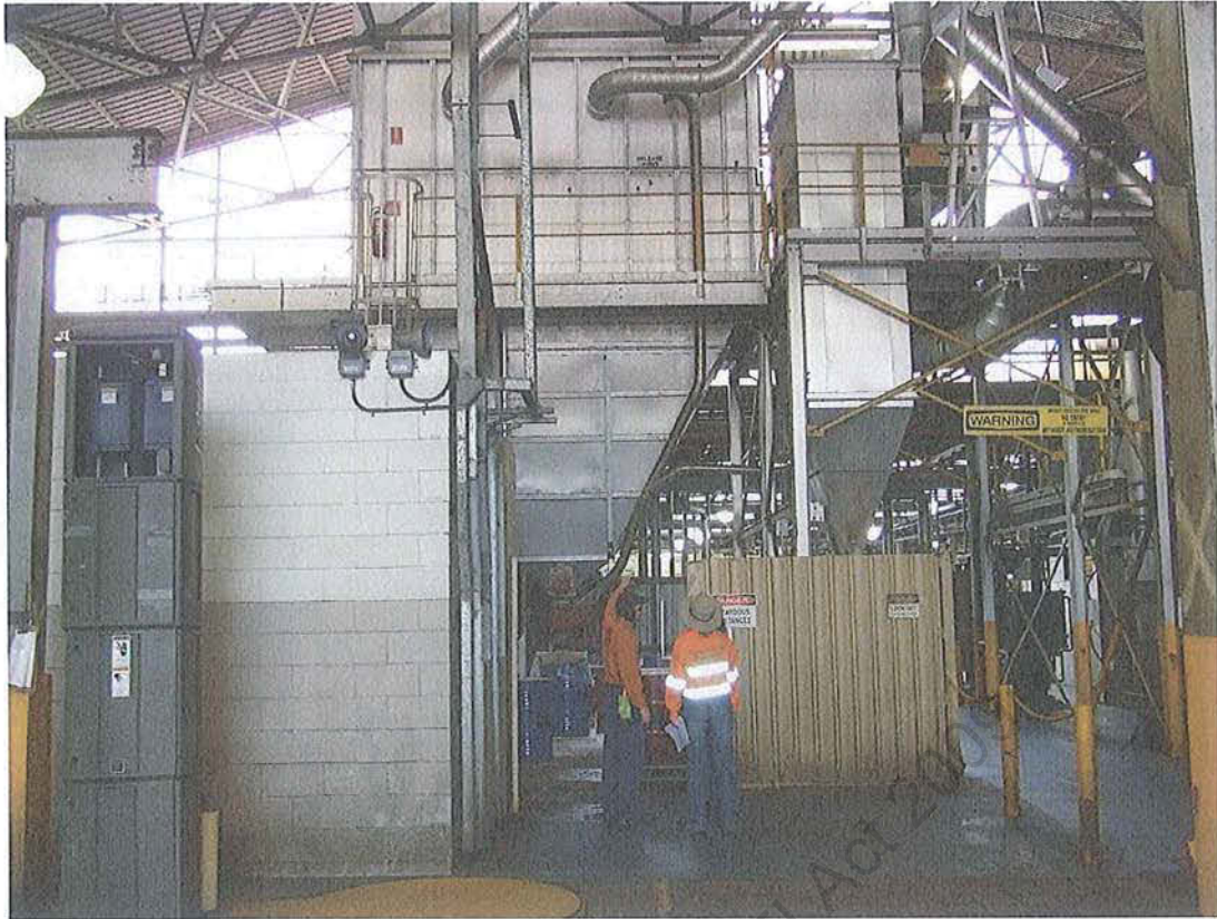
View of the stannic chloride fabric filter dust collector (baghouse). Condition B16 requires that the collector is operated at an efficiency of no less than 99.7 percent for stannic chloride and ammonia chloride particulate matter. O-I was not able to describe how the collection efficiency for the collector was determined or maintained.
