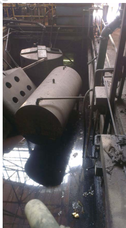
Photo 6 – Water treatment system.
