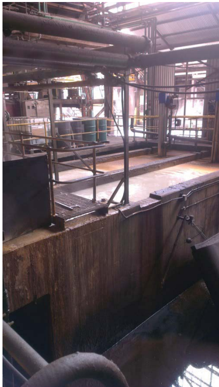
Photo 9 – Water treatment system.
