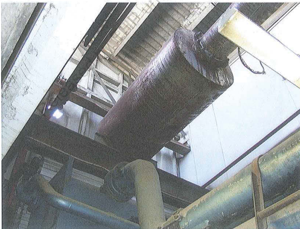
View of the generator muffler.
