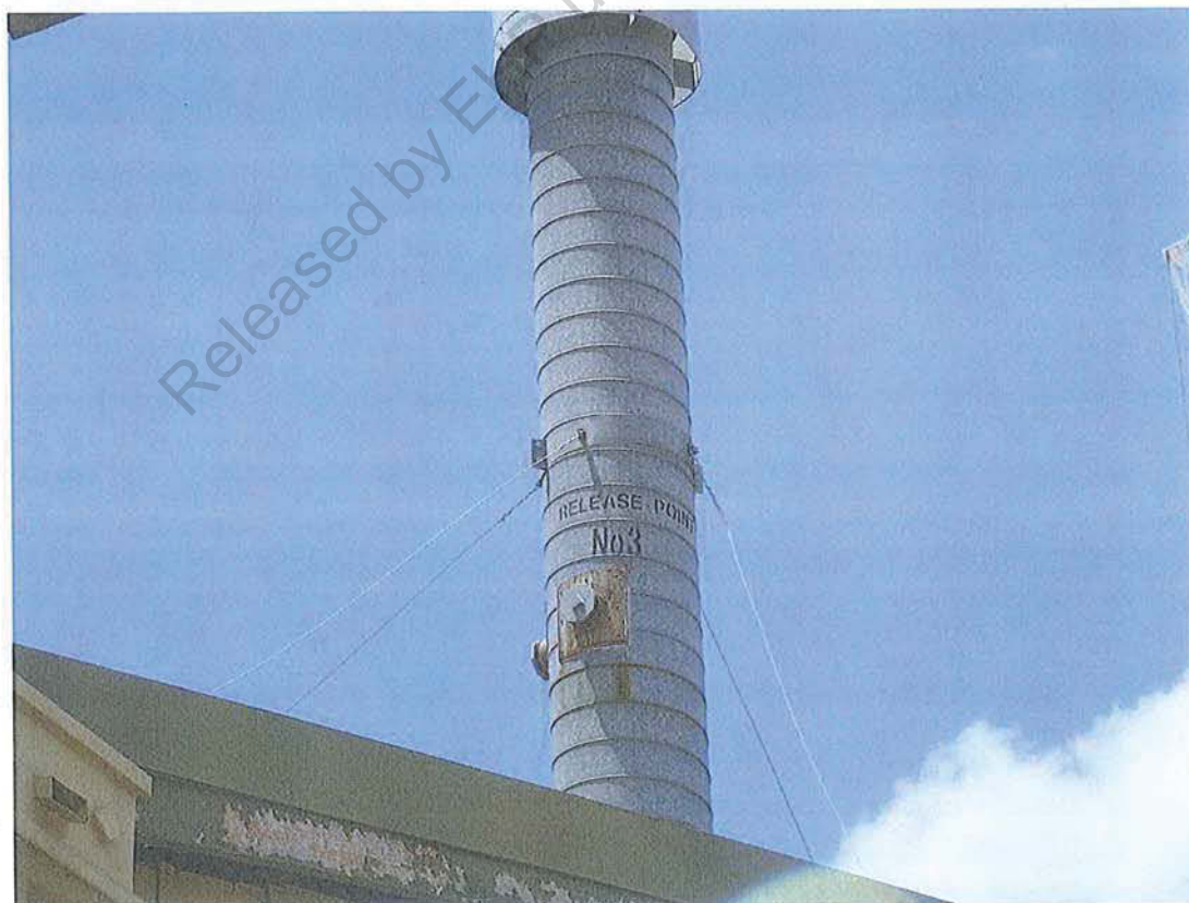
View of the RP3 sampling port. RP3 complied with conditions B11 and B12 as it was conspicuously labelled, and the labelling was clearly visible from ground level and at the sampling point. Direct access to the sampling ports looked to be via the roof. This situation should be checked for compliance with the requirements of Australian Standard AS 4323.1-1995 Stationary source emissions- Selection of sampling positions .
