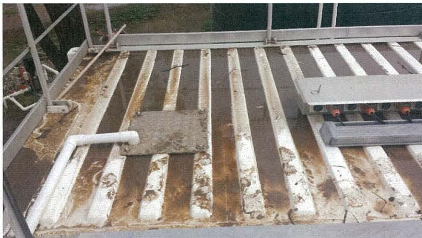
Figure 1: Spill on top of STP (front)
