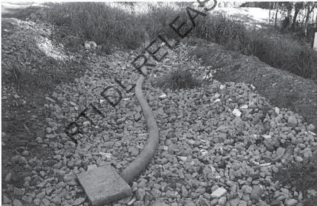
Photo 6: Hose to pump leachate from Cell 8 to the outlet
