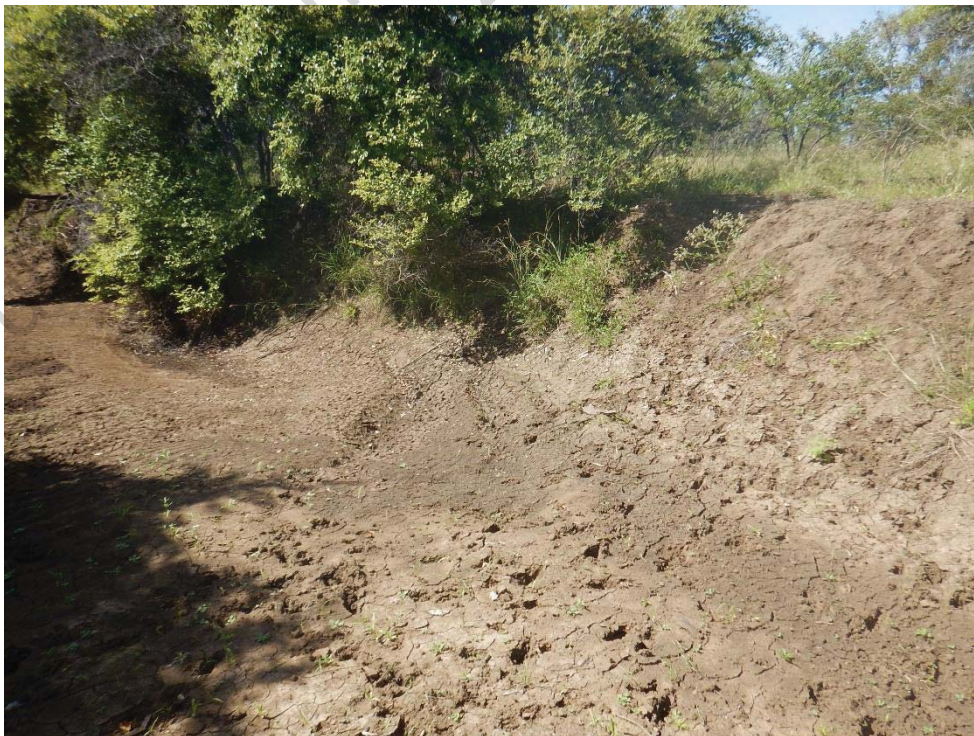
Figure 6.1 Bank Erosion and Undercutting Downstream Of TMC-US1
