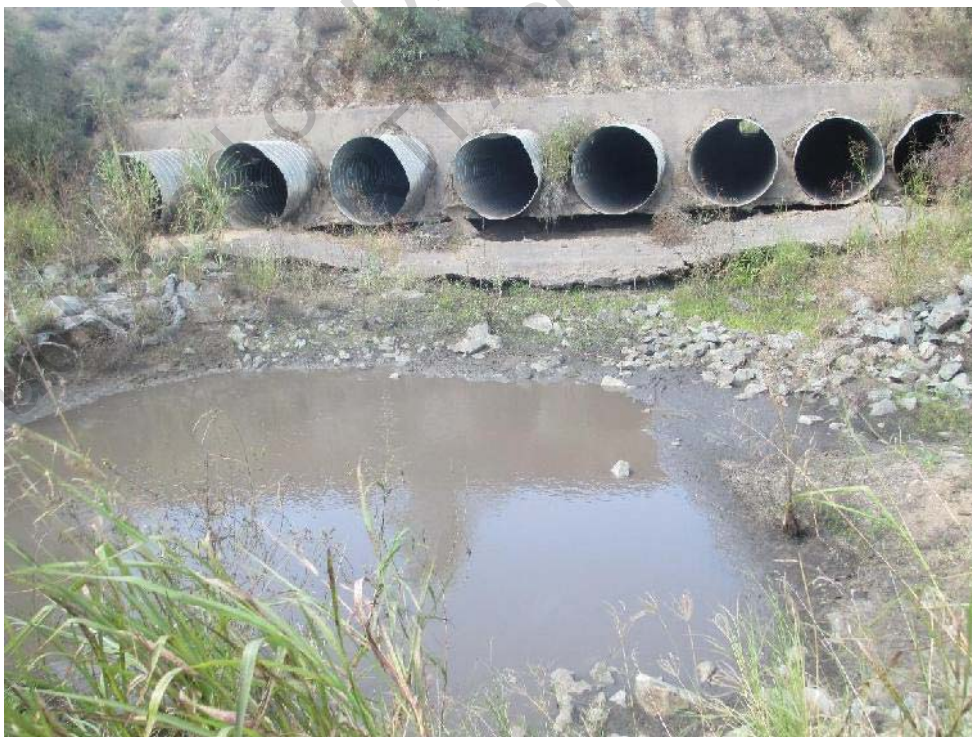
Figure 6.12 Scour Hole And Damaged Apron At Downstream Headwall Of High Level Haul Road Culverts
