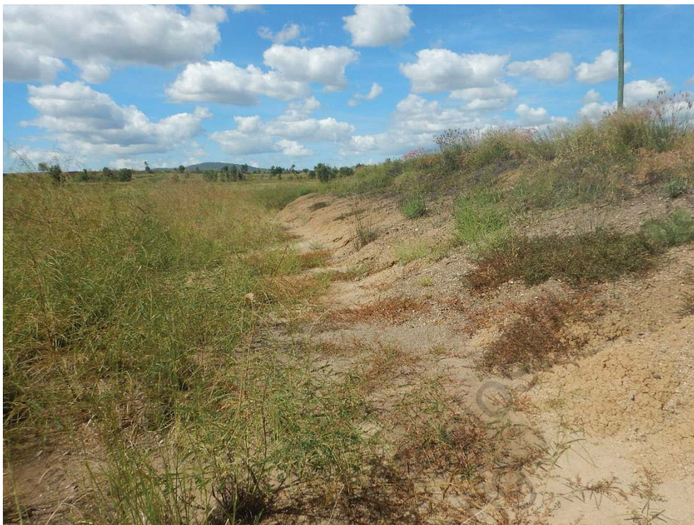
Figure 6.21 Scour at Toe of Embankment Upstream of Light Vehicle Road Crossing
