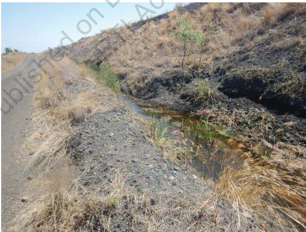
Photo 10 Seepage at toe of First Rejects Wall Lift above Starter Bund - Western Side of Cell 2 Near with Cell 3
