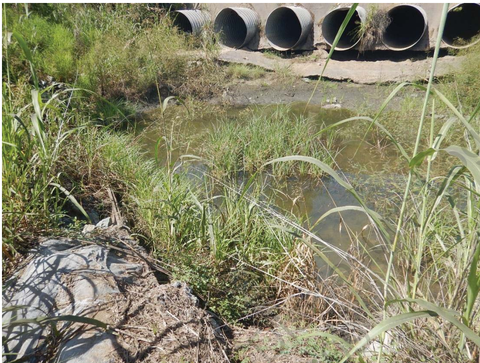
Figure 6.13 Scour Hole and Damaged Apron at Downstream Headwall of High Level Haul Road Culverts
