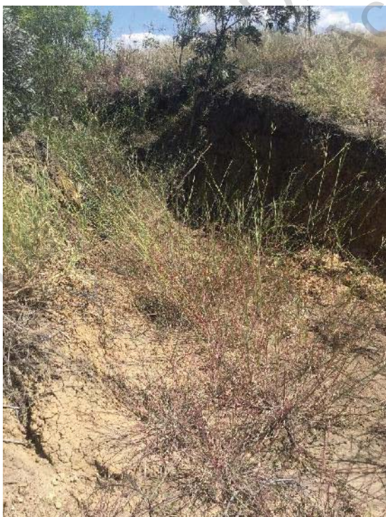
Figure 6.22 Secondary Smaller Erosion Gully Near Light Vehicle Road Crossing
