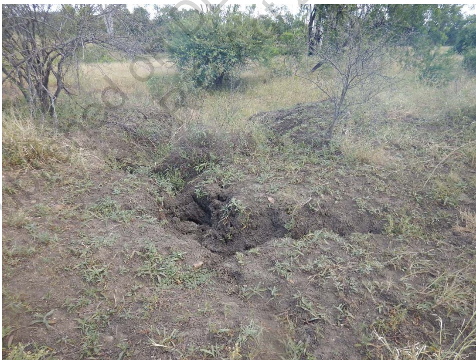
Figure 6.29 Gully Erosion on Right Bank Downstream Of TMC-DS3
