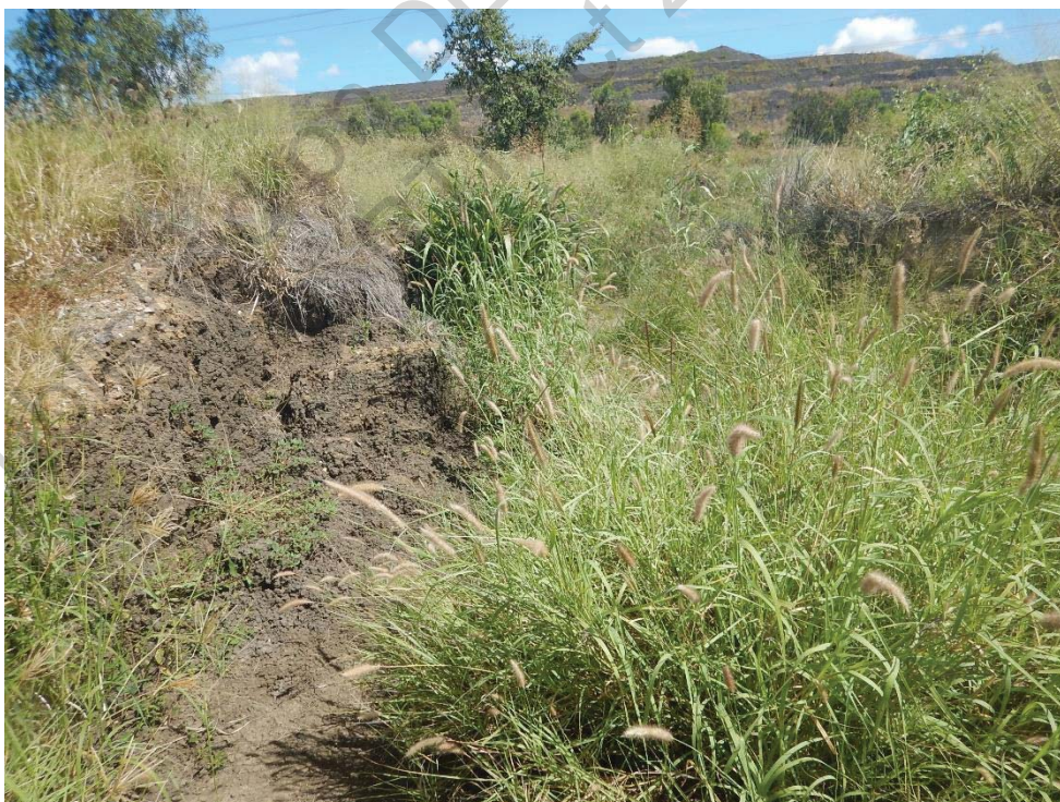
Figure 6.18 View Along Erosion Gully on Left Bank of Diversion Downstream Of TMC-Div2
