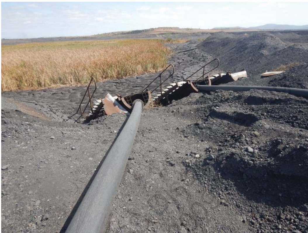
Photo 17 Pump Discharge Lines from Cell 3 Decant Pond into Decant Inlet of CDA1/2
