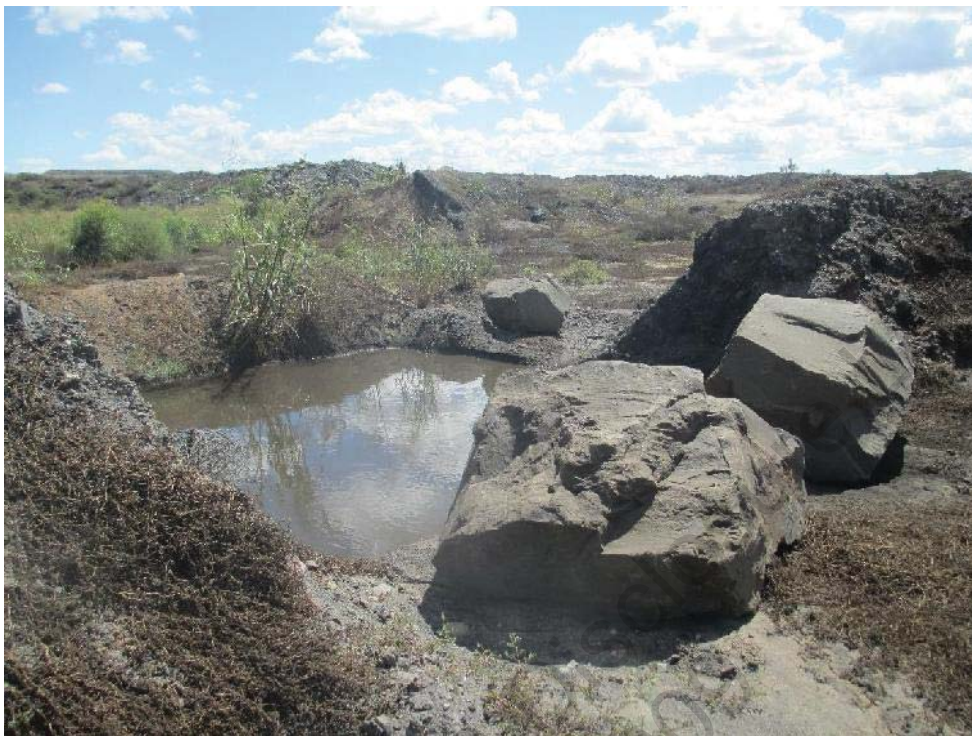
Figure 6.11 Scour Hole Downstream Of Haul Road Causeway
