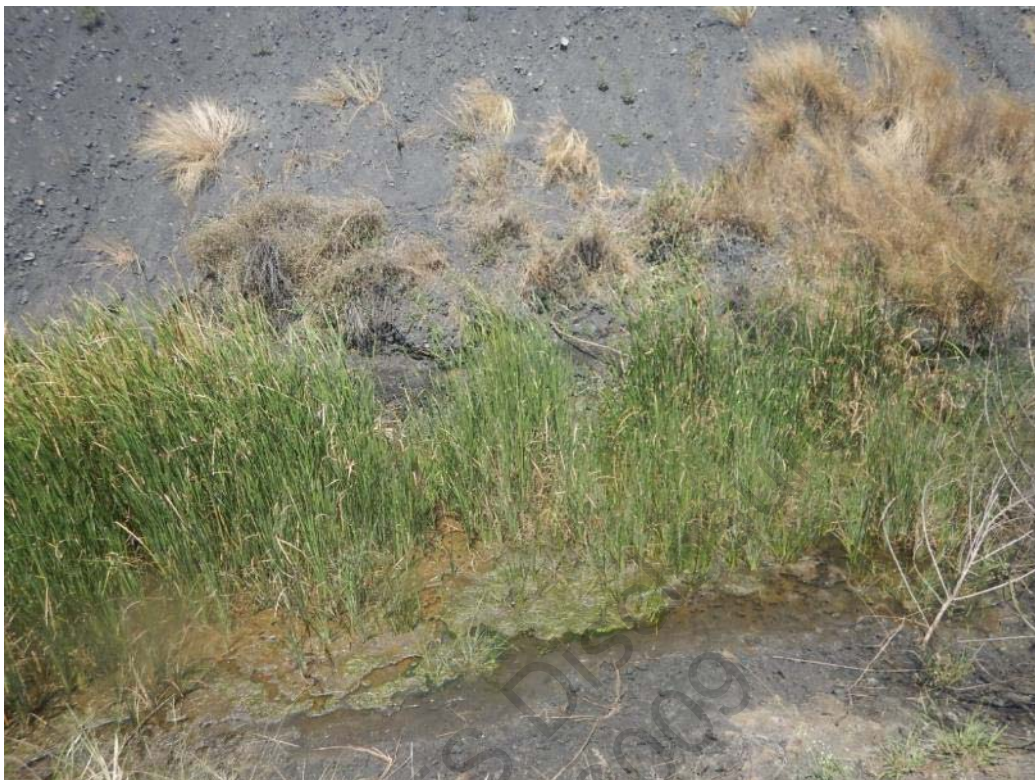
Photo 19 Seepage Expression Above Starter Bund – Eastern Side of Cell 4 near Cell 3
