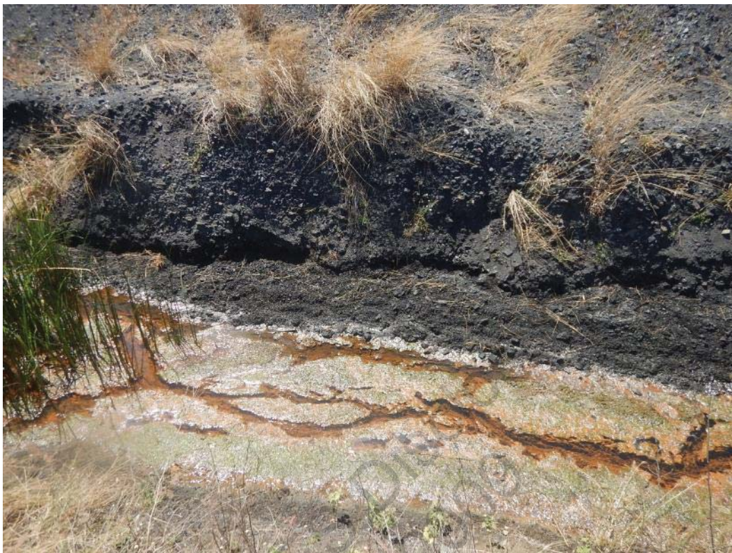
Photo 13 Seepage Expression Above Starter Bund – Western Side of Cell 3
