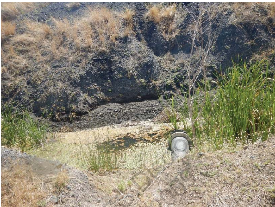
Photo 7 Ponding in Drain above Starter Bund - Northern Side of Cells 1 and 2
