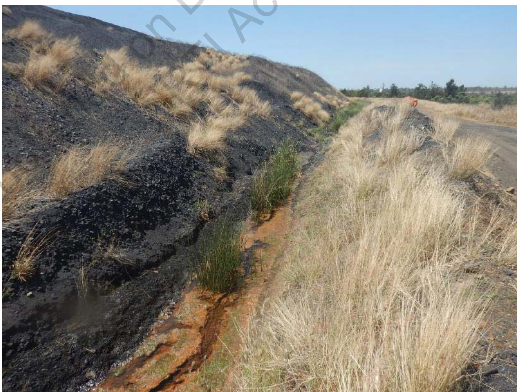
Photo 10 Western Side of Cell 3 Including Seepage Flows in Drain above Starter Bund
