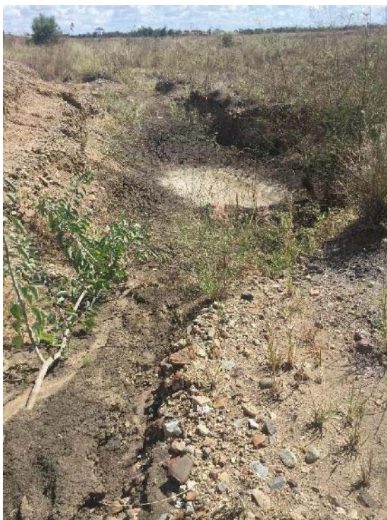
Figure 6.23 Scour At Toe Of Embankment Upstream Of Light Vehicle Road Crossing
