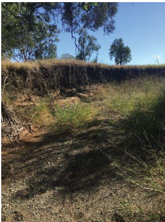
Figure 6.3 Bank Erosion Upstream Of TMC-US4
