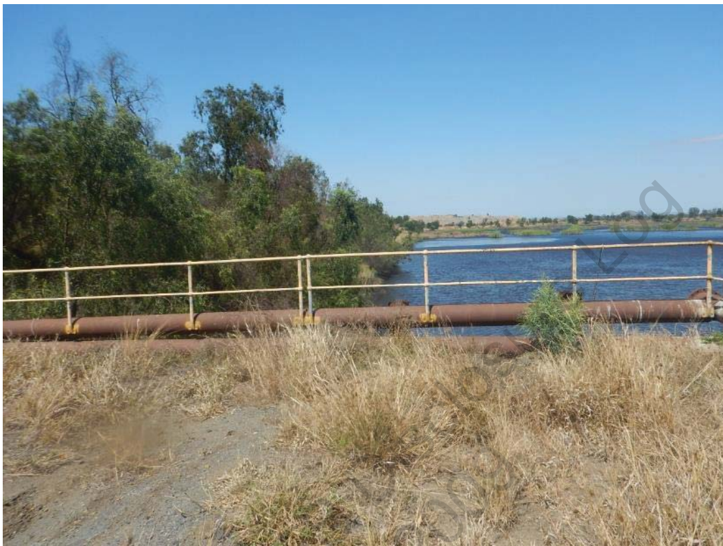
Photo 5 Return Water Dam and Trees Growing on Return Water Dam Batter and Northern Starter Bund
