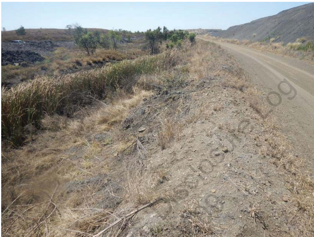
Photo 17 Trees Growing on Outside Face of Starter Bund - Eastern Side of Cell 4
