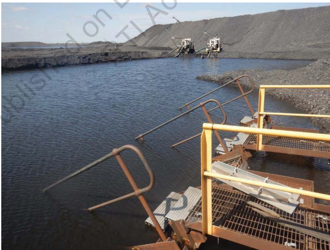
Photo 4 Decant Inlet Structure and Two Trailer Mounted Pumps Located at Cell 3 Decant Pond
