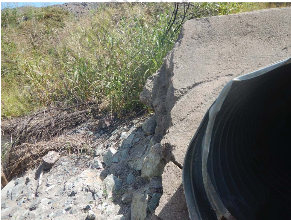
Figure 6.10 Damaged Headwall of High Level Culverts at Upstream Side of Haul Road
