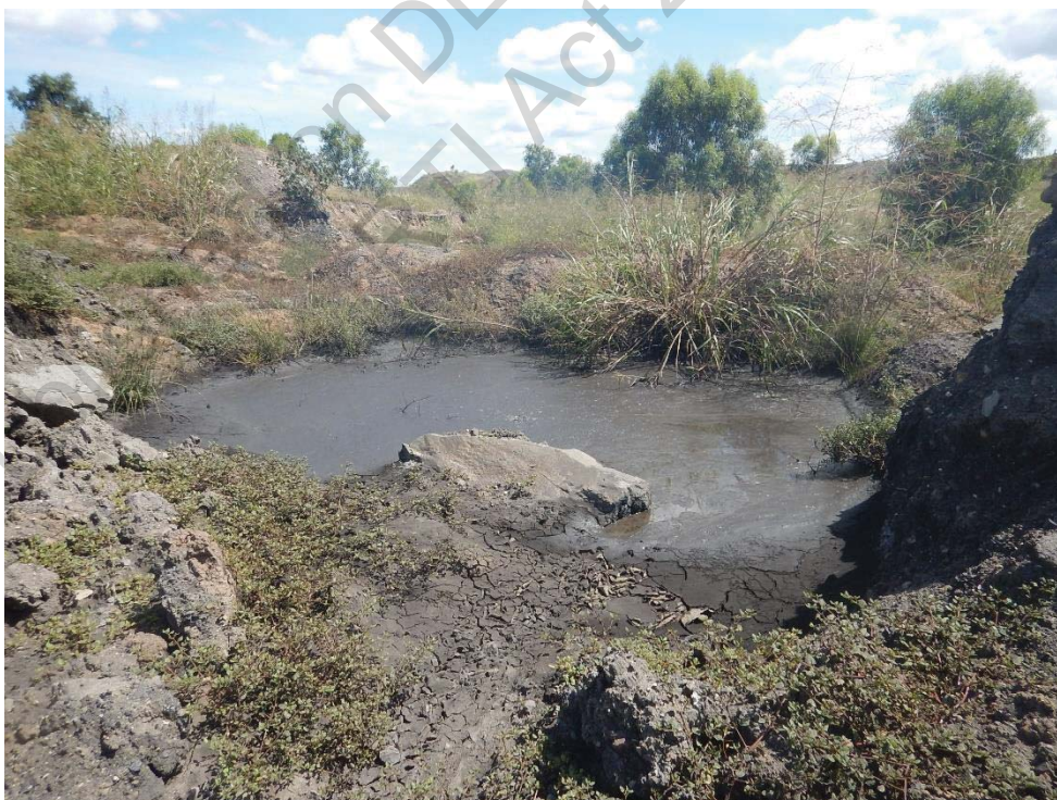
Figure 6.12 Scour Hole Downstream of Haul Road Causeway
