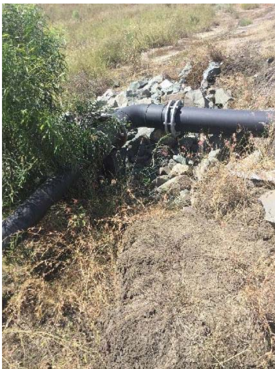
Figure 6.19 Sd5 Release Pipeline Off Mounting Blocks
