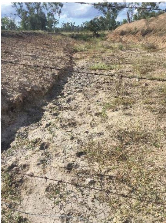
Figure 6.33 Erosion At Toe Of Left Bank Of Drain Downstream Of Drake 1 Pit And Drake 2 Pit
