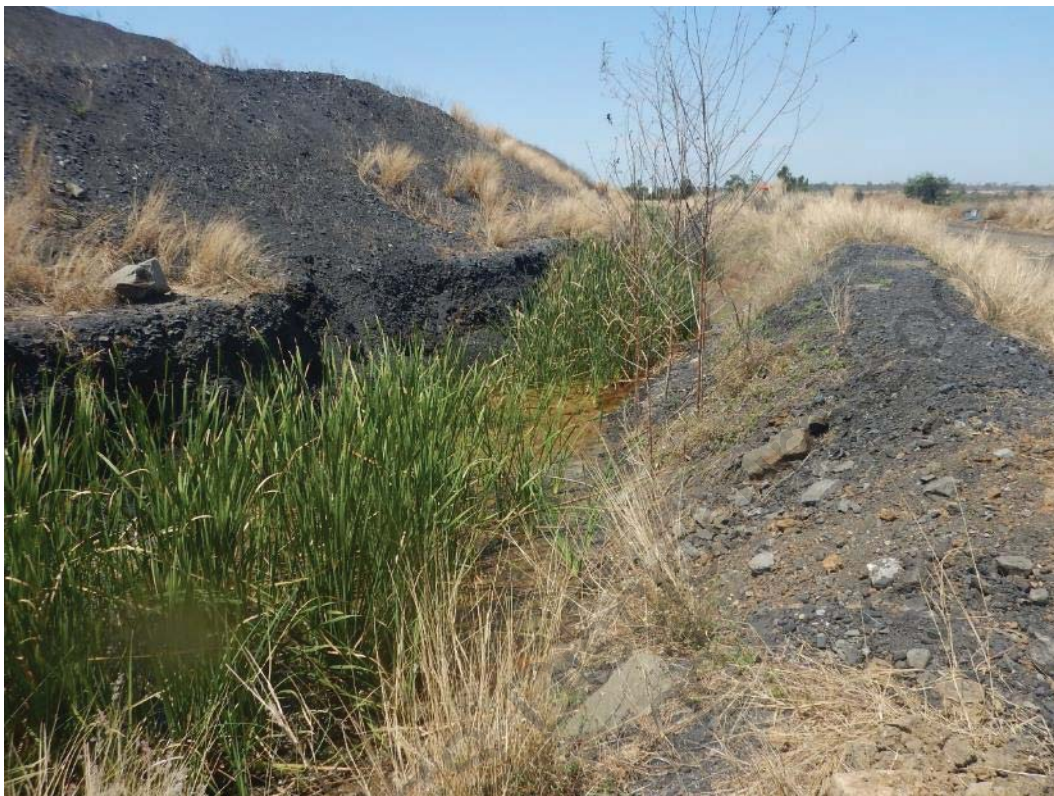
Photo 15 Reeds Growing in Drain above Starter Bund - Western Side of Cell 3
