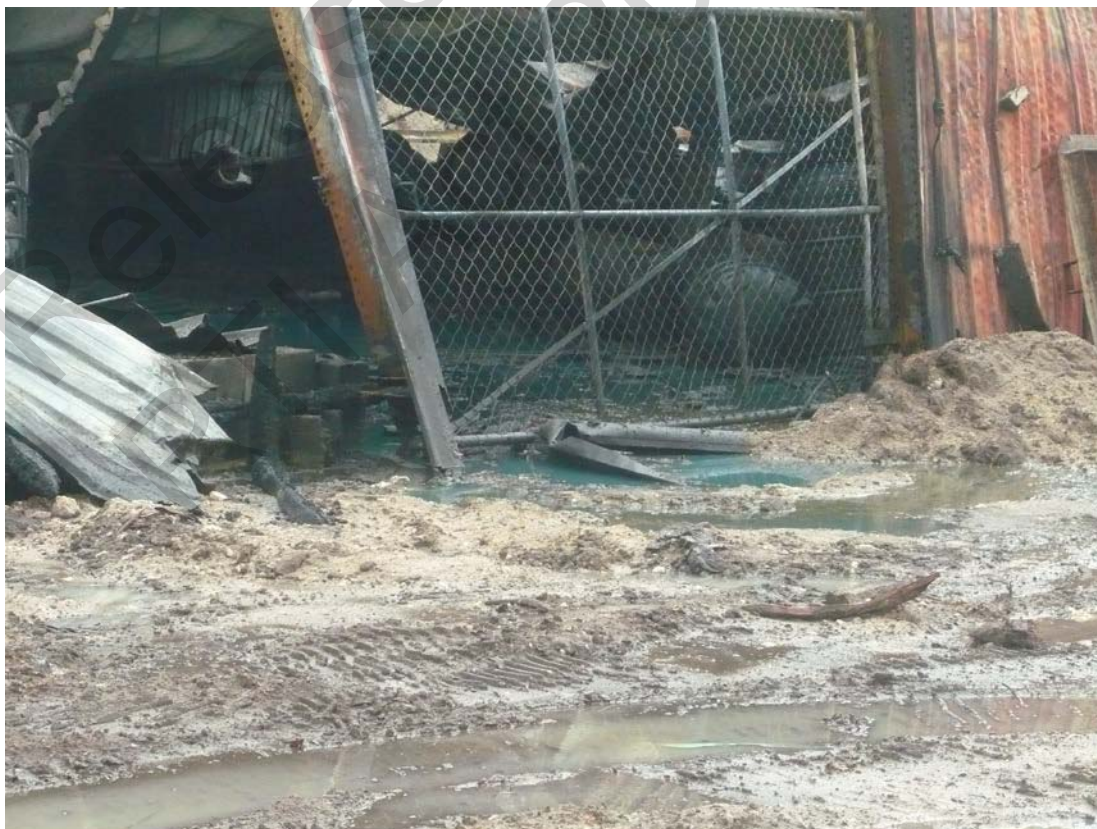
Photo 11 – Contaminants exiting the building due to the rainfall. Photo taken of the northern end of the building parallel to Potassium Street.
