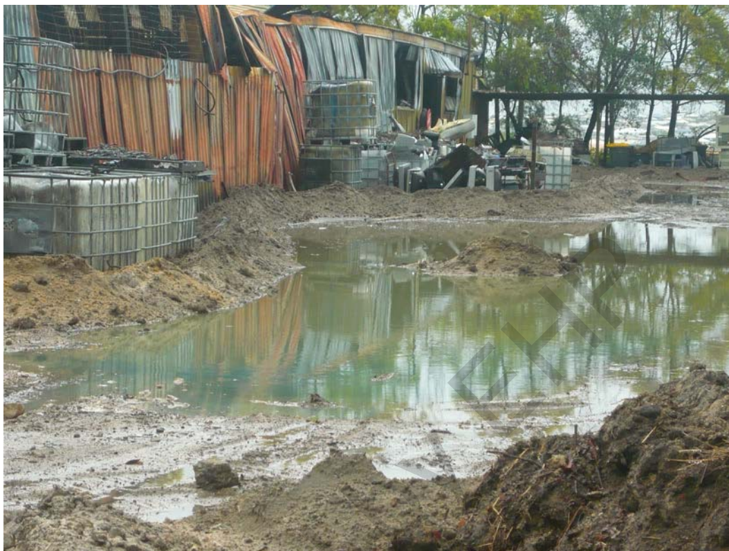
Photo 10 – Close up of the water pooling within the bunded area at the front of the building (photo is looking south from the northern end of the building – parallel to Potassium Street). Please note the blue sheen on the water indicating that contaminants are exiting the building due to the rainfall.
