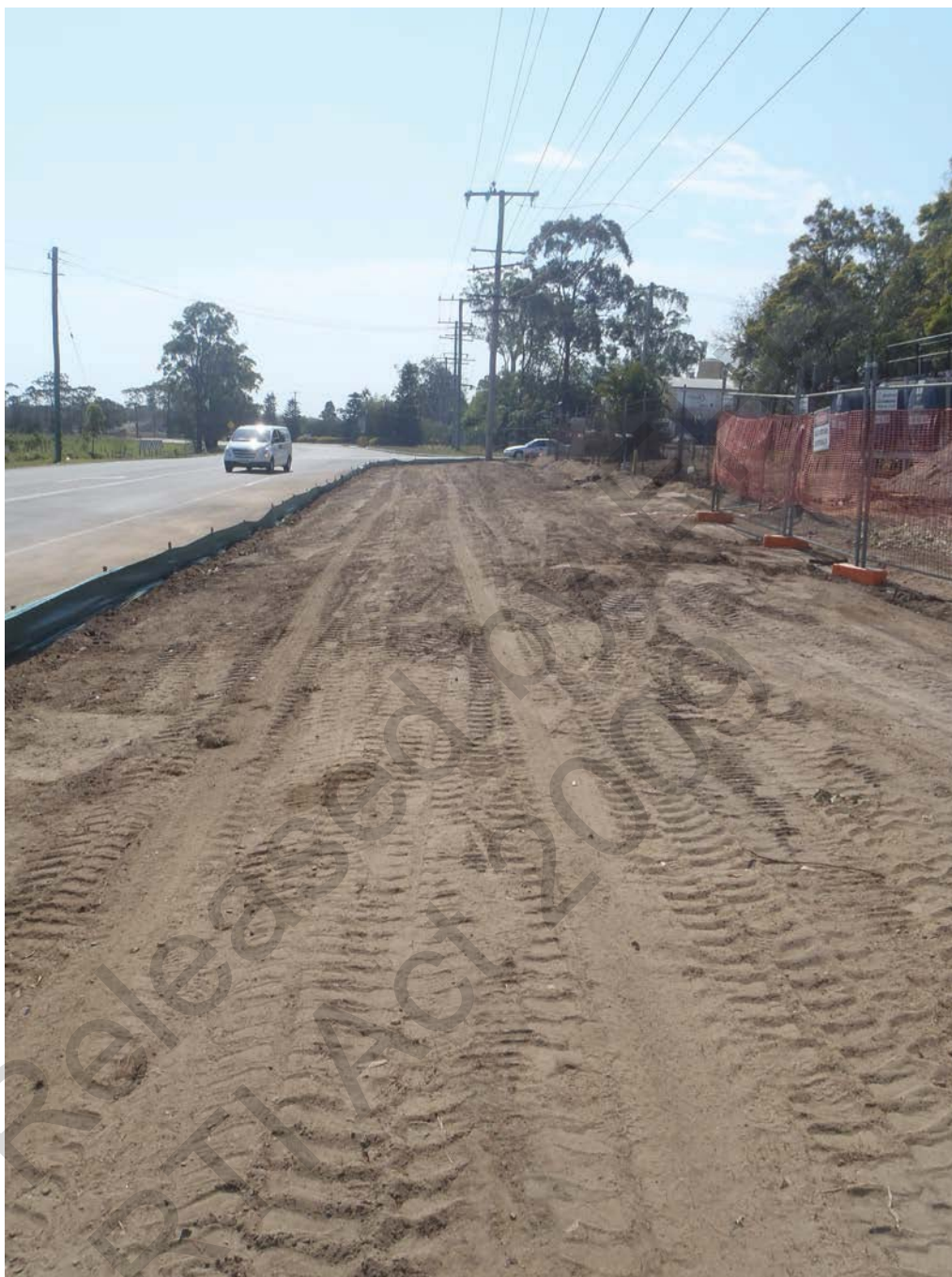
Photo 13 – This photo is taken from the same location as photo 12 but facing west. It shows the work Moreton Bay Regional Council has done along the footpath of the site to remediate the contaminated land. Please note the sediment fence that has been placed on the site boundary.
