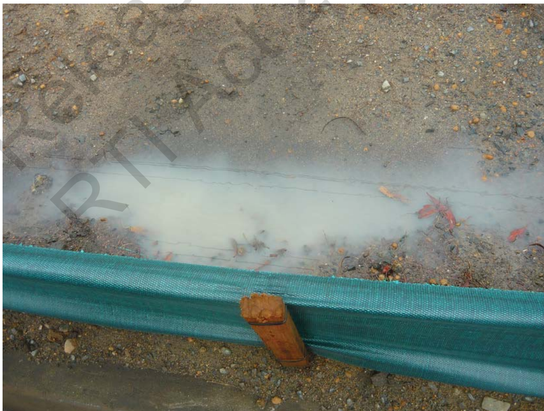
Photo 5 – Pooling rainwater seen in photo 4 above, at the sediment fence along the footpath of Boundary Road. Please note that there are not contaminants evident in the water.
