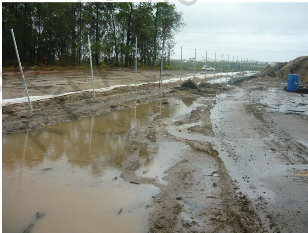
Photo 13 – Pooling of water on the eastern side of the building. Please note no contaminants can be seen in the pooled water.
