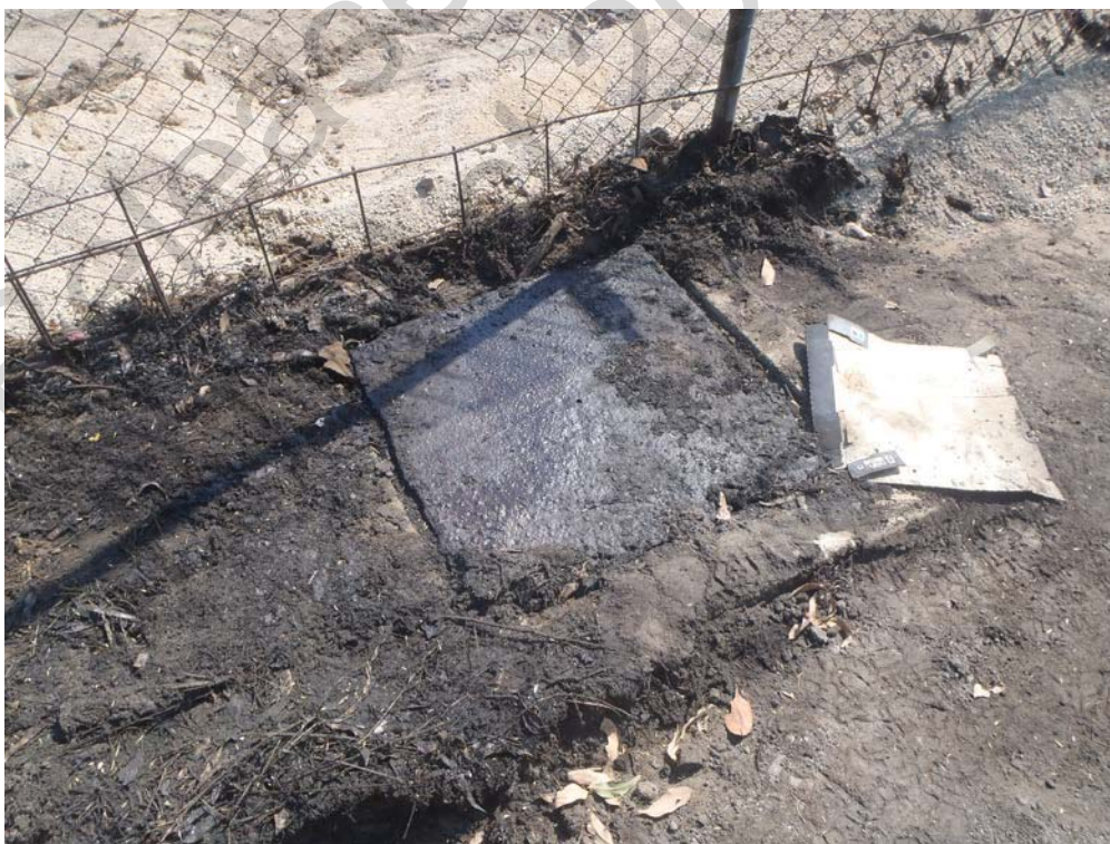
Photo 11 – This photo is taken from the boundary of the site along Boundary Road. This is a sump that catches contaminants before stormwater flows into a drain on the other side of Boundary Road (Stockland land). This sump is currently contaminated and must be remediated as part of the site clean-up.
