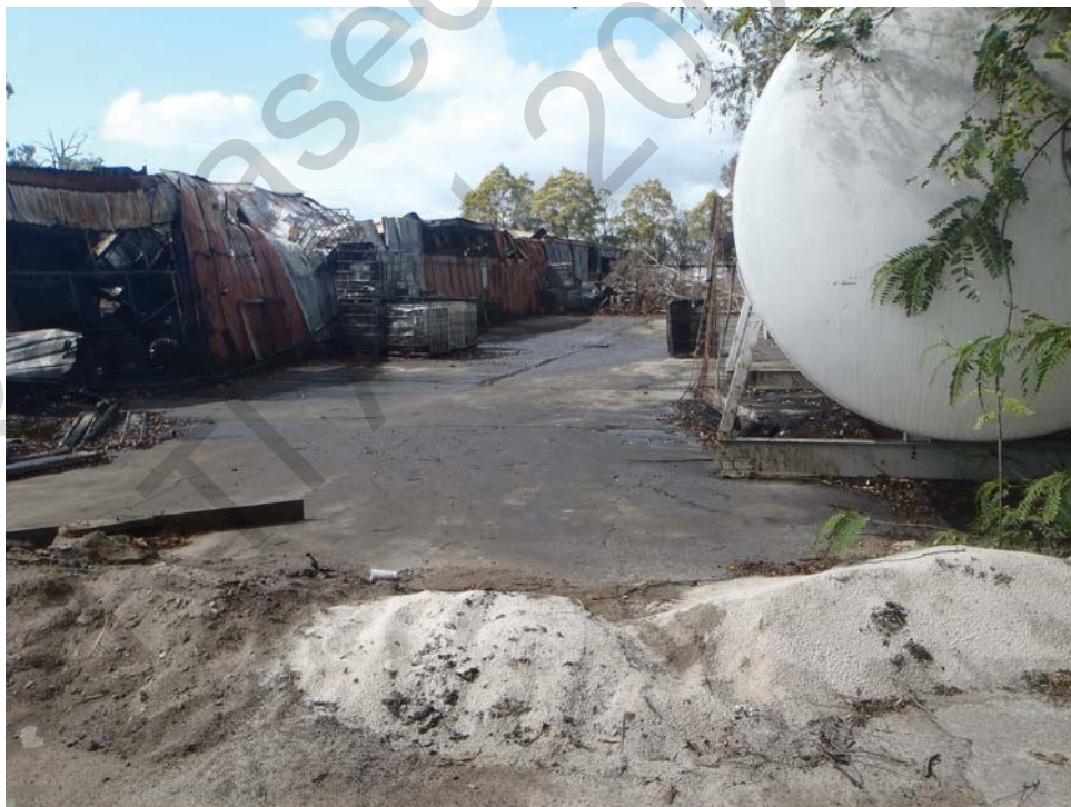
Photo 1 – The front of the destroyed building along Potassium Street (facing south). No change from the site visit on the 18 December 2012. Note some moisture on the ground, likely to be from rainfall. Also note that the bund is still in place around the main building.
