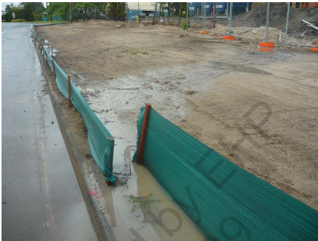
Photo 6 – Pooling rainwater seen in photo 4 and 5 above, at the sediment fence along the footpath of Boundary Road. Please note that there are not contaminants evident in the water.
