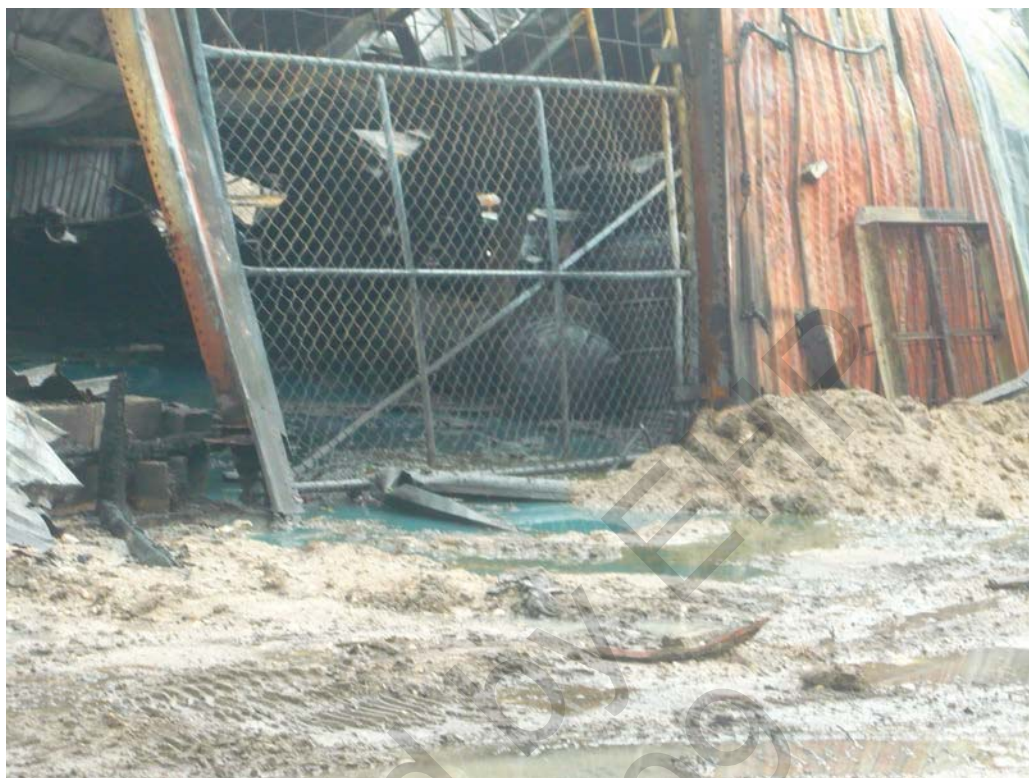
Photo 12 – Close up of the contaminants exiting the building due to the rainfall. Photo taken of the northern end of the building parallel to Potassium Street.
