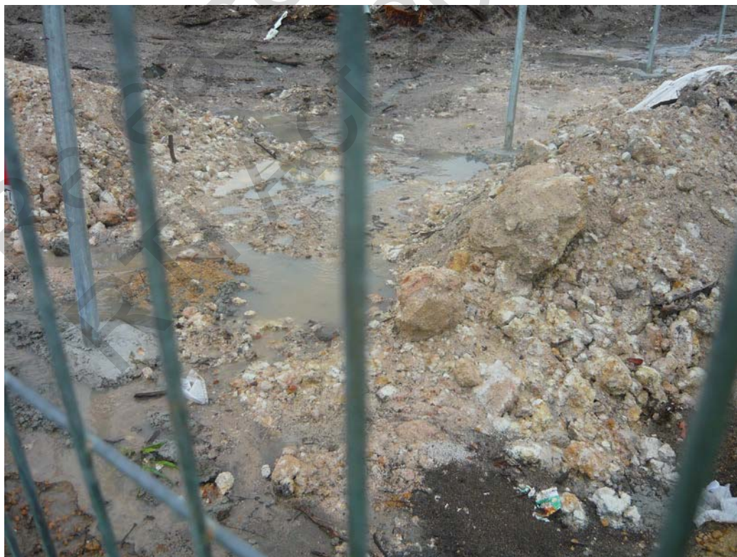
Photo 7 – The break in the bund wall (referenced in photo 4). This bund wall was installed by Projex Partners (DSDIP consultants). It is broken where the bund turns the corner and runs parallel with Boundary road. As the bund is broken where the new fence posts start, it is possible that the break could have been caused by the fence contractors (the fence contractors were seen onsite on Thursday 24/01/2013 – see file note)
