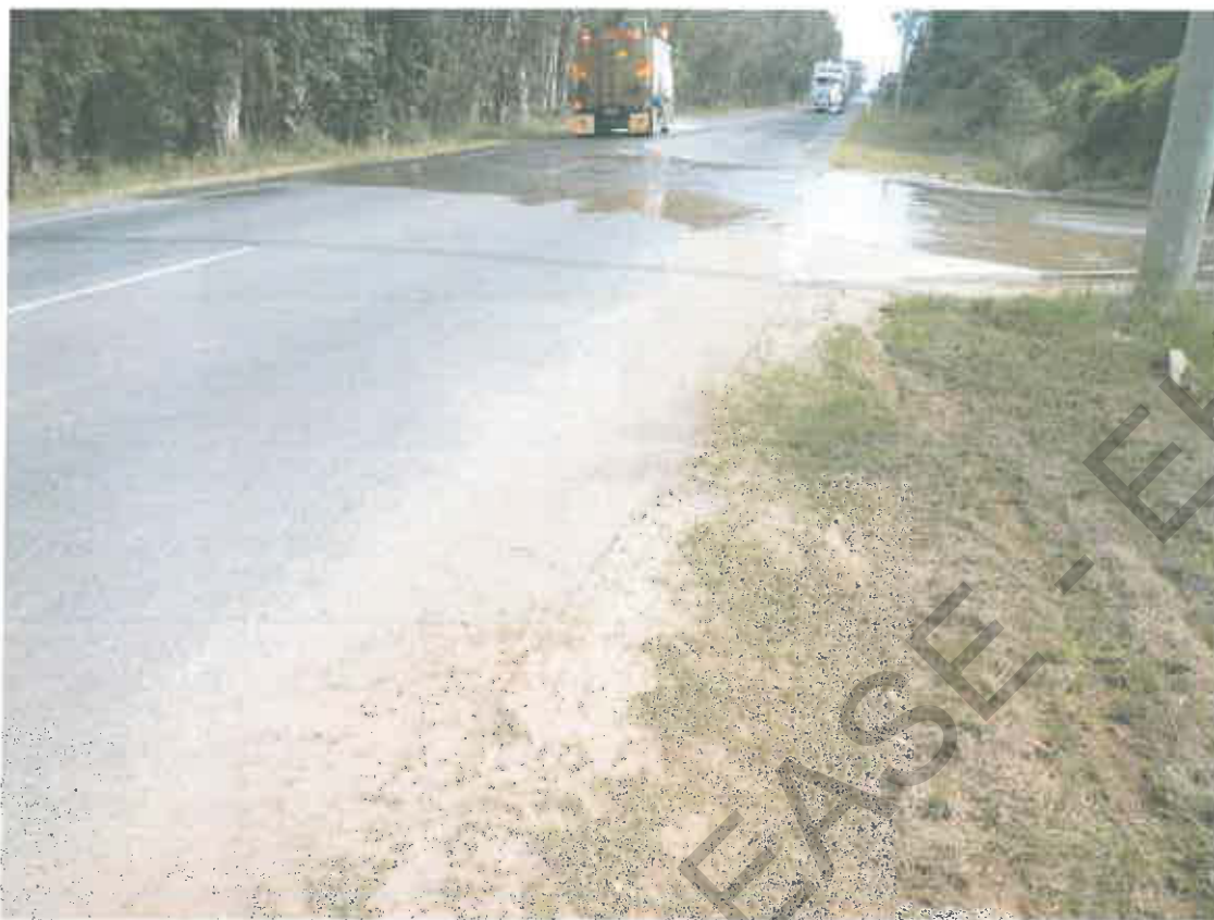
Figure 3 – Sediment on Road at Pimpama-Jacobs Well Road Entry Point 2
