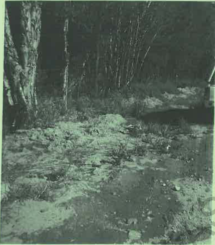
Figure 3 – Sediment along Behms Road adjacent to Waragap Entry/Exit point on Behms Road
