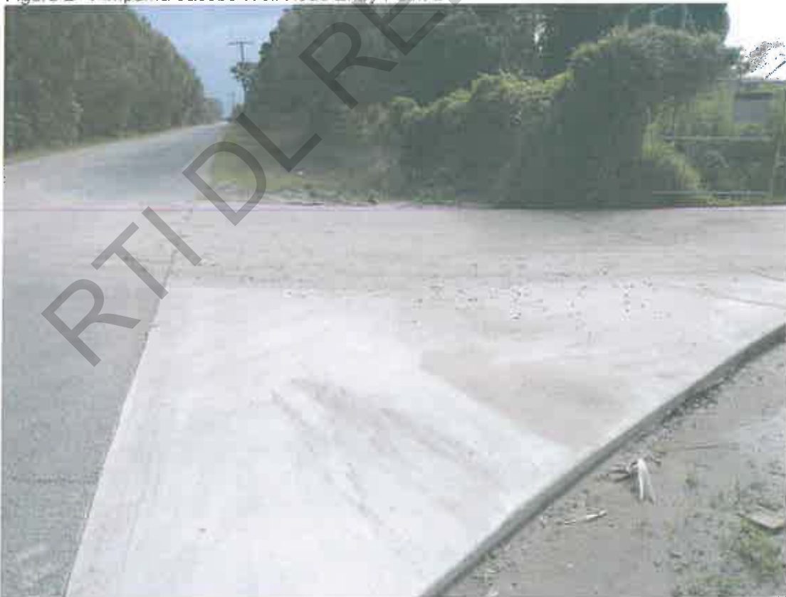
Figure 3 – Sediment on Concreted Entry way at Pimpama-Jacobs Well Road Entry Point 2
