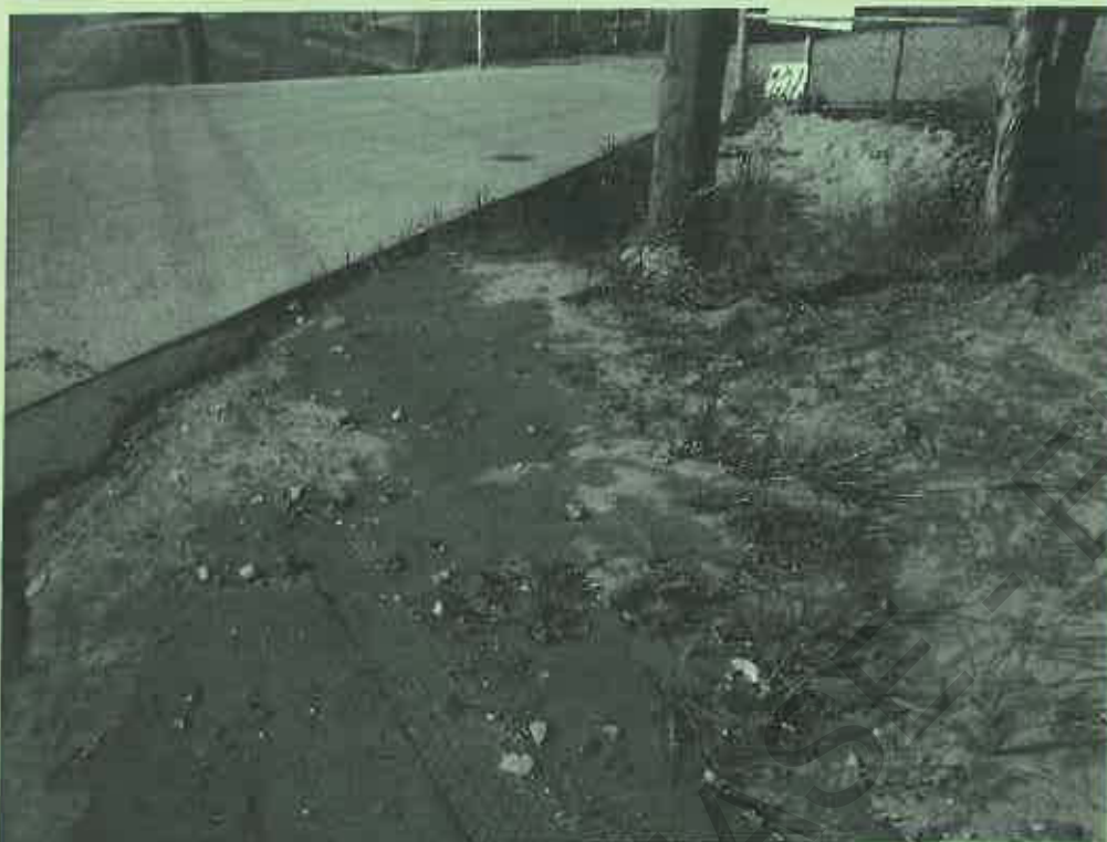
Figure 1 – Sediment adjacent to Waragap Entry/Exit point on Behms Road
