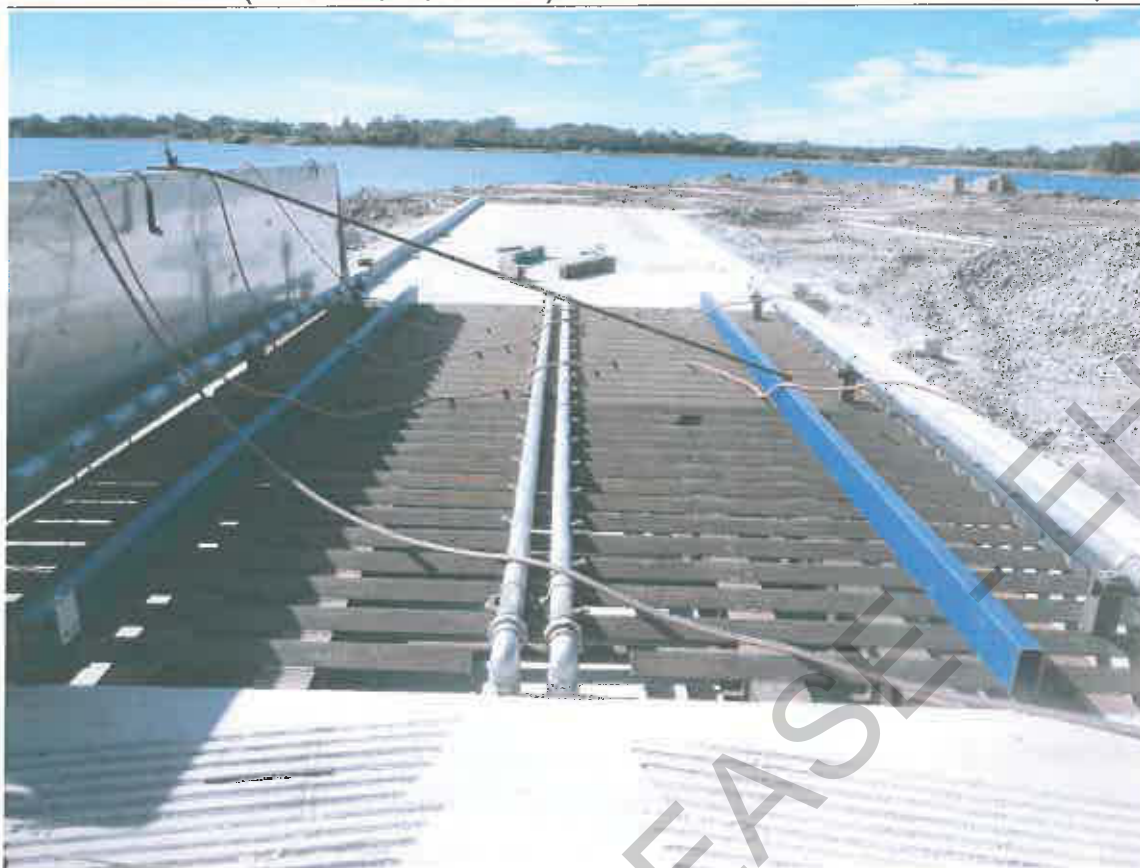
Figure 1 – Wheel Wash installed on site at Exit Point 1 (see map below)
