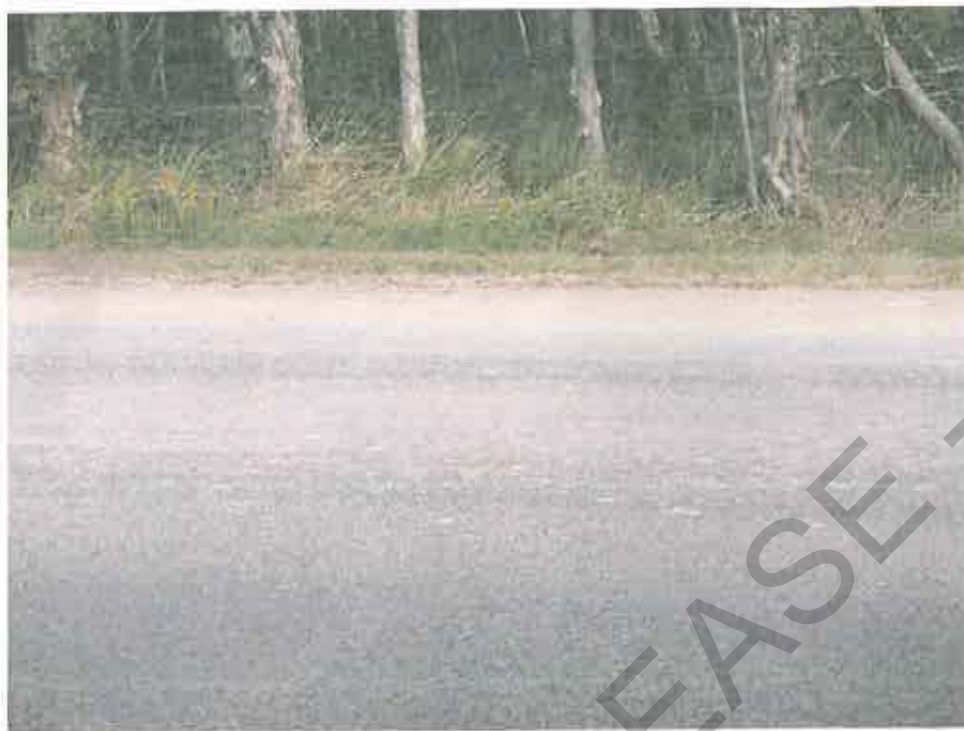
Figure 2 – Sediment on Road at Pimpama-Jacobs Well Road Entry Point 2 (see map below)
