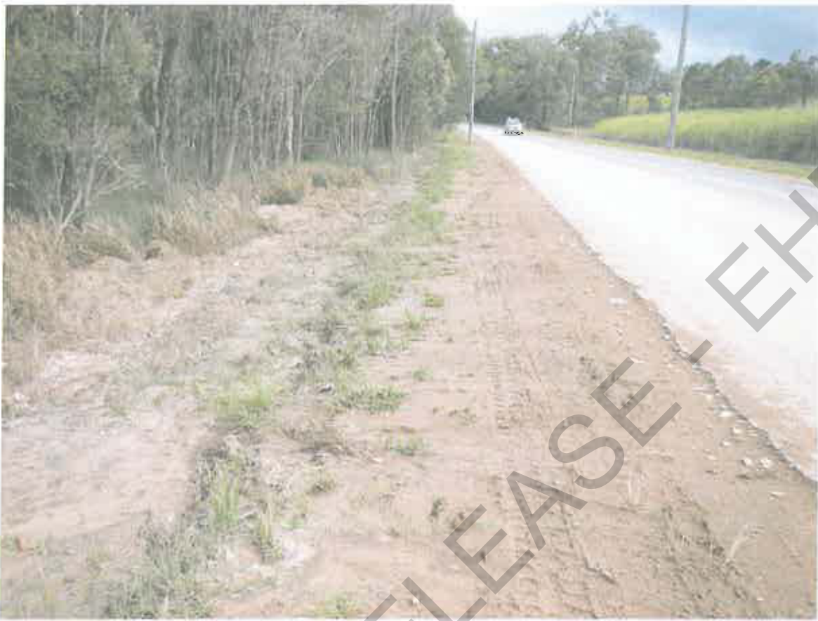
Figure 8 – Sediment building up on side of road
