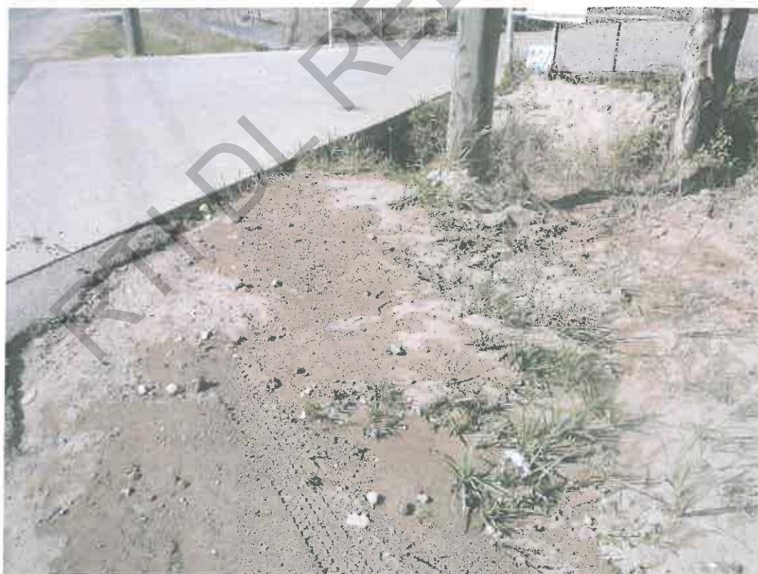
Figure 4 – Sediment adjacent to entry/exit point on Behms Road
