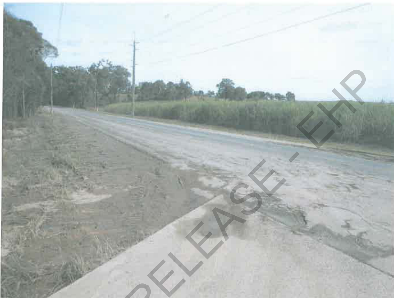
Figure 7 –Sediment on road on Behms Road from the site
