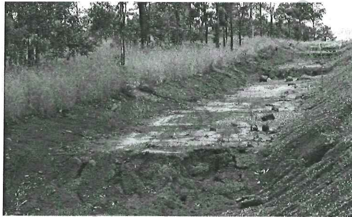
Figure 48 Stepped drain without energy dissipaters - note erosion that has occurred within 12 months of construction
