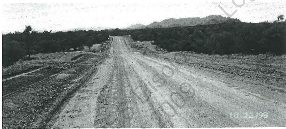
Figure 5 Example of well formed haulroad - note areas of impact beyond pavement surface
