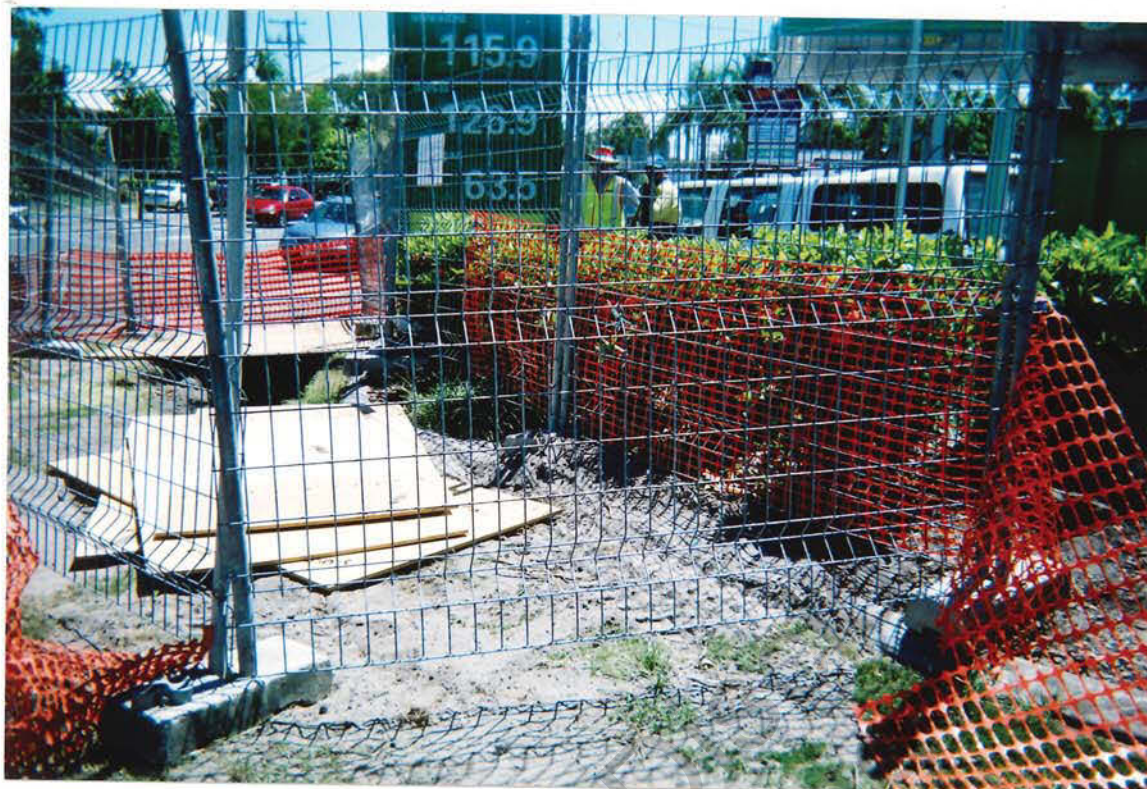
Photo 3 : 21/2/06 Energex pit on the footpath of BP at Mary St, Noosa
