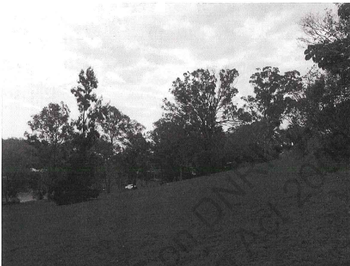
Site Photo 5 – Looking North Over Hillslope (Sinkholes Inside Orange Barrier in Background)
