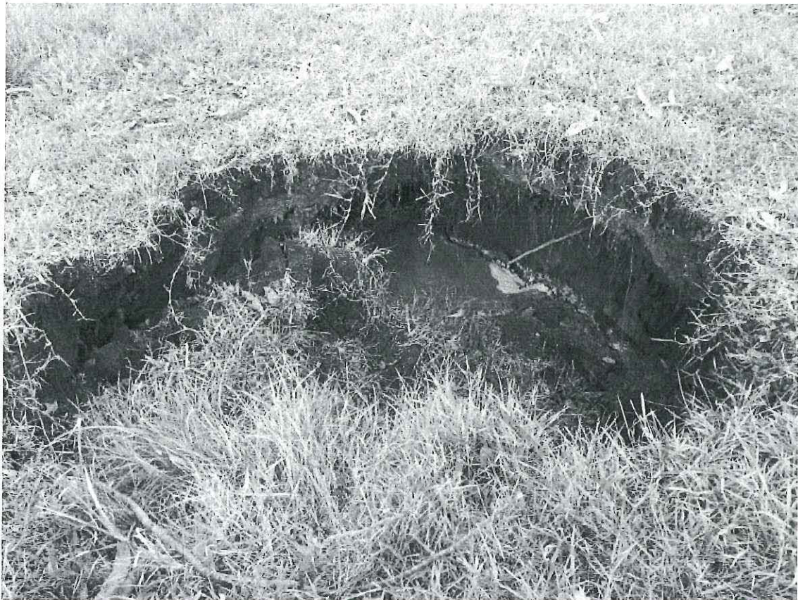
Site Photo 3 – Close Up of One of the Sinkholes
