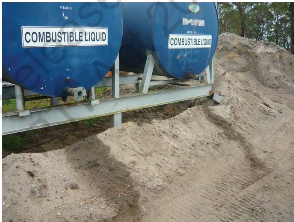
Photo 4 – Liquid storage tanks at the side of the main building (along Boundary Road). Note the moist soil under the taps in the tanks. This could indicate that the tanks are leaking or continually being emptied/released.
