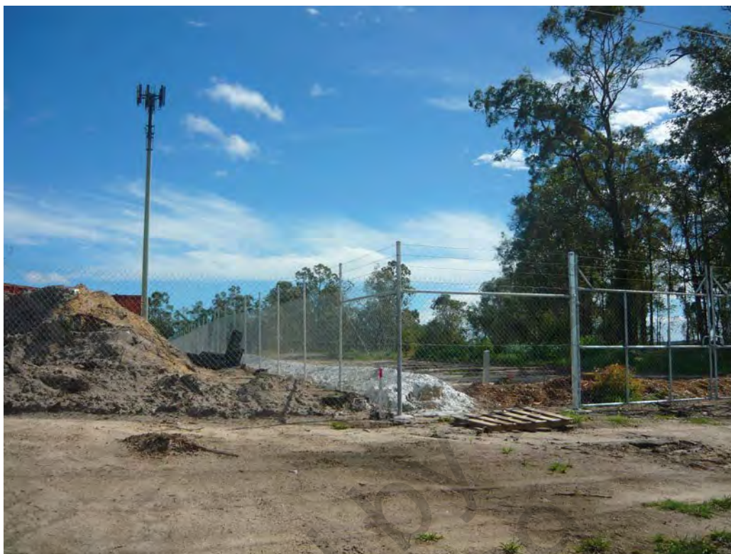
Photo 4 – The front of the incident site along boundary road (facing north). Note the polymer that has been applied to the top of the bund on the adjacent state land property. Also note further stock piles of material. JP to check when this material will commence being land farmed.
