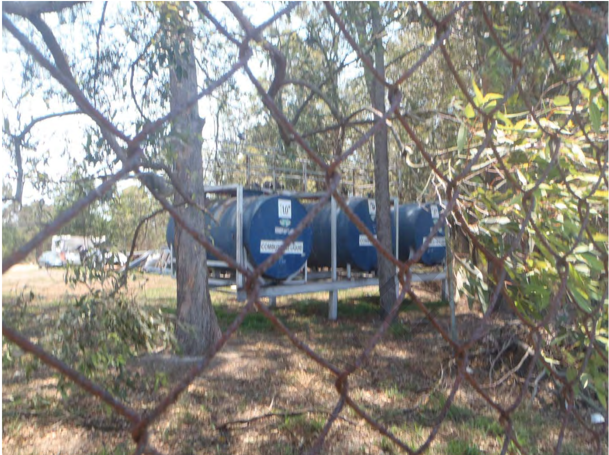
Photo 5 – Photo taken from Potassium Street looking at the southern end of the main building onsite. Note the combustible liquid storage.
