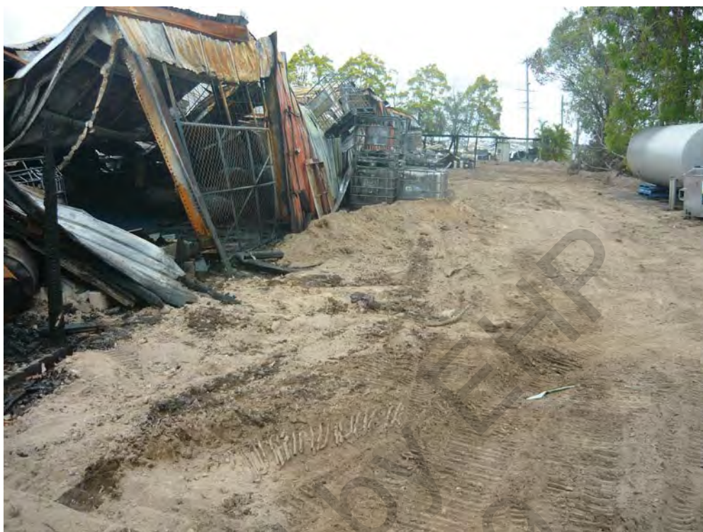
Photo 1 – The front of the destroyed building along Potassium Street (facing south). Further bunding has been placed around the building (see the bund on the left). Excess material has also been placed along the concrete slab to soak up any further containment in preparation for excess rainfall.
