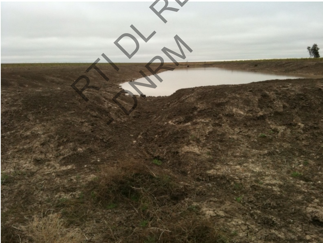
Breach in the bund, looking from near the Weir River along an element of the watercourse towards irrigation development.
