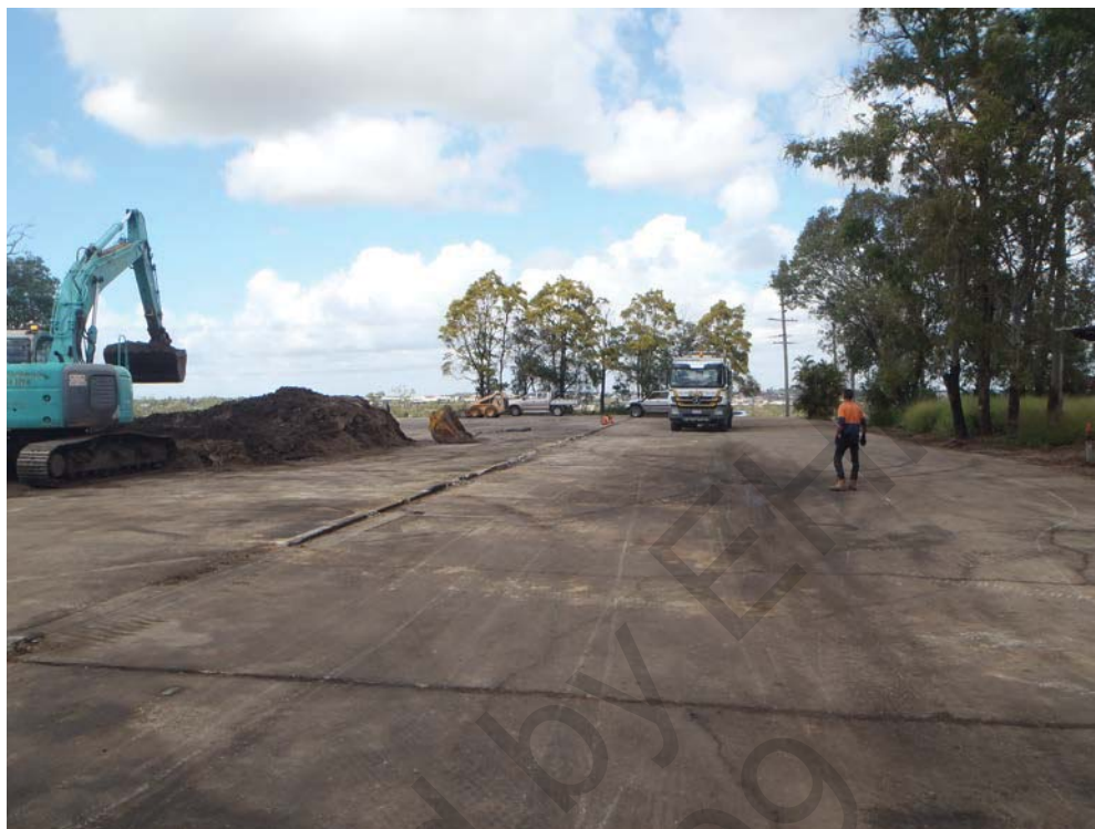
Photo 2 – Photo taken looking south from the potassium street entrance gate at the top of the property. Note The liquid waste truck at the rear of the photo. This truck was being used to clean the out the stormwater drainage systems in order for the system to be re-opened.
