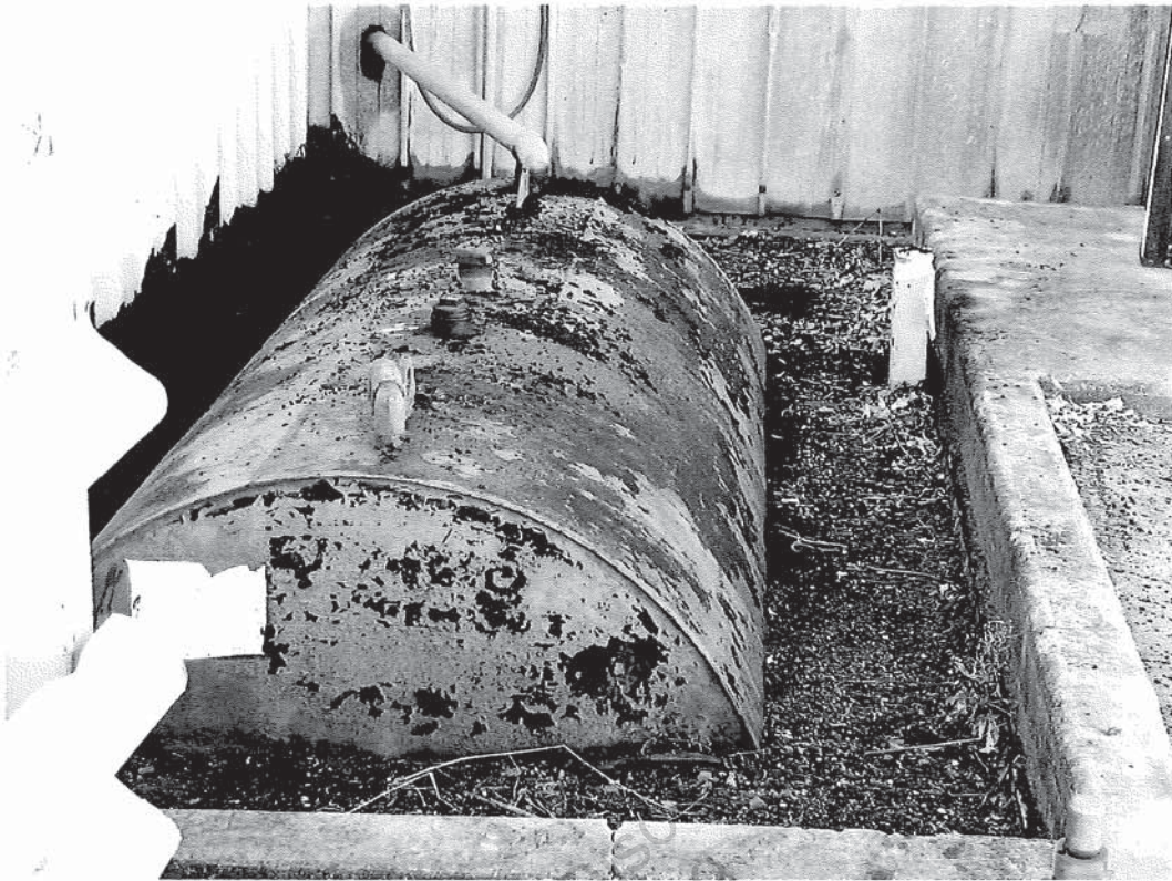
Photo 13 – A semi submerged tank on the west side of the motor vehicle workshop. It is used to collect waste oil. The tank has not been integrity tested.
