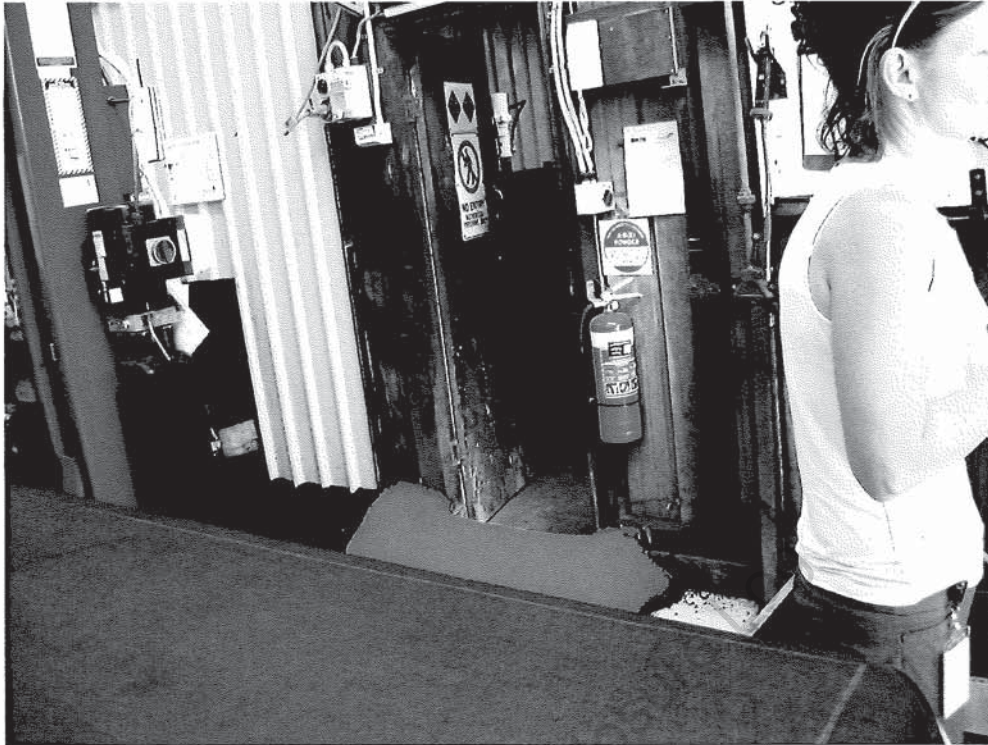
Photo 27 – The bunding situated at the door of the chemical storage room. The bunding has been painted red for safety reasons.
