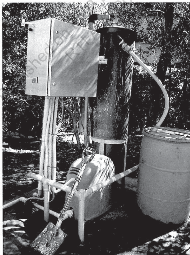
Photo 8 – The wastewater separator situated behind the main wash bay.
