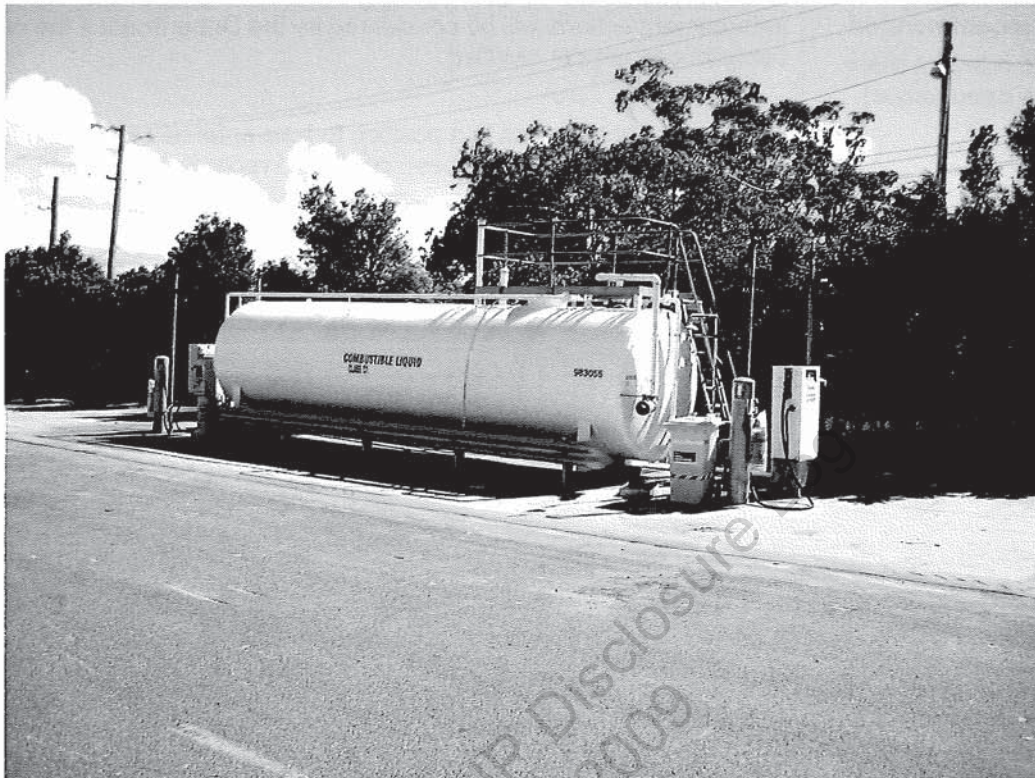
Photo 1 – Large diesel storage tank situated on the northern boundary (parallel to Jull Street) of the property and adjacent to the depot entry. WHS have been contacted regarding the suitability of the bunding.
