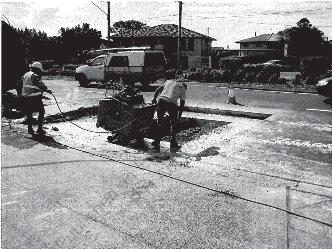
Figure 3. Photograph looking eastward over the incident location.
