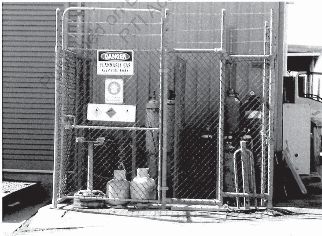
Photo 16 – Flammable gas storage opposite the green waste stock piles.
