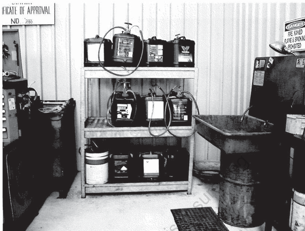
Photo 23 – Motor vehicle oil cleaning and disposal area inside the workshop. The oil containers are stored on a bunded stand.
