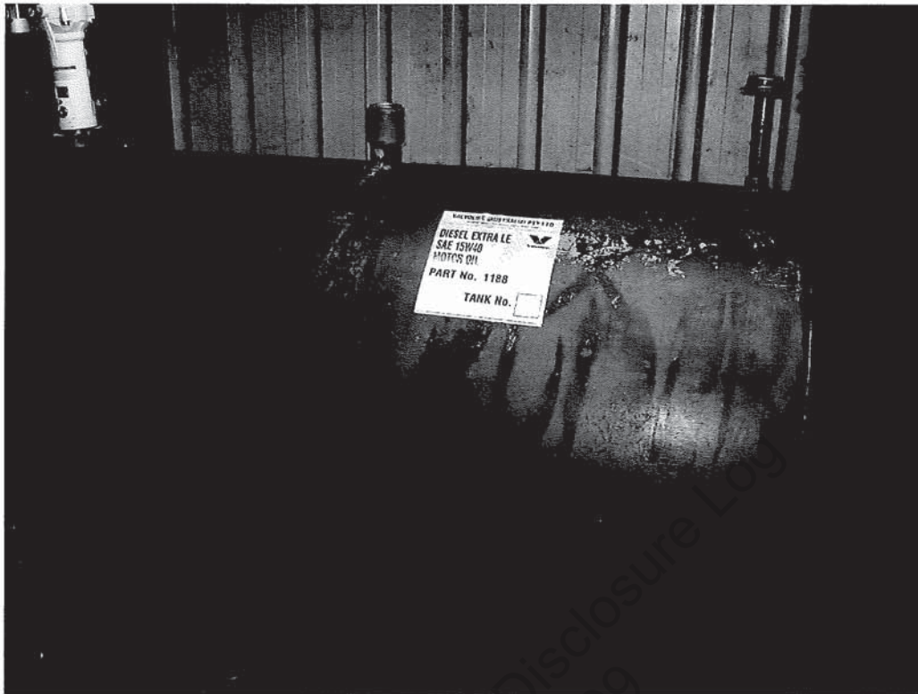
Photo 25 – Diesel storage tank on the southern wall. This tank is the largest in the chemical storage room.
