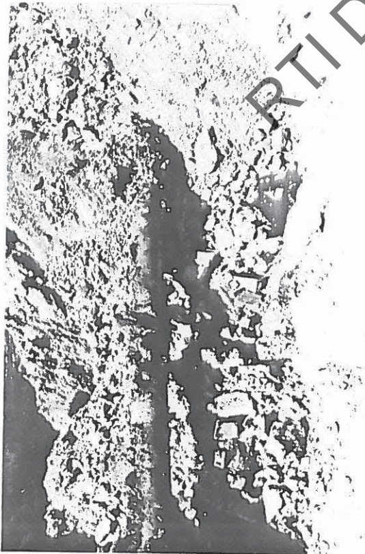
Photograph 1 View showing damaged oil pipeline with oil in excavation.
