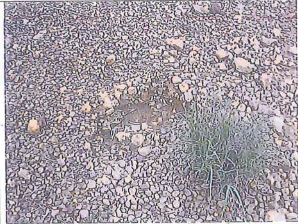
Figure 15- Sinkhole developing with lateritic gravels
