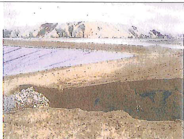
Figure 2- Sink hole adjacent to stormwater pond 2.
