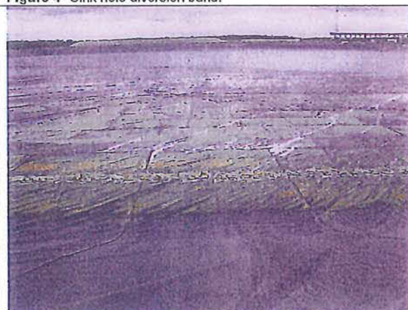
Figure 6- Possible leaks in stormwater pond 2.
