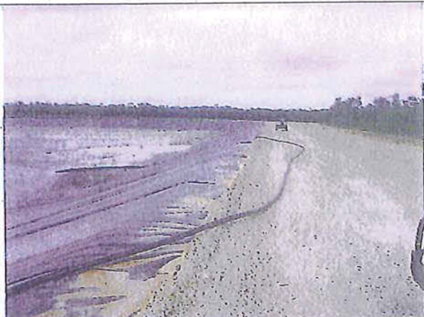
Figure 9- Mobile pump and leak detection bore
