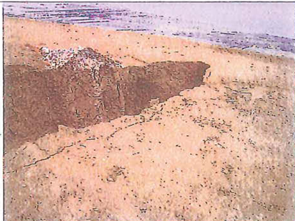
Figure 3- Sink hole adjacent to stormwater pond 2.
