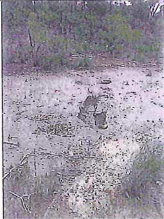
Figure 16- Sinkholes forming on recently disturbed road for sterilization drilling
