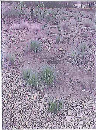
Figure 14- Lateritic gravel with evidence of sinkholes
