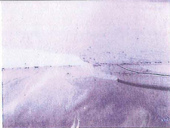
Figure 10- Pipe discharging waters from underneath pond 2 liner.
