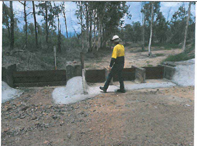
DSCN1930. Levee Bank overflow
