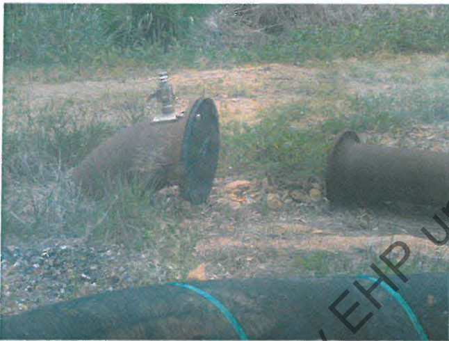
DSCN1925. Closed off ocean outfall pipe
