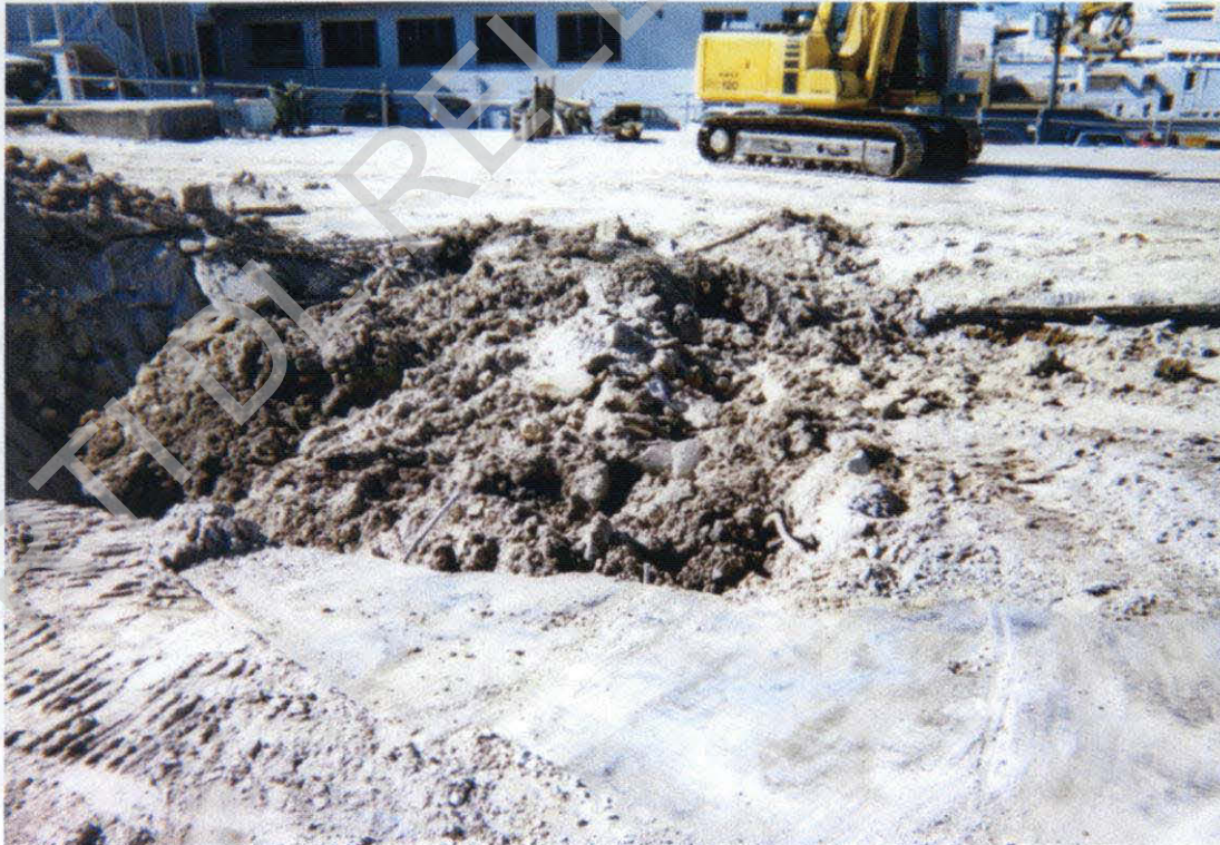
Plate 14: Excavated material from waste oil pit was reinstated in the excavation. This was not a recommendation of PPK. This pit cannot be deemed validated.
