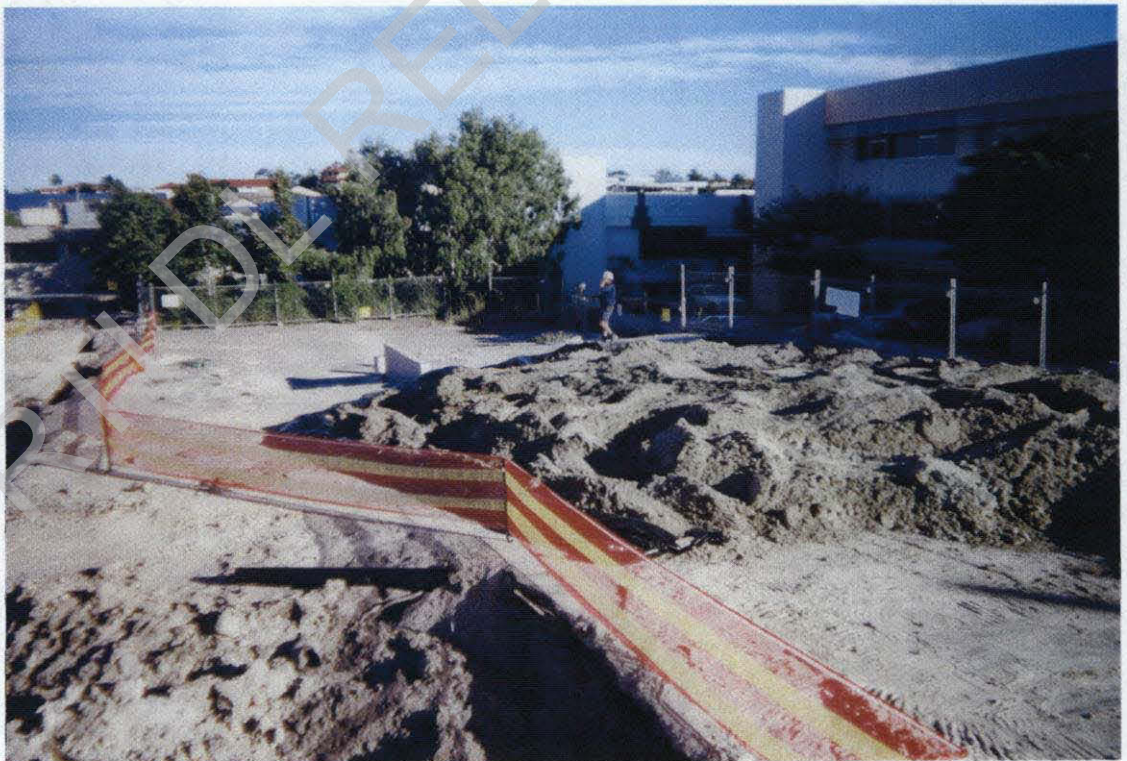
Plate 16: Photo of potentially contaminated, stockpiled soils. Note that stockpile is on plastic sheeting and a 'sausage' bund employed on the lower-elevation edge.
