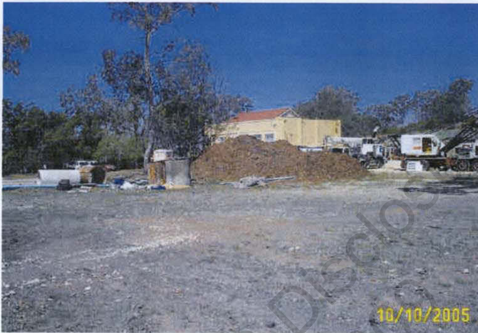
Photo 3: Stockpile of mulch and piles of construction and demolition material on Lot 5 looking south.
