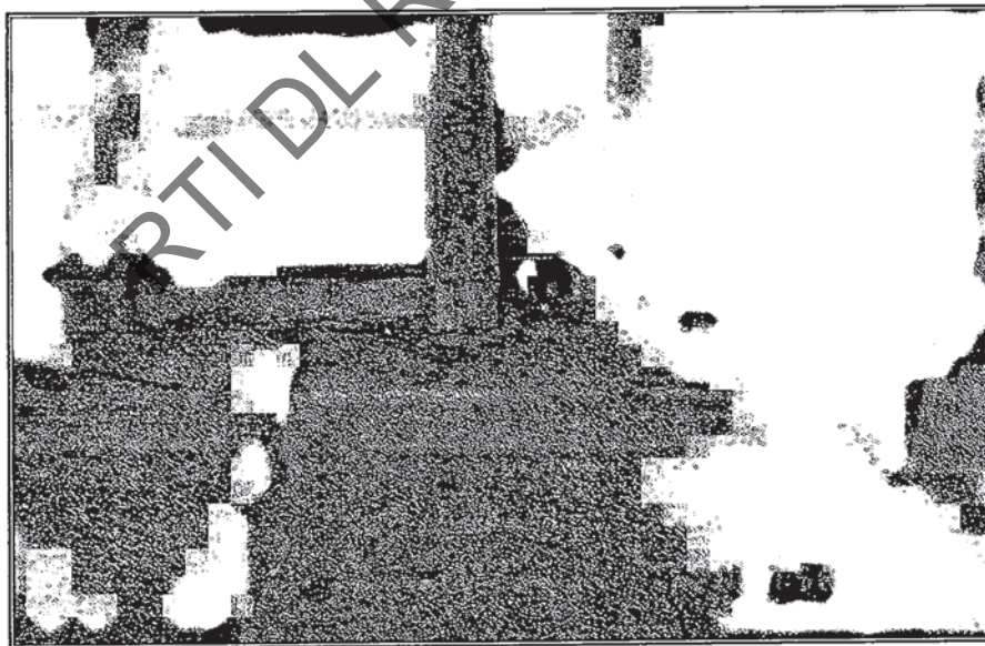
Photo 8 : Asbestos cement debris scattered over floor of south / east and south / west decks, Second Floor.
