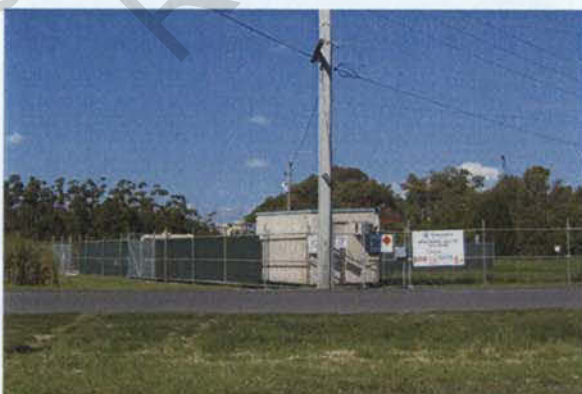
Figure 15: "Gate station" east of the site
