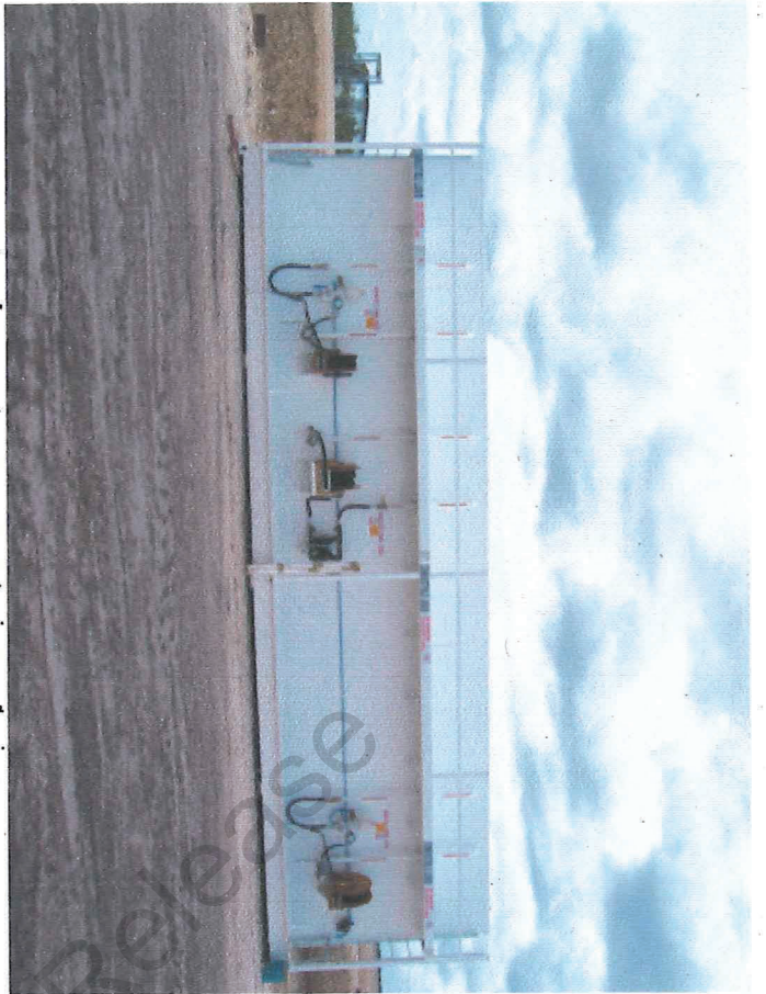
petroleum storage container 1.jpg
