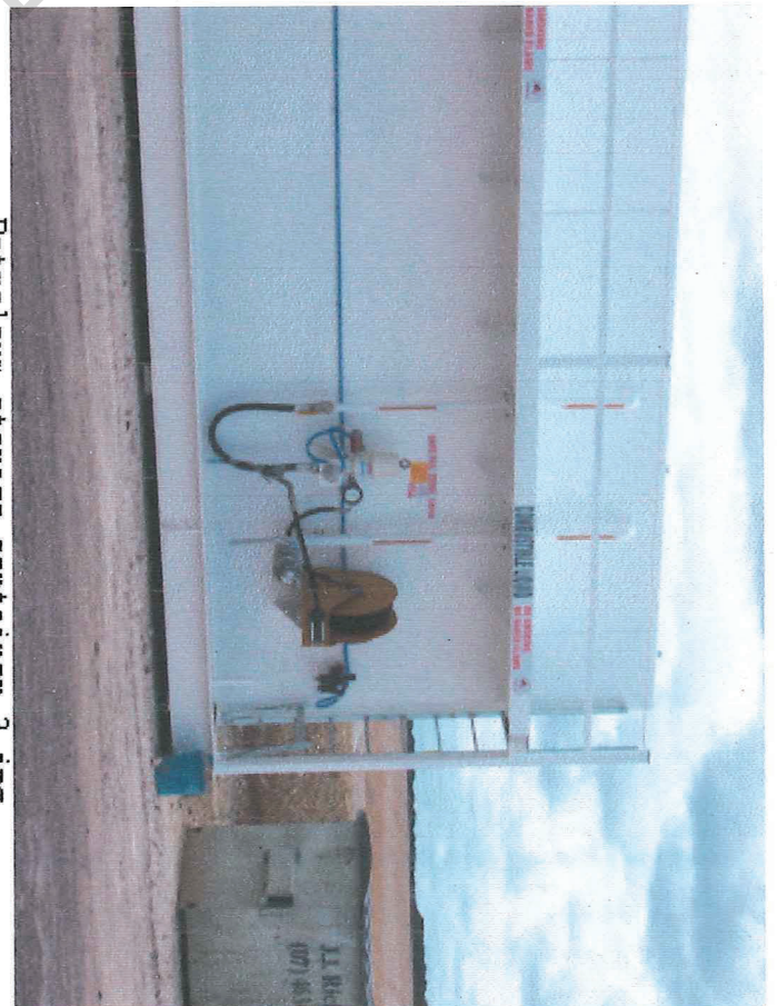
Petroleum storage container 2.jpg
