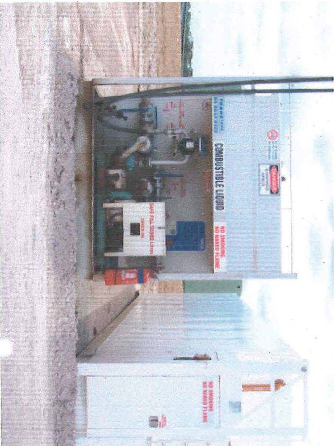
combustable liquid storage.jpg
