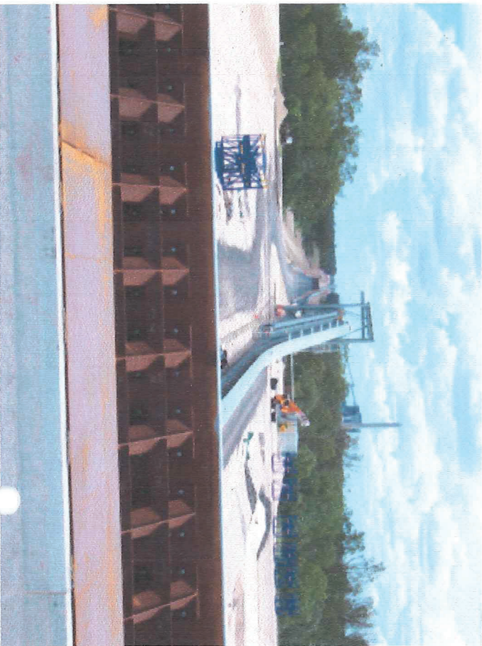
coal hopper and conveyor.jpg
