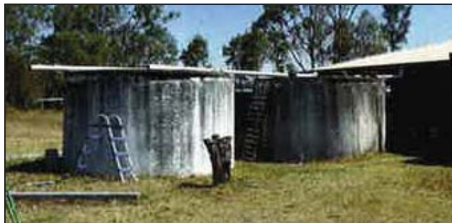
Figure 4. Concrete Tanks that supply water to the internal taps.
