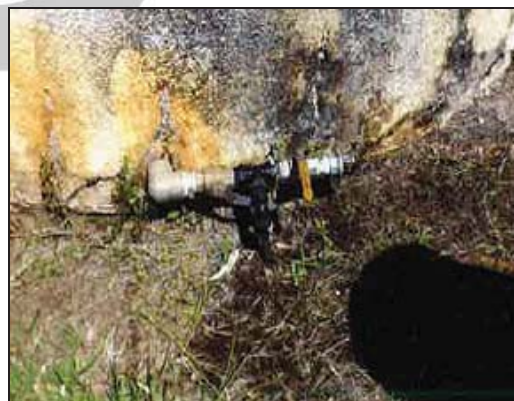
Figure 7. Concrete water tank tap, sample was collected.
