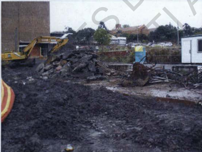
Photo 6 - C and D waste looking north to rear of site.
