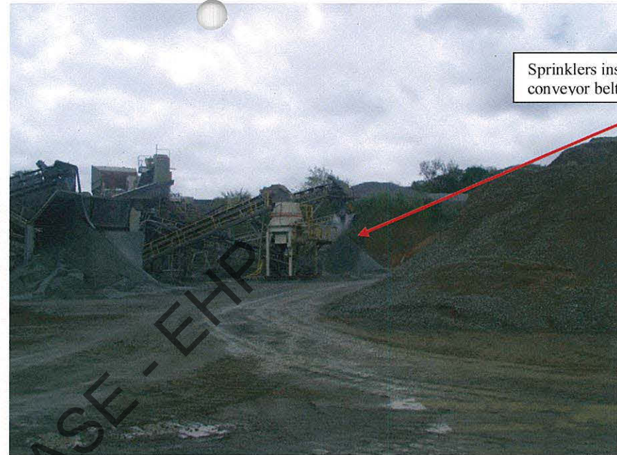
Photo 3: Shows the sprinkler system installed on the screening equipment.
