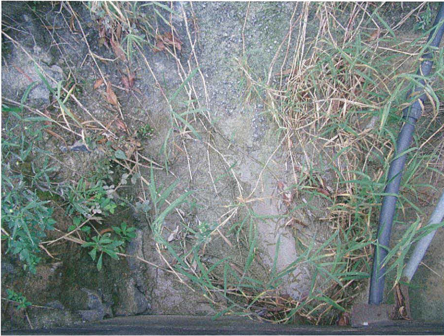
Photo 5: Shows sediment leaving the site under the road
