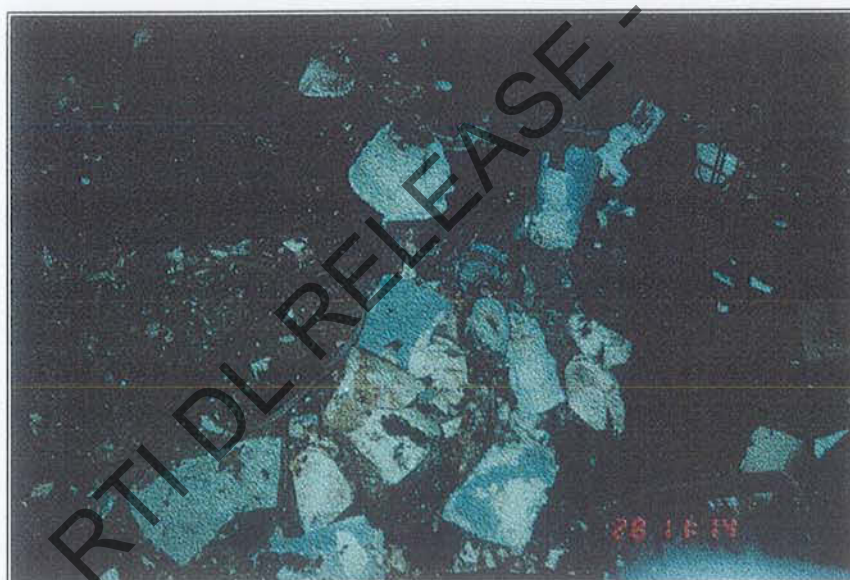
Photo 6 : Asbestos insulation debris in Switch Room, Level 1.
