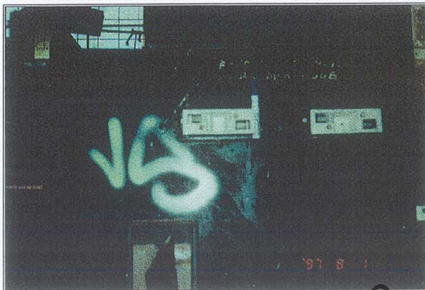
Photo 5 : Asbestos insulation in the electrical fuse socket in the Switch Room, Level 1.
