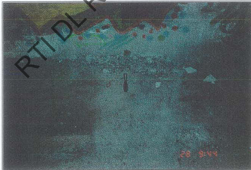
Photo 4 : Asbestos insulation debris on floor against northern wall, Level 1.
