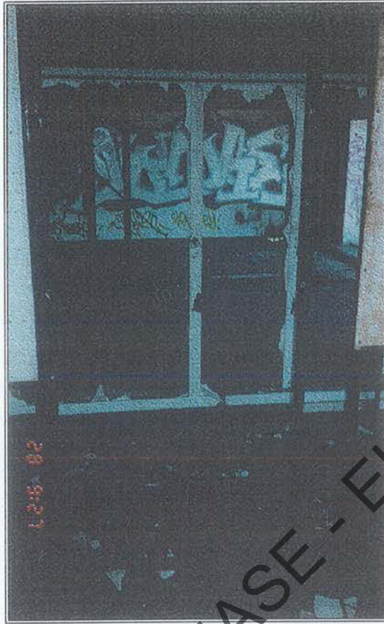
Photo 7 : Damaged asbestos cement wall sheeting, Level 2.
