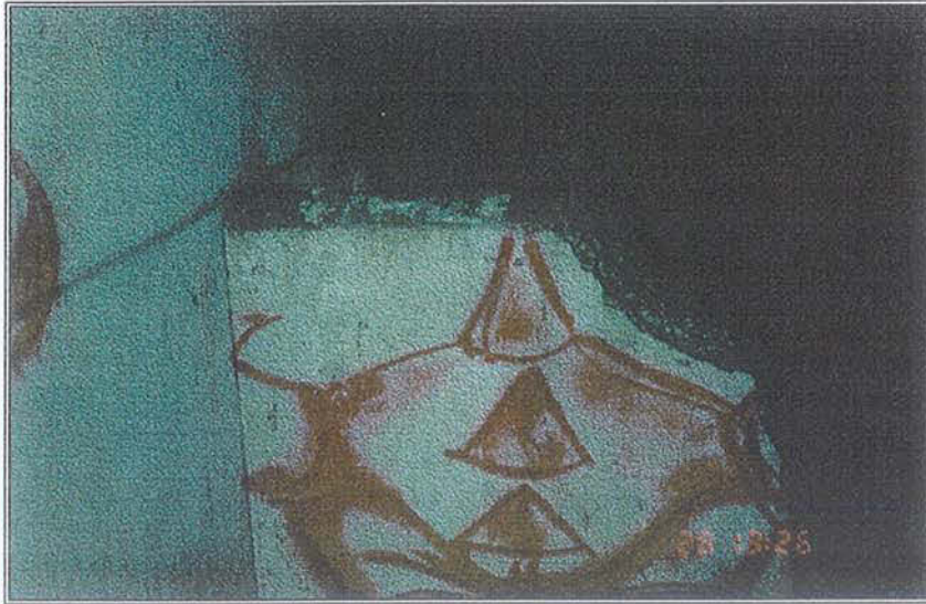
Photo 1 : Asbestos insulation debris on top of concrete plinth, Ground Floor.
