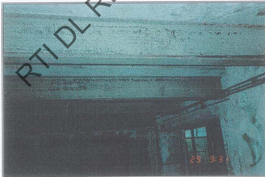
Photo 12 : Silver lead based paint on horizontal structural steel beams, Level 2.
