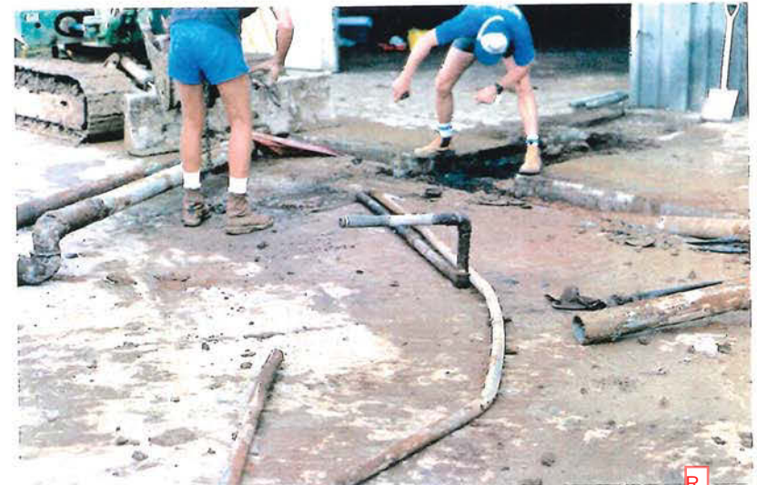
Excavated pipework in the area between the pump and the drum: note the black oil staining of the soil. The pump was located at the top right corner to the left of the shovel. The grating covering the drain can be seen immediately to the right of the person on the left.
