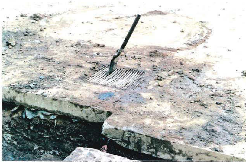
Oil stained soil in the vicinity of the drain.
