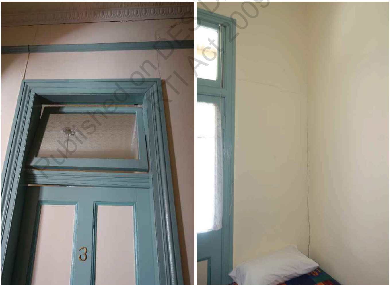
Image 23a (left) an image of the door to room 3 with racks and misalignment Image 23b (right) The interior of a room showing a vertical crack in the corner and horizontal crack between the window and corner. (DES, 23 August 2019.)
