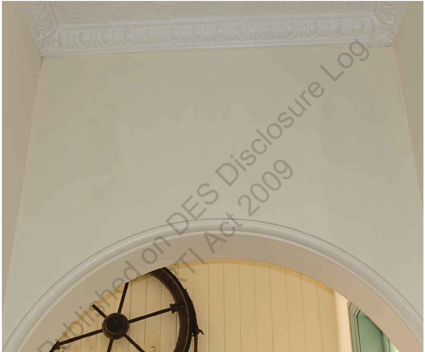
Image 26: A fine crack mid archway behind the upstairs coffee room - the pulley and rope mechanism for the food lift was part of the original design and is visible and intact (DES, 23 August 2019).
