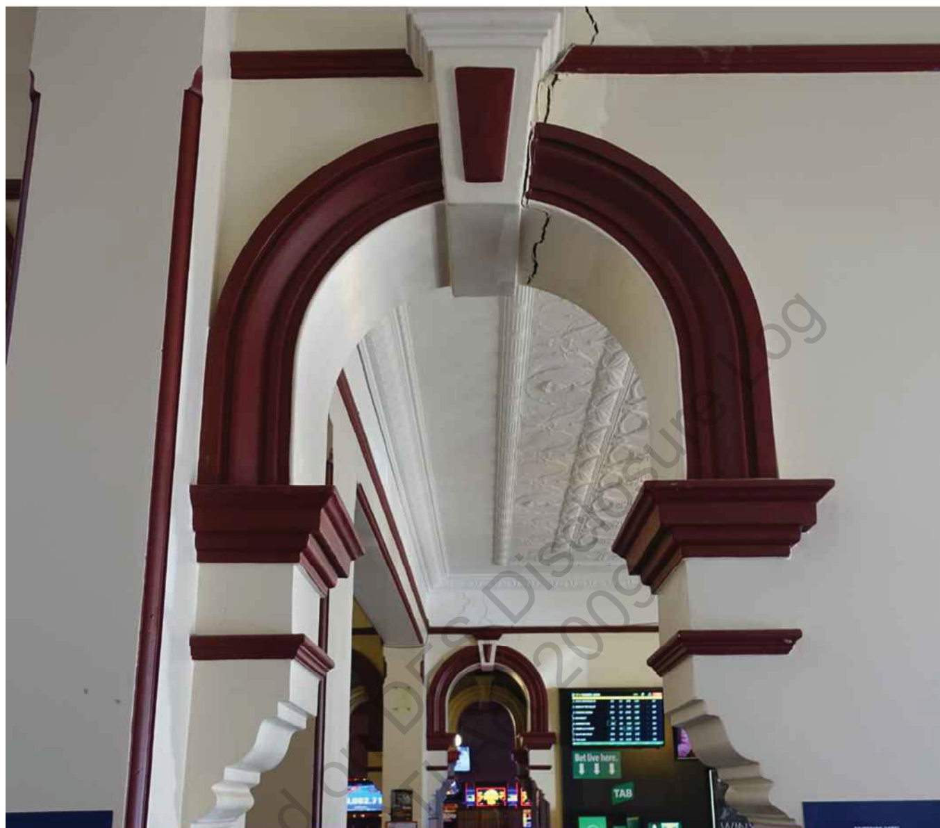
Image 12: An image showing the alignment of cracks in the archways from the billiard room to the public bar to the lobby located in the front section of the Criterion Hotel to the west of the main structural beam (DES, 23 August 2019).
