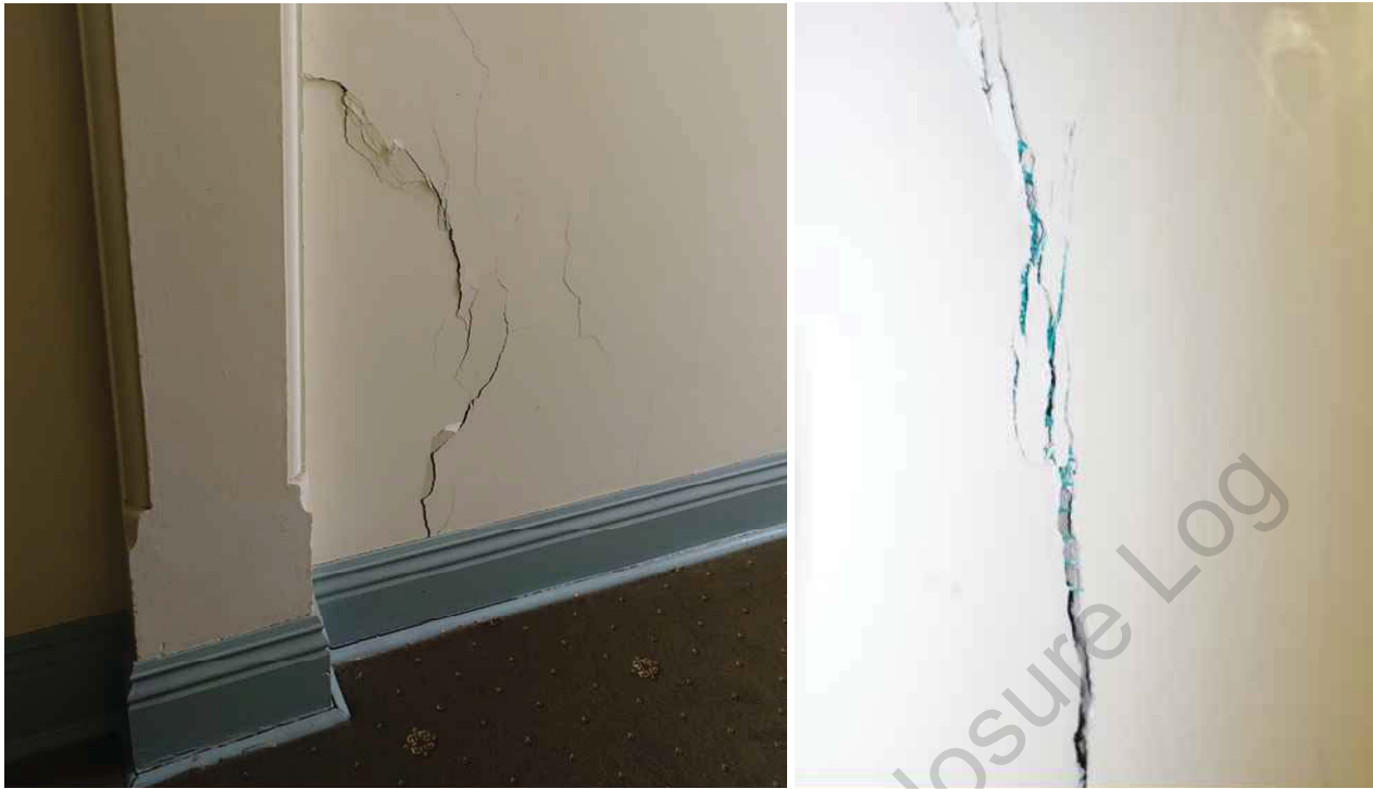
Image 24a (left) cracking in the northern end of the upstairs wall and Image 24b (right) a close-up image of the cracks showing metal mesh in the plasterwork and render underneath (DES, 23 August 2019).
