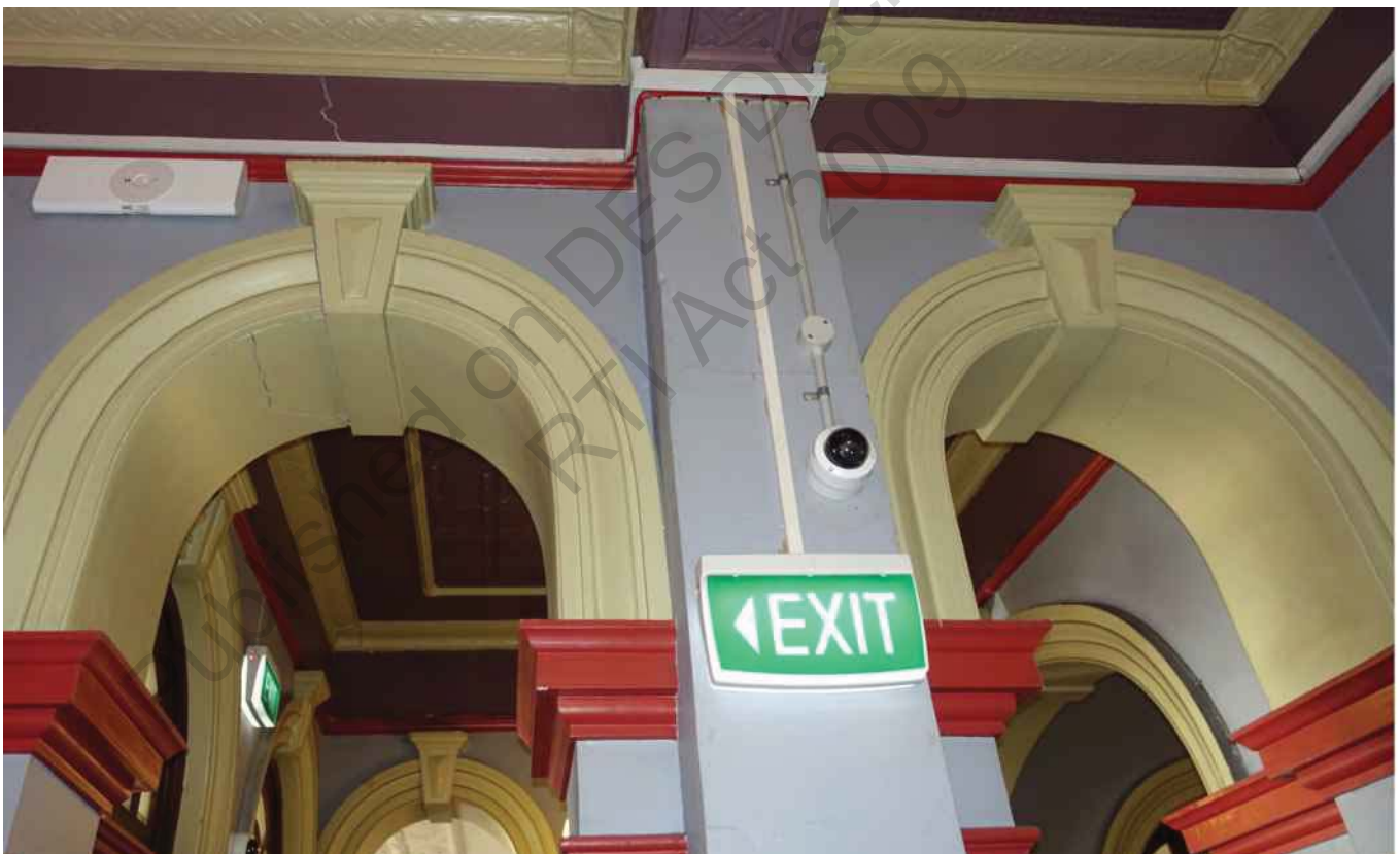
Image 9: Cracks in the underside of both archways and above the keystones in the walls leading from the gaming lounge back to lobby (DES, 23 August 2019).
