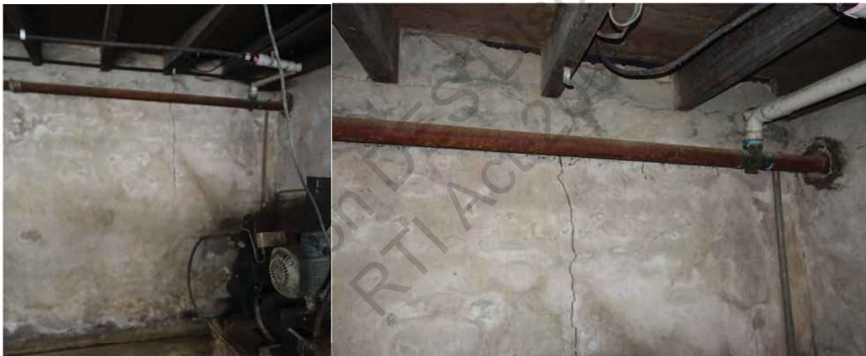
Images 16a (left) and 16b (right): showing the crack on the northern wall (DES, 23 August 2019).
