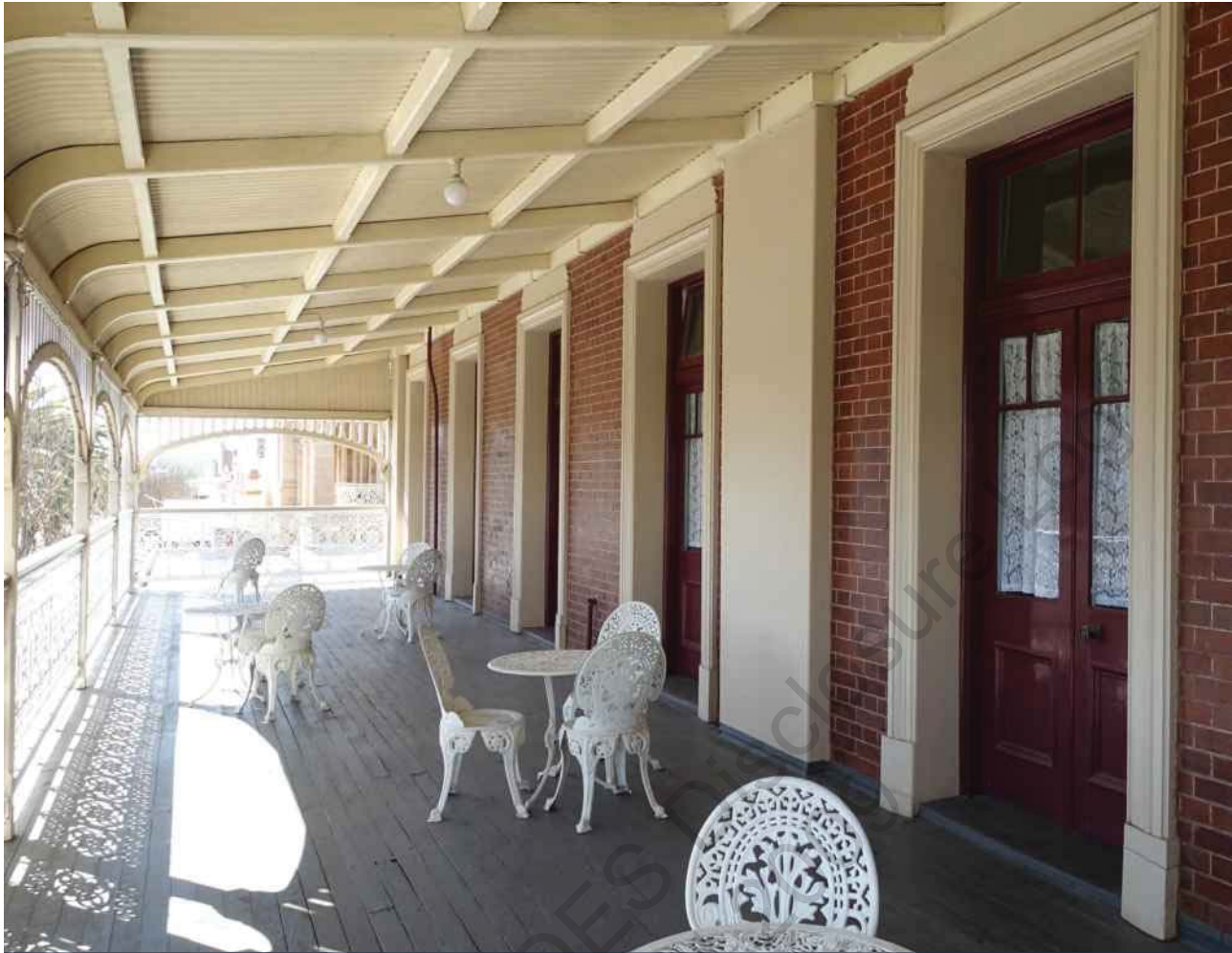
Image 27: A view north along the verandah - some cracks are evident in the base of some door frames (DES, 23 August 2019).
