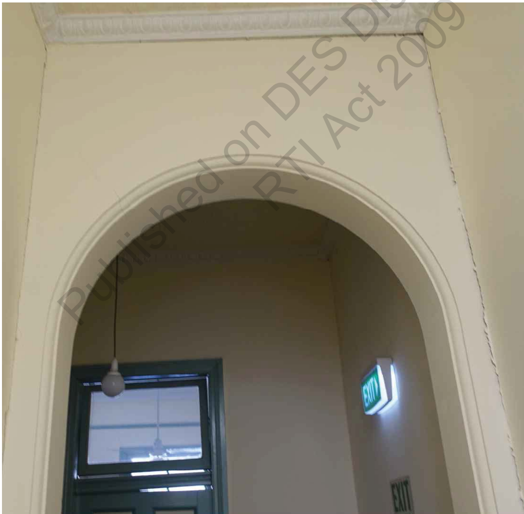
Image 25. Looking west toward room 1 on the first floor - note the cracking above the arch, along the wall joints and delaminating of the architrave. The door and fan light to room one behind are also misaligned. (DES, 23 August 2019.)
