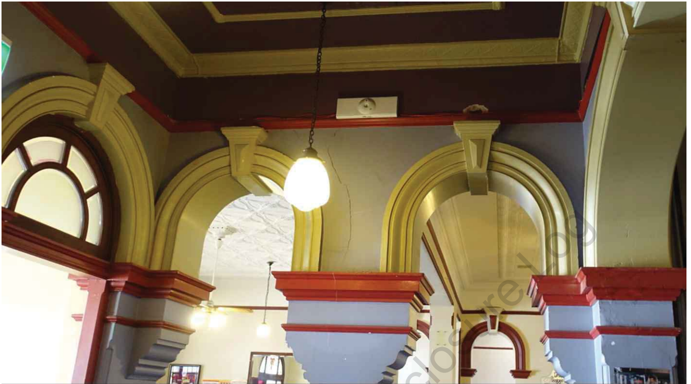
Image 10: The lobby leading into the public bar. The supporting columns and associated walls have clear vertical cracking along the wall and into the column (DES, 23 August 2019).
