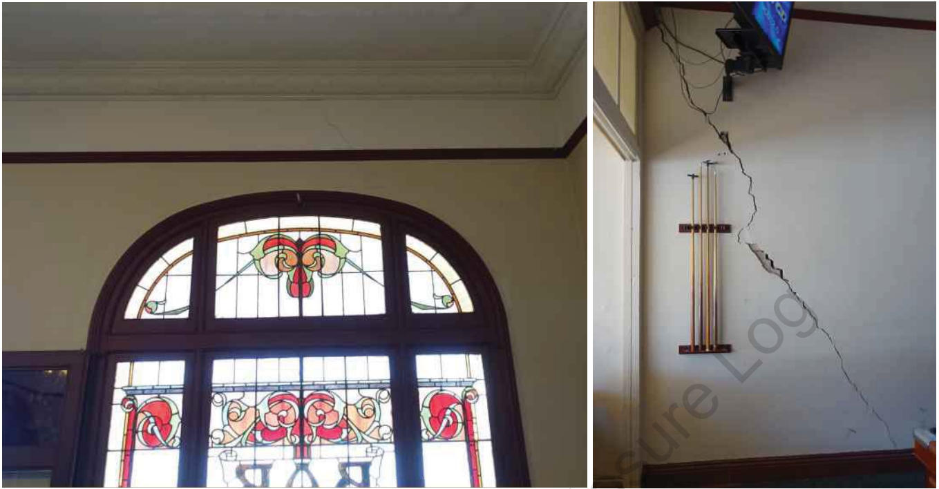
Image 6a (left): A fine crack above the stain glass window of the public bar facing Palmerin Street (DES, 23 August 2019).
