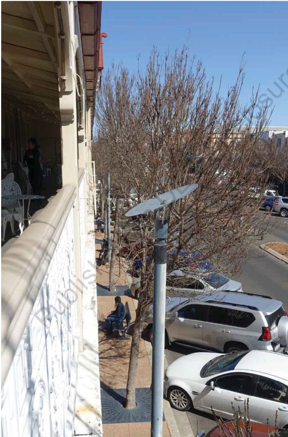
Image 34: Looking south along Palmerin Street - note the proximity of the trees to the verandah guttering and balustrade posts and associated downpipes (DES, 23 August 2019).
