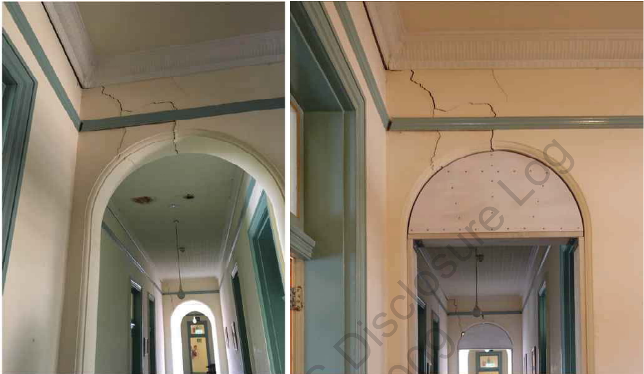
Images 20a (left) an image from the engineers report and 20b the same location with stabilisation works. Note the rust on the pressed metal ceiling in 20a. (DES, 23 August 2019.)
