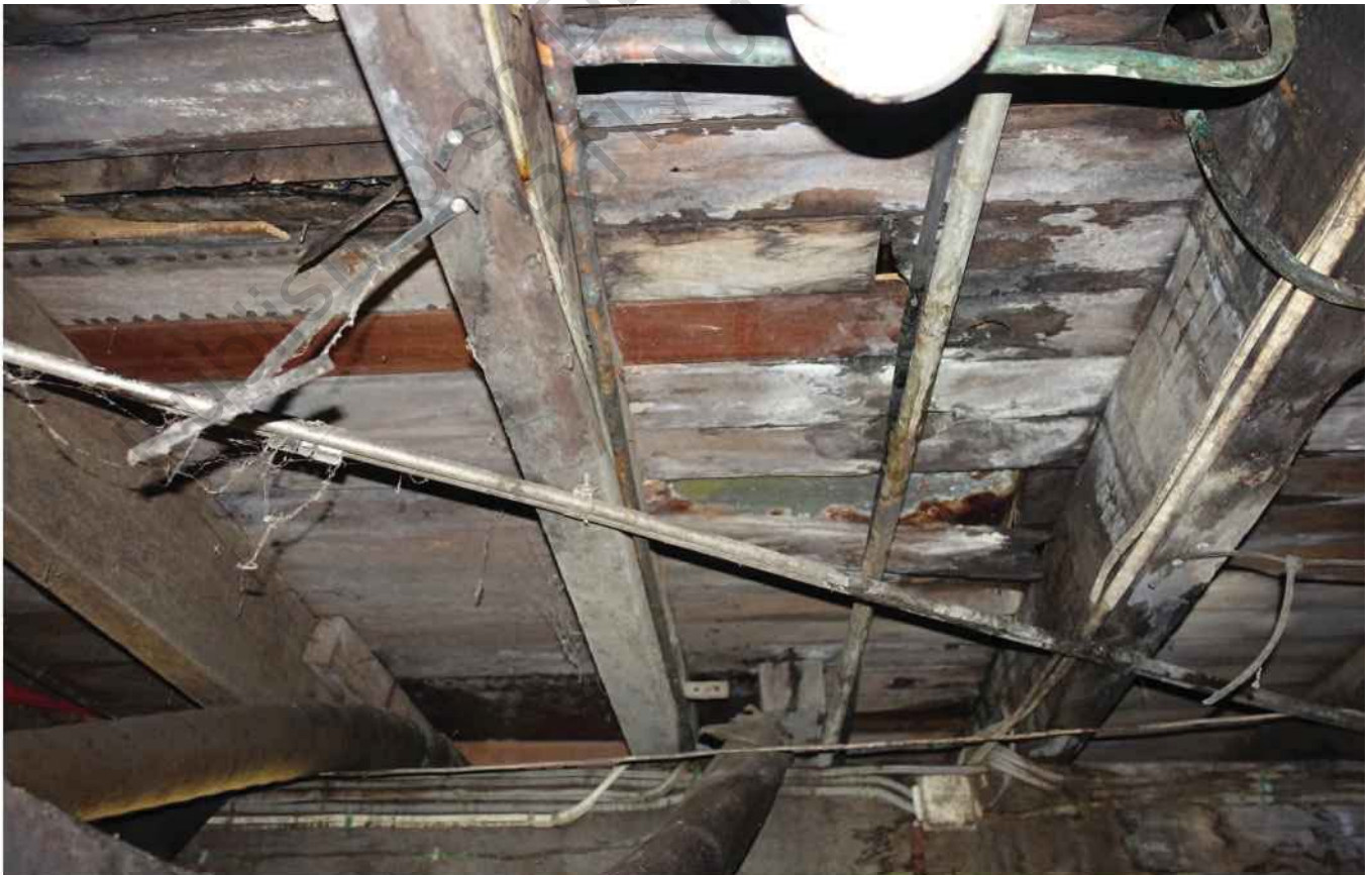
Image 19: The rotten and damaged floor boards in the wine and spirit store located directly under the bar (DES, 23 August 2019).
