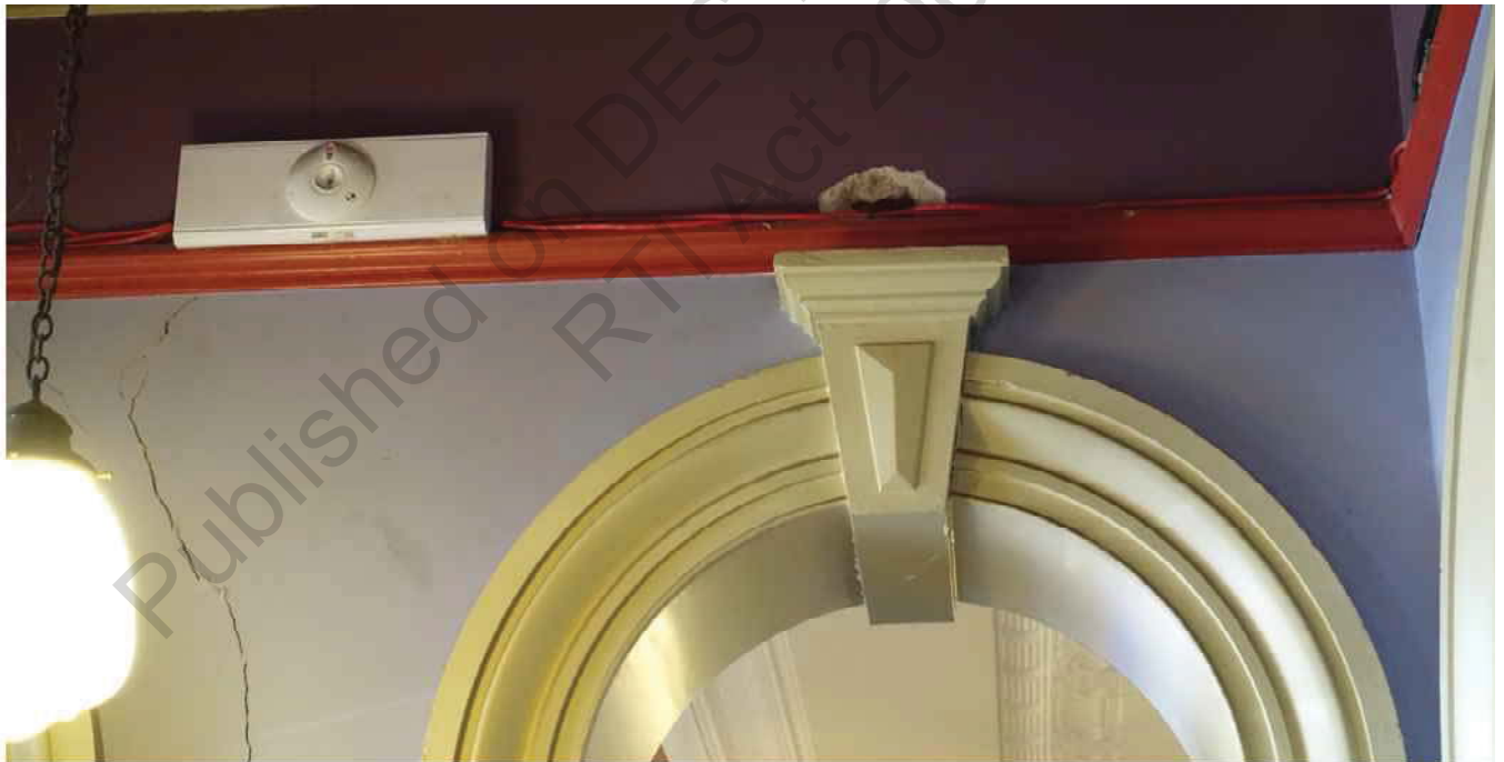
Image 11: A close-up of the crack in the column and the missing render above the keystone leading from the lobby to the public bar (DES, 23 August 2019).
