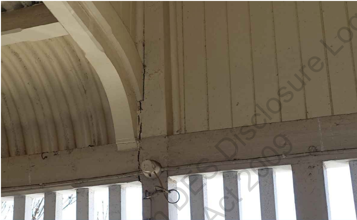
Image 31: A vertical crack in the timber frame located in the centre section of the verandah roof - located directly outside the sitting room (DES, 23 August 2019).
