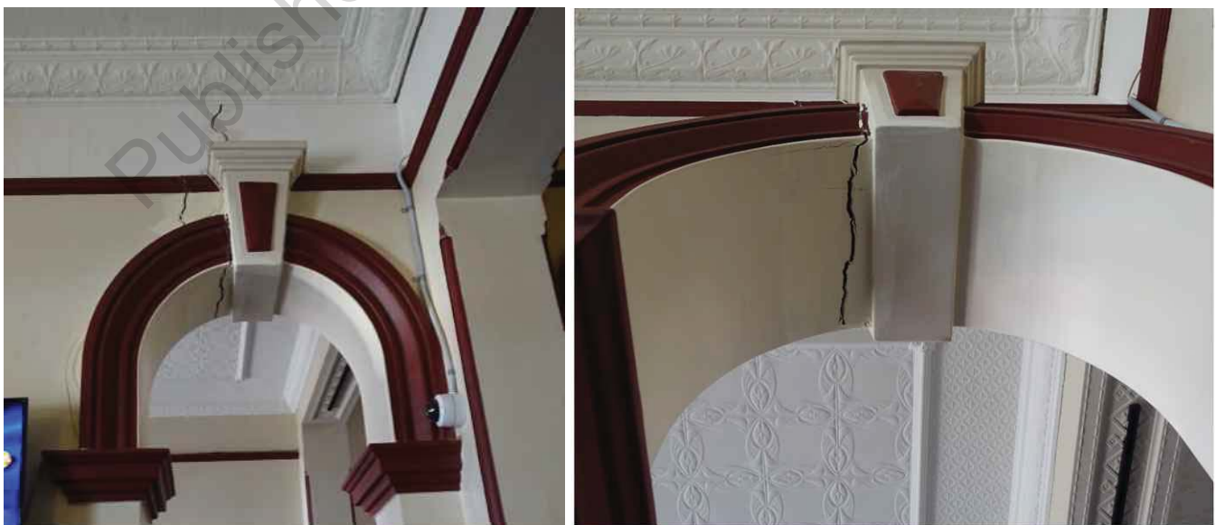
Images 5a (left) and 5b (right): A pronounced crack around the keystone of the archway heading north out of the public bar into the billiard room. (DES, 23 August 2019.)
