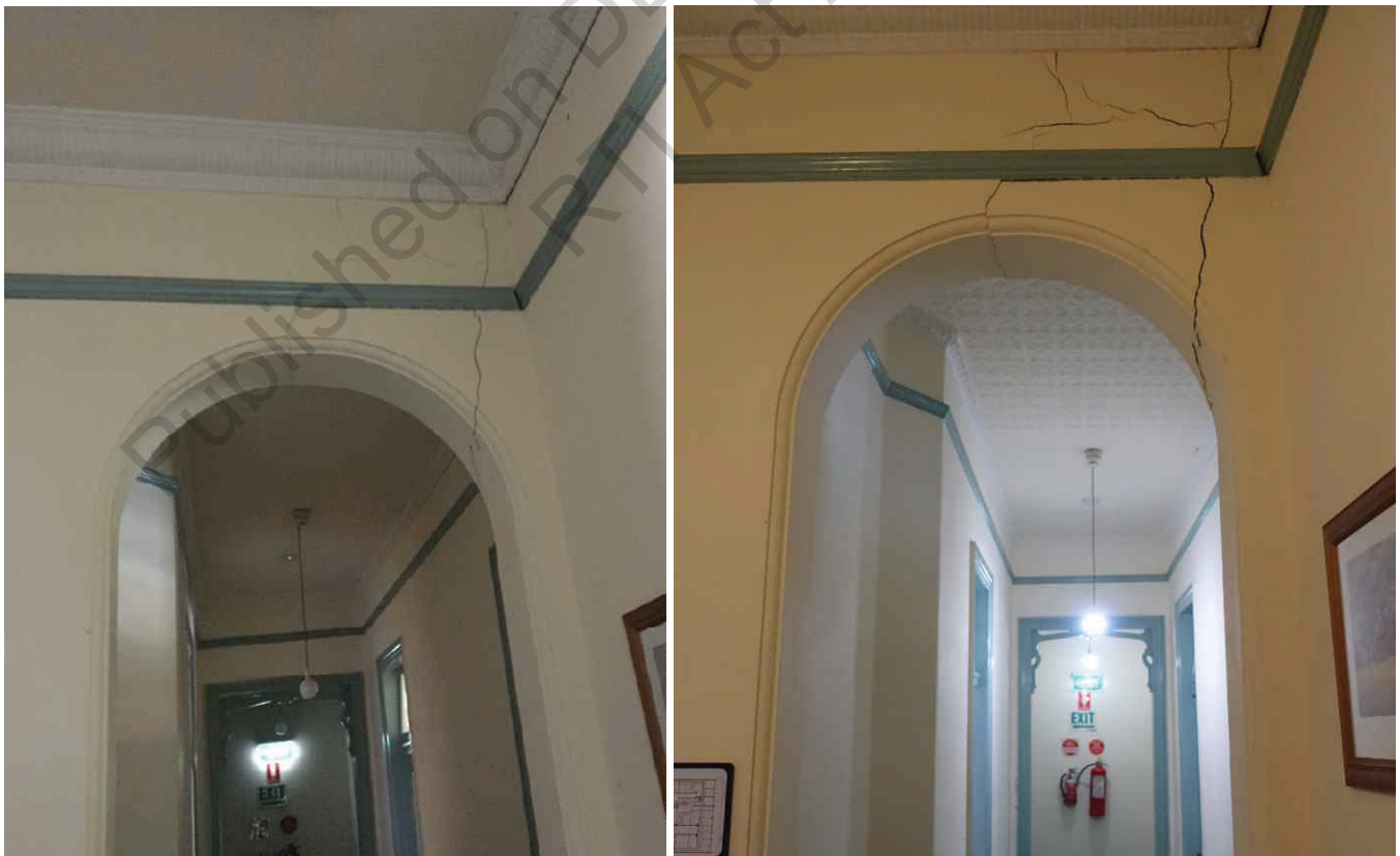
Images 21a (left) an image from the engineers report and 21b (right) the same location during the site visit. The cracks do visually appear to be more pronounced in the later images. (DES, 23 August 2019.)
