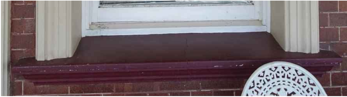
Image 30: A vertical crack in the sill of the verandah window to bed 8 (DES, 23 August 2019).
