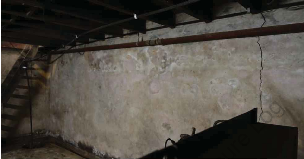
Image 15: The northern wall of the basement showing the proximity of the crack relative to the cellar access hatch and sump. Note the clear evidence of water staining and efflorescence, especially in the lower portions of the wall immediately above the spoon drain (DES, 23 August 2019).
