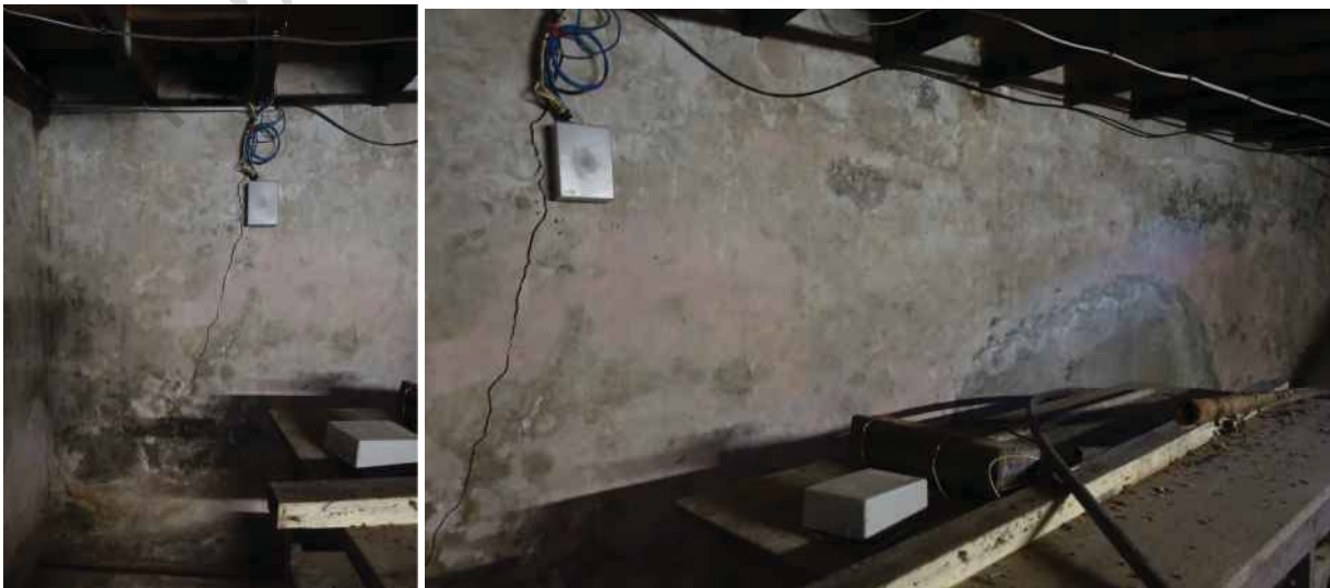
Images 17a (left) and 17b (right): showing the crack on the southern wall (DES, 23 August 2019).
