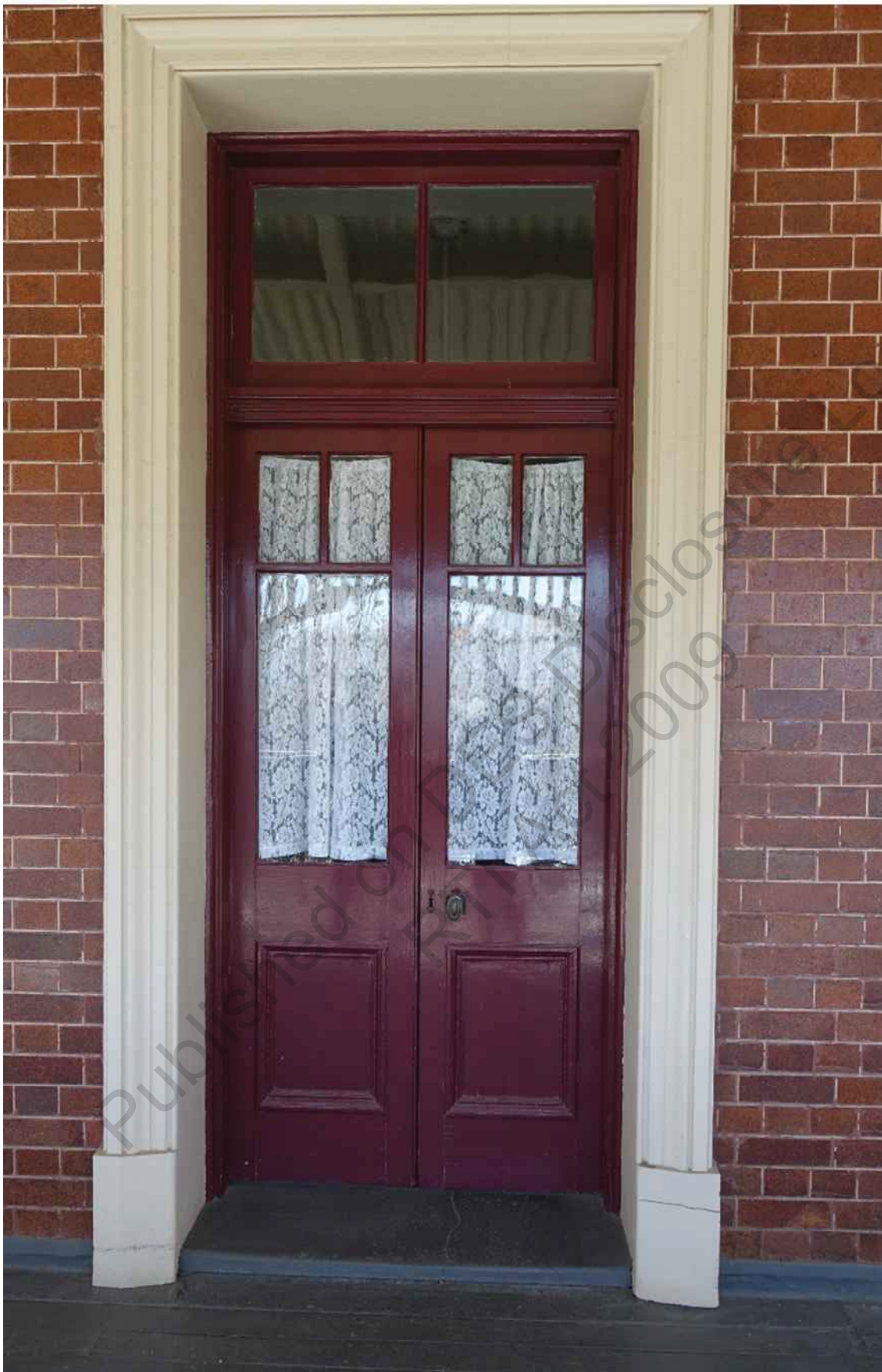
Image 29: Verandah French doors located in bed 5 showing horizontal cracks at the architrave plinth on both sides of the door frame - the left crack has paint applied, the right crack is open. The exterior moulded rendered door architrave otherwise appears to be sound condition. There is also a vertical crack through the tread between the frames but this does not appear to be recent. (DES, 23 August 2019.)
