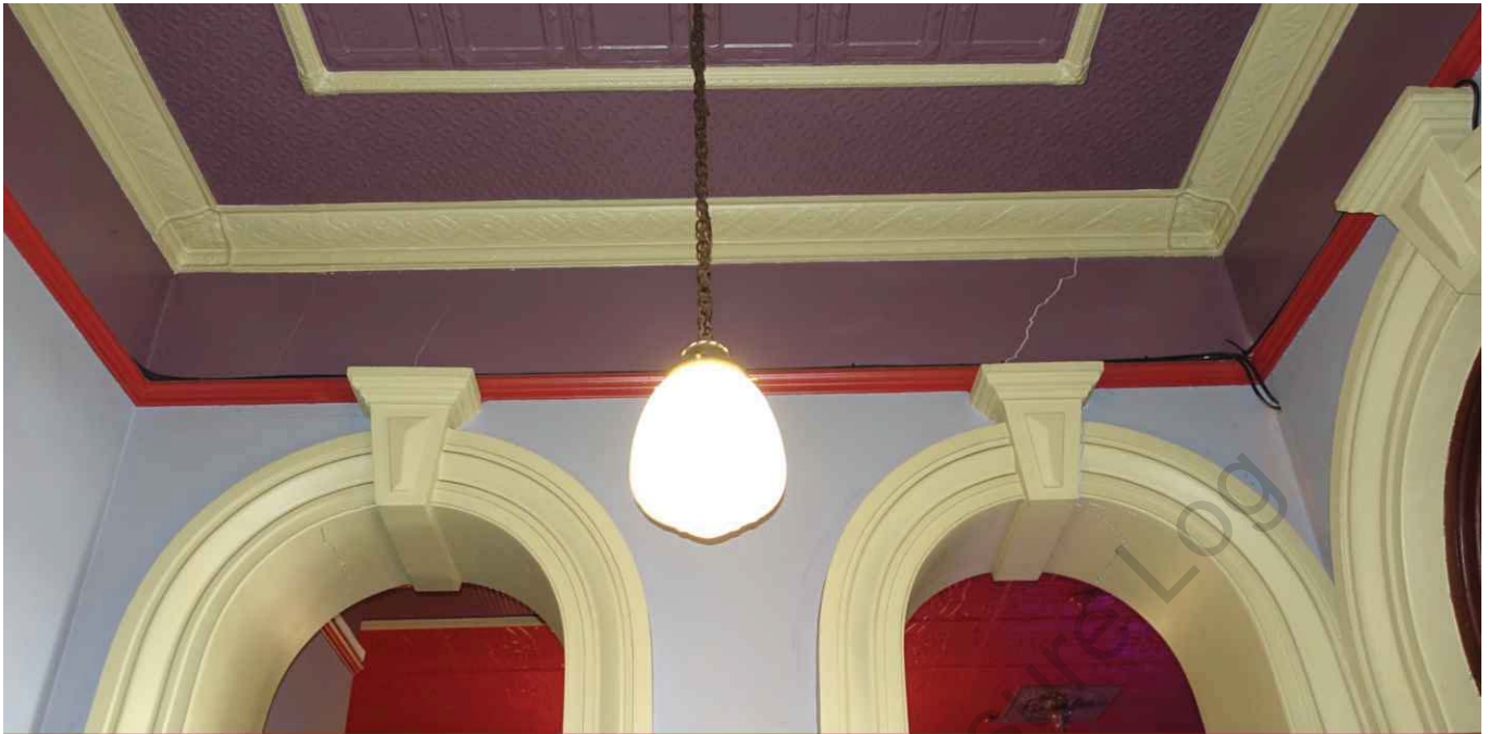
Image 8: Cracks in the underside of both archways and above the keystones in the walls leading from the lobby through to the gaming lounge (DES, 23 August 2019).
