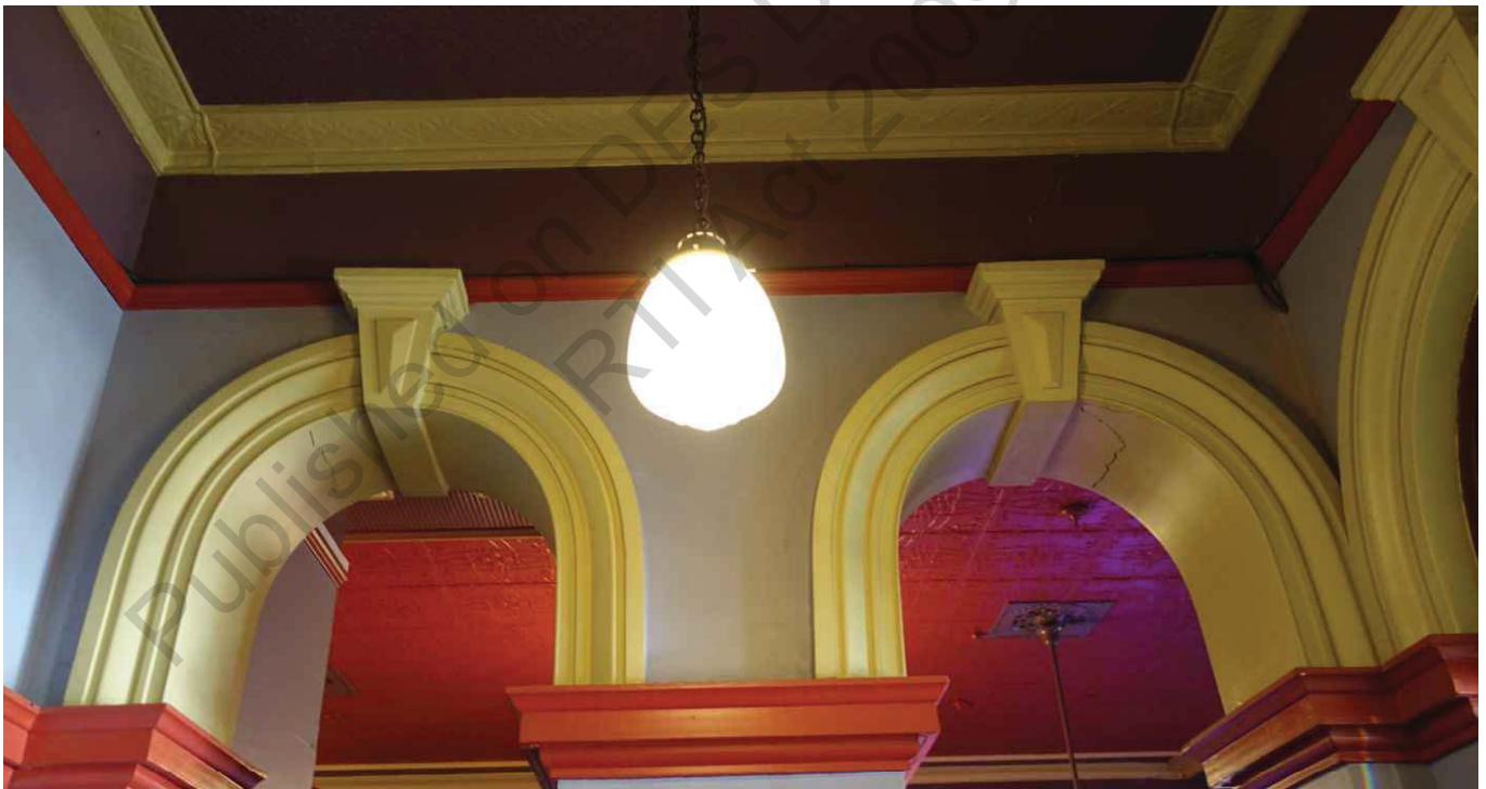
Image 7: Cracks in the underside of both archways leading from the lobby through to the gaming lounge (DES, 23 August 2019).
