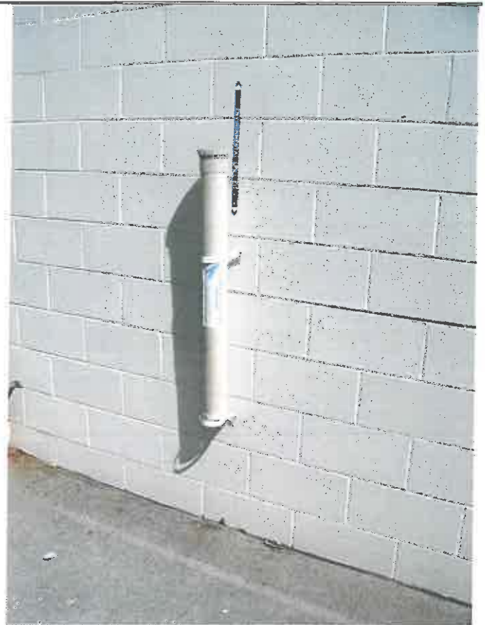
Photograph 15 – A strategically wall-located spill kit containing a gully trap-sealing mat positioned adjacent to the bunded installation shown in Photograph 14.
