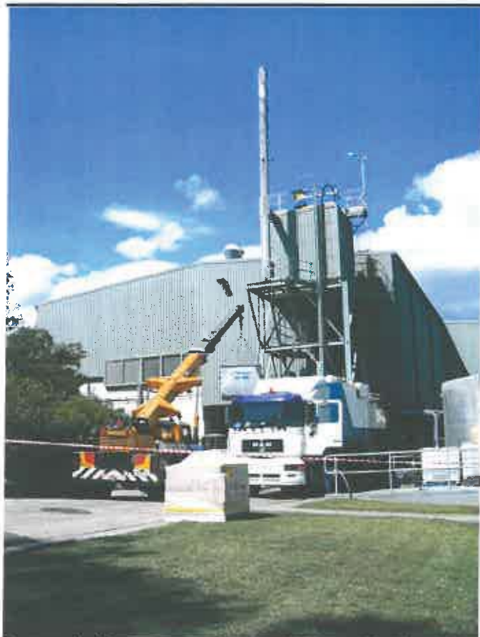
Photograph 16 – On the day of the formal site inspection, the gelatine processing plant was temporarily shutdown to allow cleaning of ash from the Finafire Boiler Baghouse and replacement of the filter bag set.
