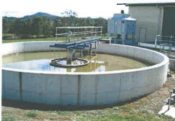
Photograph 20 – The treated wastewater overtopping the Clarifier Tank weir to the transfer trough to the Balancing Storage Dam was noted to be essentially translucent, light brown in colour and demonstrating a minor odour profile.
