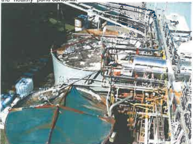
Photograph 23 – Biological digestion tanks for the acid and alkaline sludges emanating from the hides/facepieces cleaning tanks, prior to gelatine extraction operations.
