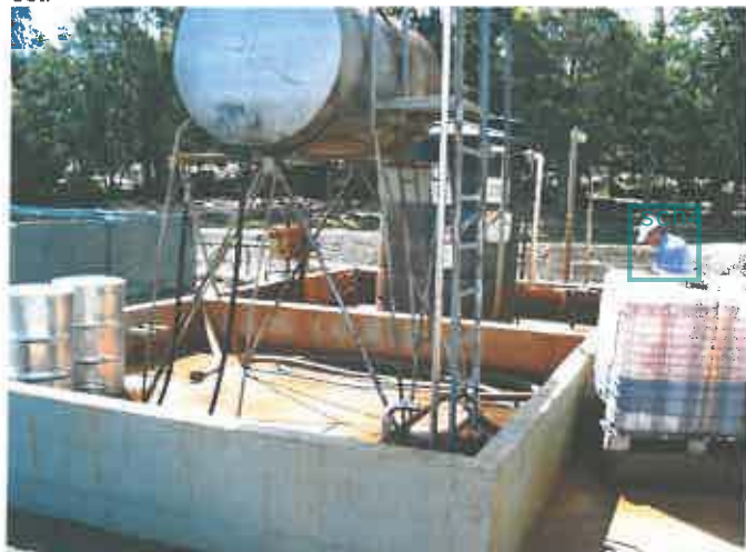
Photograph 17 – New above-ground diesel fuel (farm tractors, mechanical bucket fuel servicing) storage tank containment bund.
