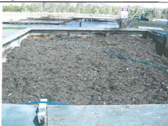
Photograph 18 – The Hybractor effluent treatment plant foul gas "Ferric" Biofilter unit showing new media fill, replaced on 13-14/10/2005. Only minor local fugitive odour was noted in the immediate surrounds to this installation and the adjacent supply fan.
