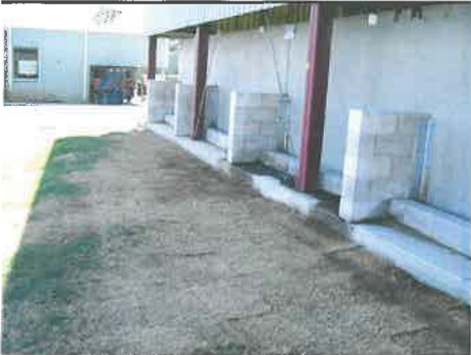
Photograph 13 – Effects of slow brine seepage from stockpiled salted hide material, through floor/wall junction, sealing of which is to be addressed during the 2005/2006 plant shutdown period.
