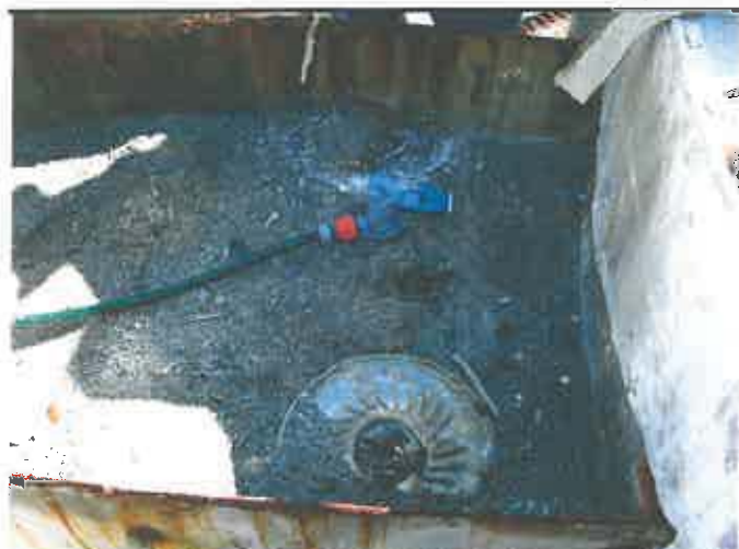
Photograph 21 – Temporary "mini make-shift" Biofilter arrangement is in place as an effective, short-term odour control measure for a slow odorous leak from the Primary Digester Unit, until repairs requiring a major plant shutdown can be effected.
