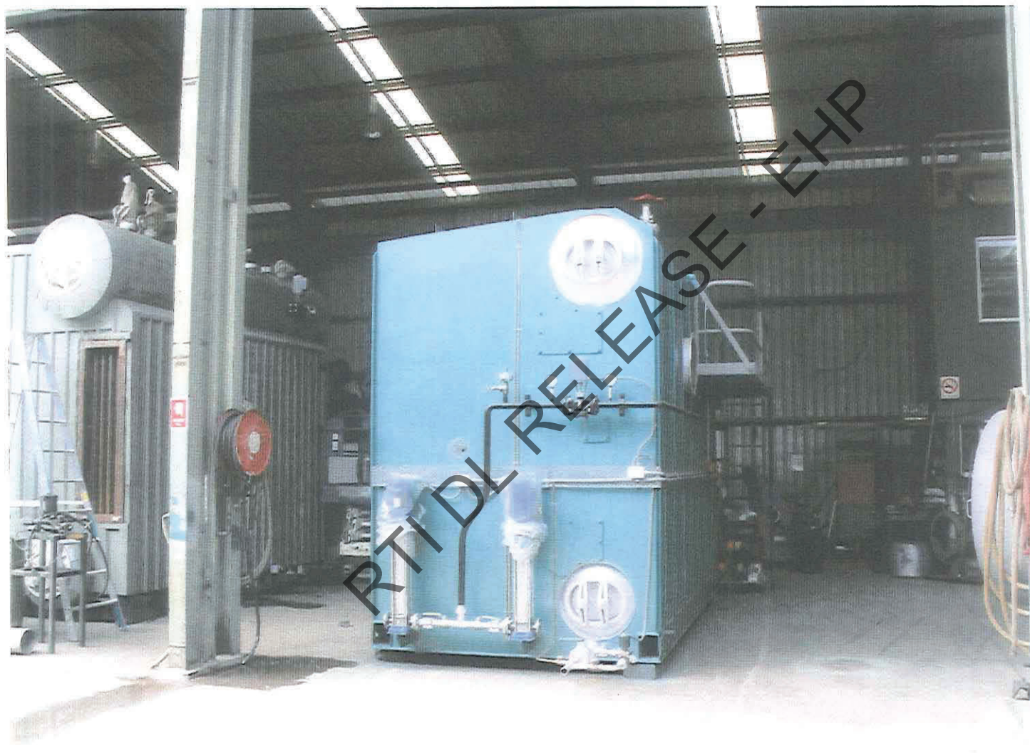
Photograph 12: Boiler Module (view from west)
