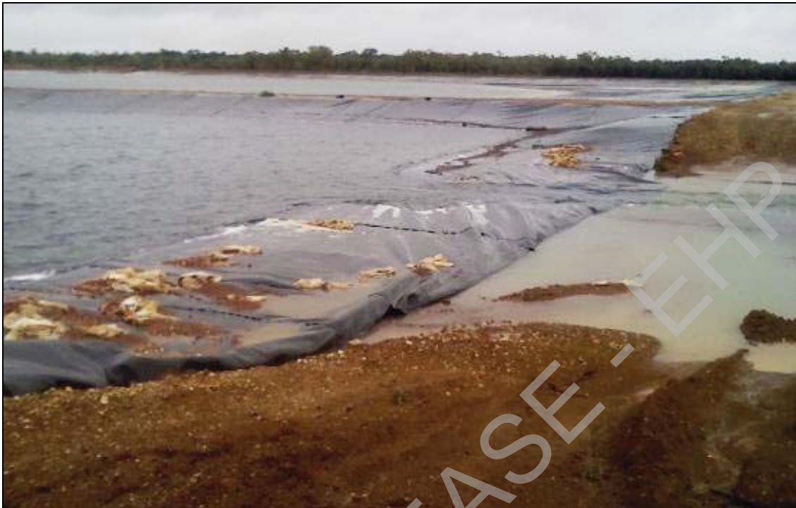
Figure 7: Scour beneath SW Pond#1 Spillway (Taken 0700 on 31JAN09).
