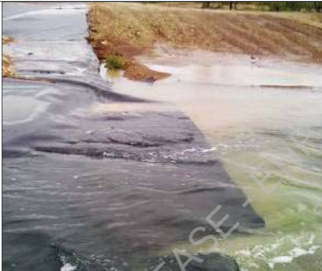
Figure 5: Water flowing over and under pond liner SW Pond #1 Spillway (Taken 0650 on
