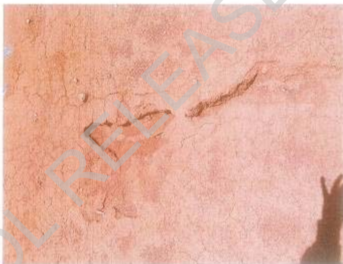
Figure 7: Depression in ground on northern side of Stormwater Pond No. 1
