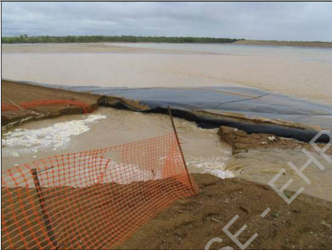
Figure 10: SW Pond #2 at point of wall failure (Taken 1000 on 30JAN09).
