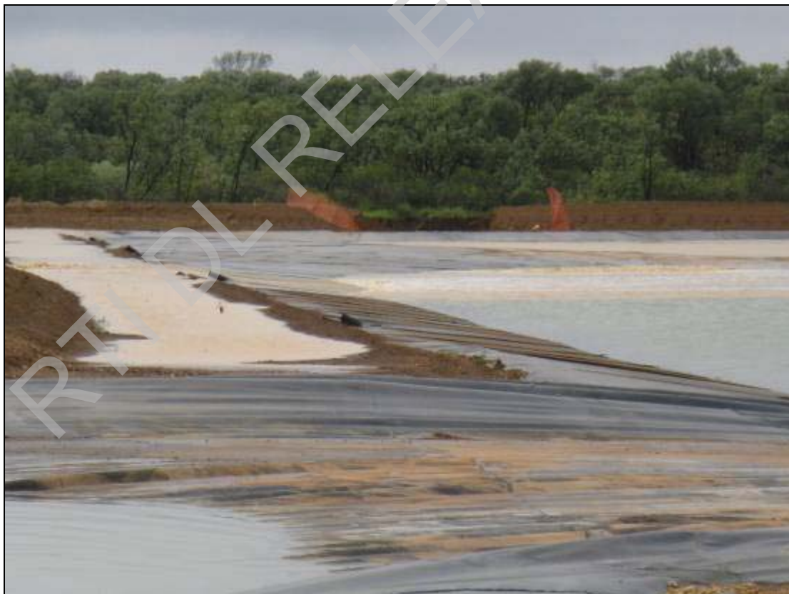
Figure 13: SW Pond #2 looking south towards wall failure (Taken 1000 on 30JAN09).
