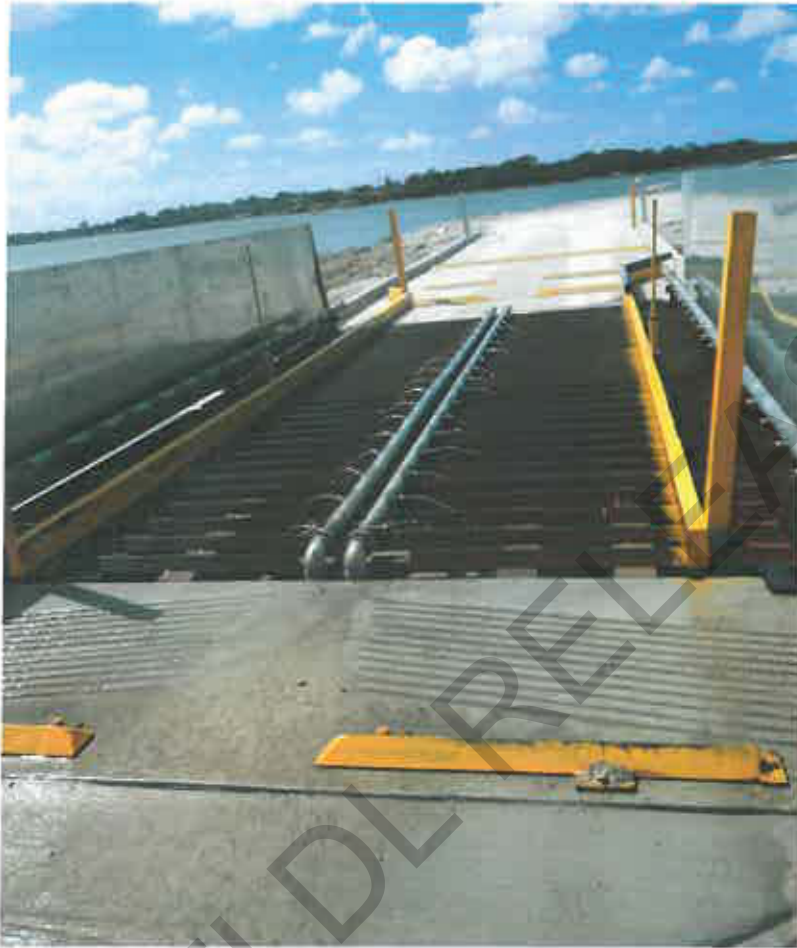
Figure 1 – Wheel Wash installed on site at Exit Point 1 (see map below)
