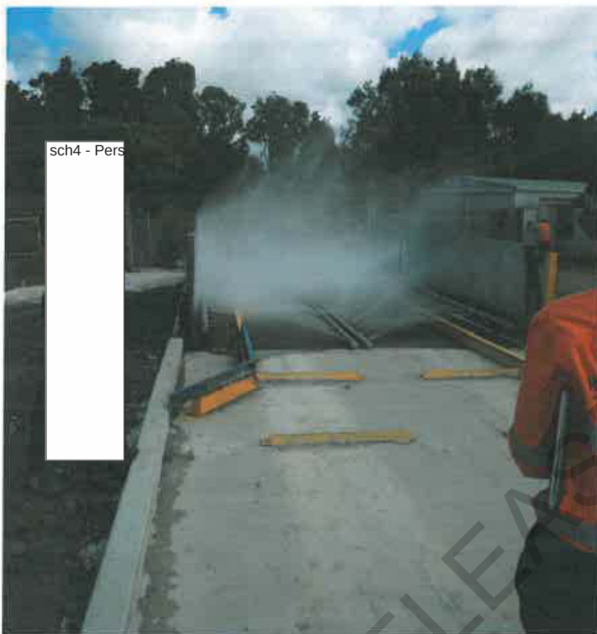
Figure 2 – Wheel Wash with sprays
